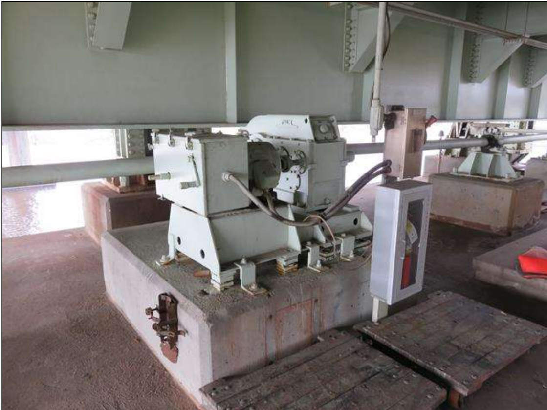
EAST TOWER SPEED REDUCER, MOTOR AND BRAKE.
