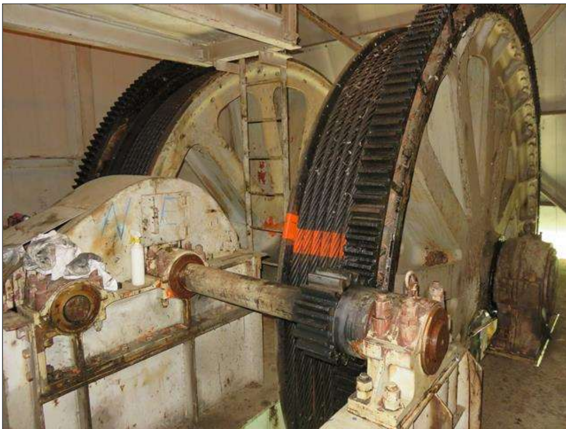
OPERATING MACHINERY NORTH EAST ROOM.
