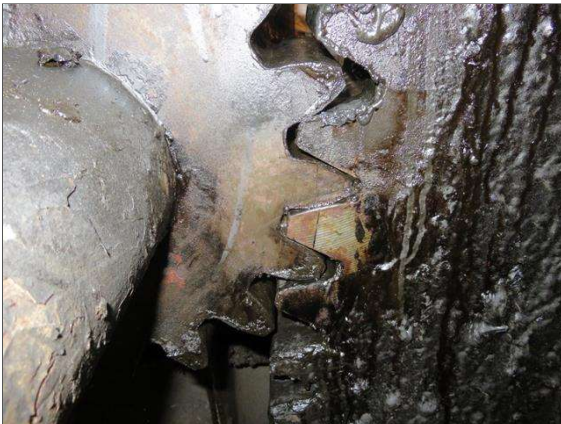
ROOT TO TIP MEASURED .147 FOR GEARS 271-1 & 276 NORTH WEST ROOM (WEST TOWER)
