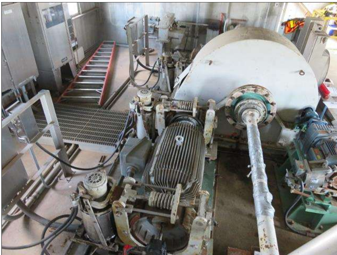
EAST TOWER OPERATING MACHINERY .
