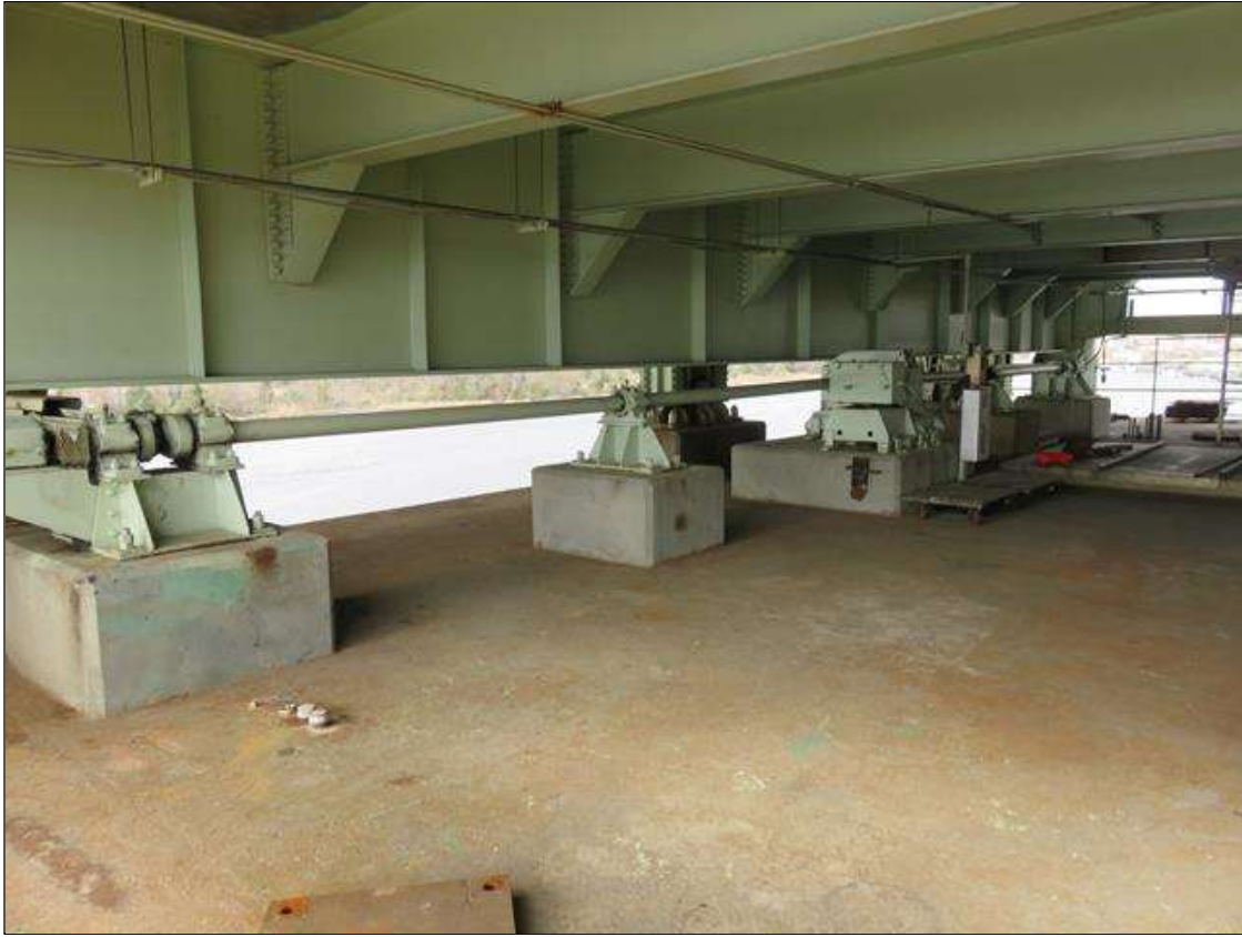
EAST TOWER LOCKING MACHINERY.
