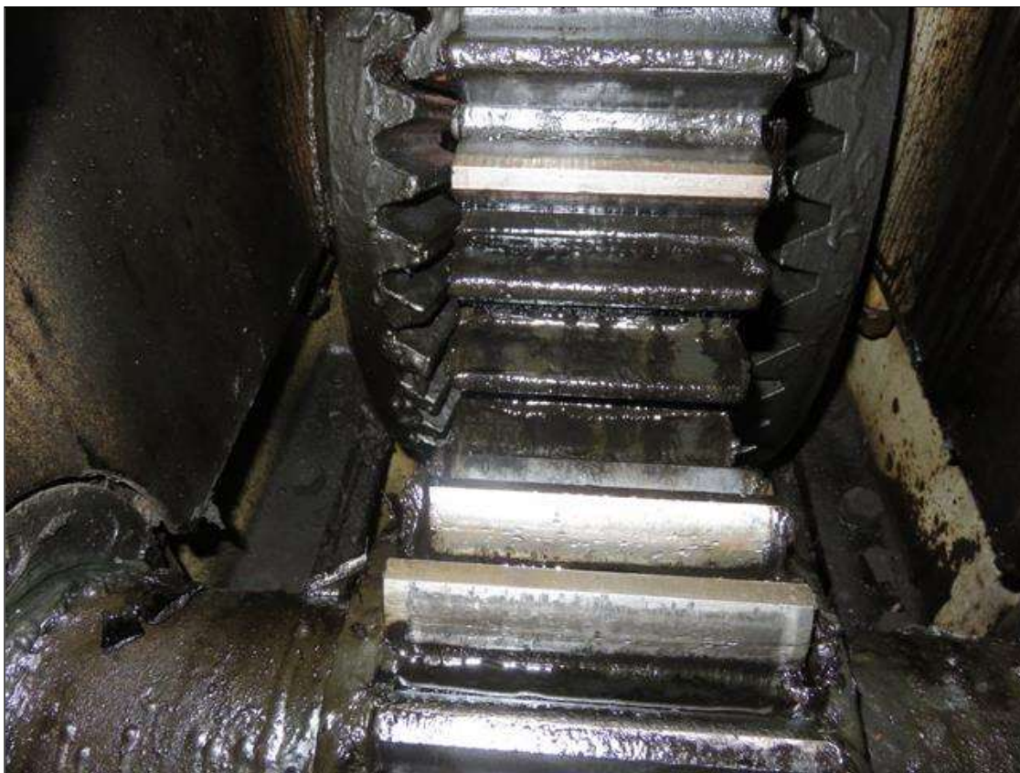
GEARS 278 & 357 NORTH WEST ROOM WEST TOWER.
