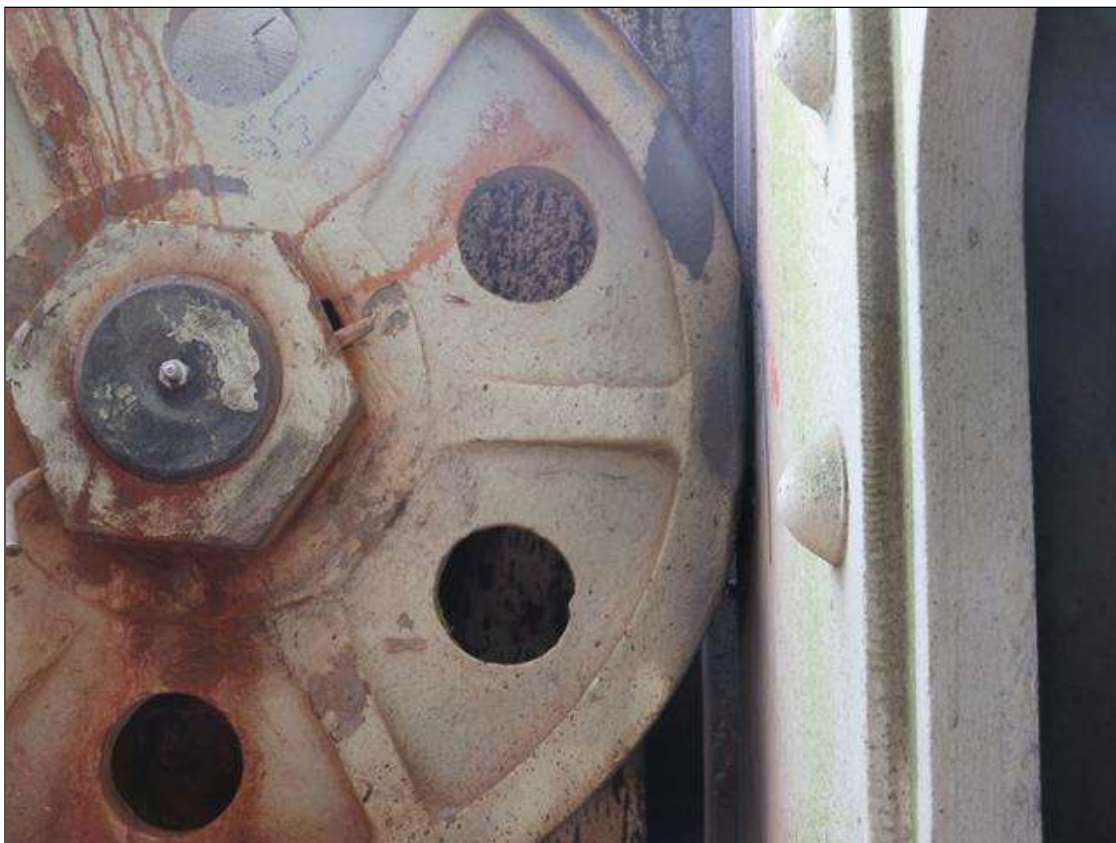
FLAT SPOT WORN ON WHEEL NORTH EAST LOWER TOWER ROLLER #54
