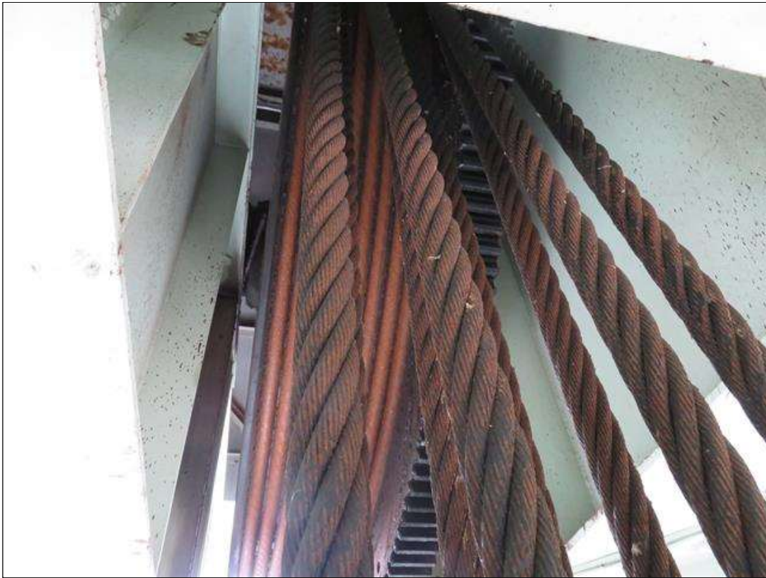
COUNTER WEIGHT CABLES SHOW EARLY STAGES OF SURFACE RUST AND NEED GREASING SOUTH EAST TOWER PICTURED ALL CABLES NEED TO BE GREASED.
