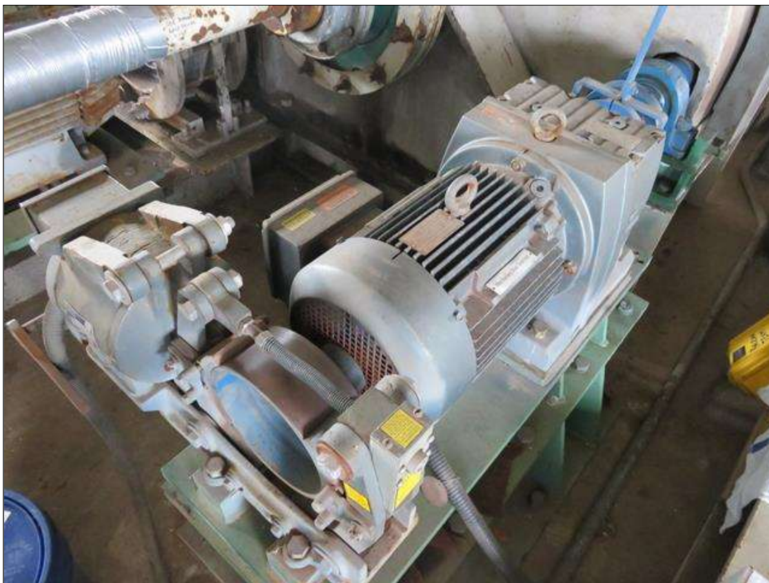
WEST AUXILIARY DRIVE GENERATOR AND BRAKE.
