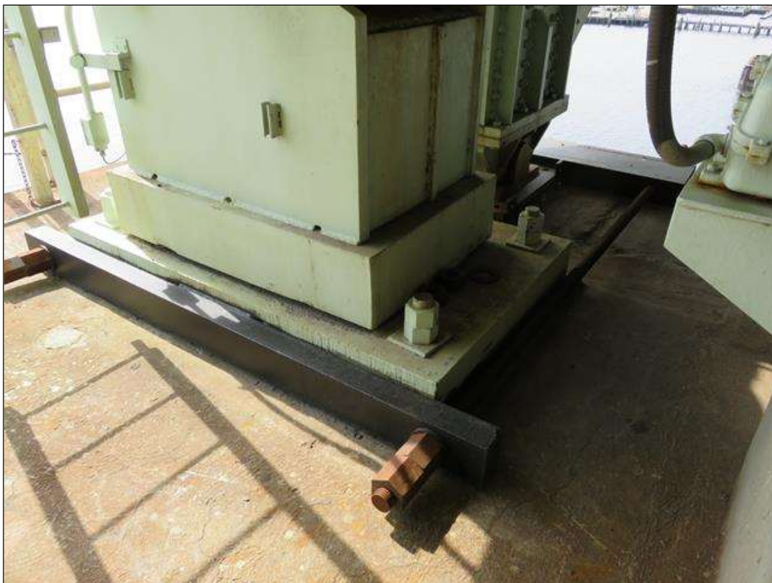
NEW SUPPORT TO SOUTH EAST FIXED BEARING HAS BEEN ADDED (NORTHEAST SIDE SAME) NOTE: STILL HAS VERTICAL MOVEMENT UNDER LIVELOAD.
