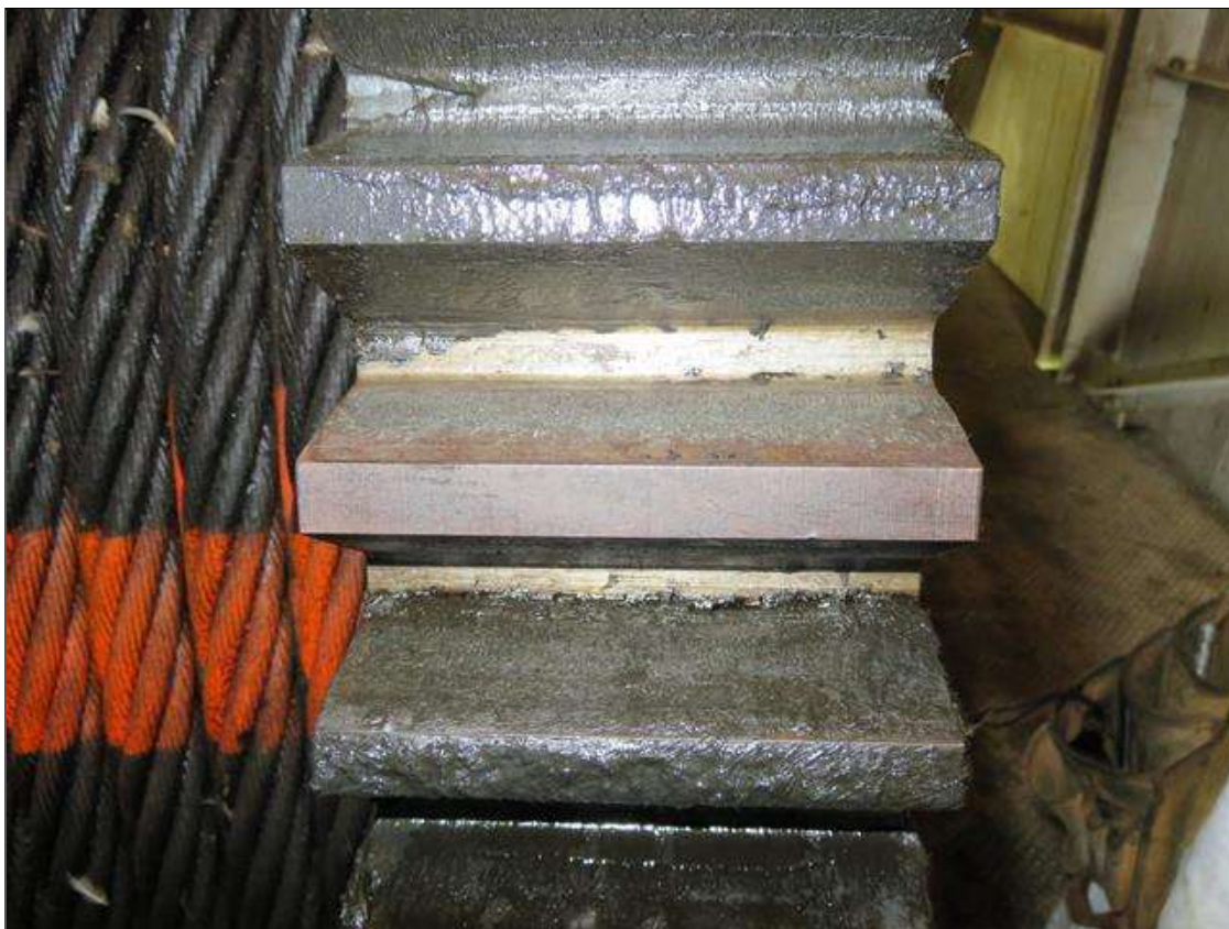
NORTH EAST ROOM GEAR 271-2 HAS MINOR SCORING TO OPEN AND CLOSING SIDE OF TEETH.
