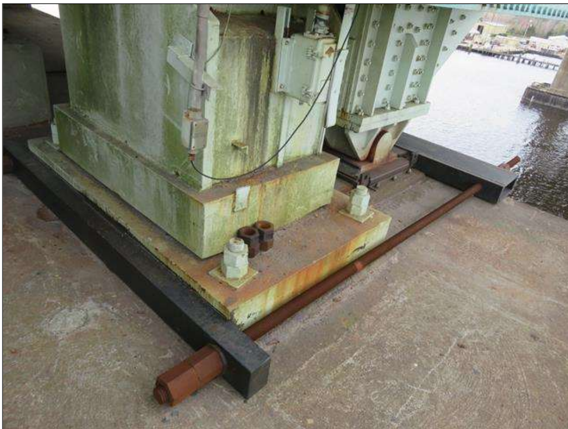
NEW SUPPORT TO NORTH EAST FIXED BEARING HAS BEEN ADDED. (NOTE: STILL HAS VERTICAL MOVEMENT UNDER LIVELOADS)
