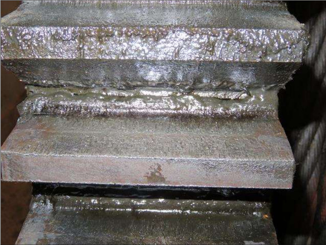
SOCRING & 1/32" GROOVES IN OPEN AND CLOSING SIDE OF 271-1 SOUTH WEST ROOM (WEST TOWER)
