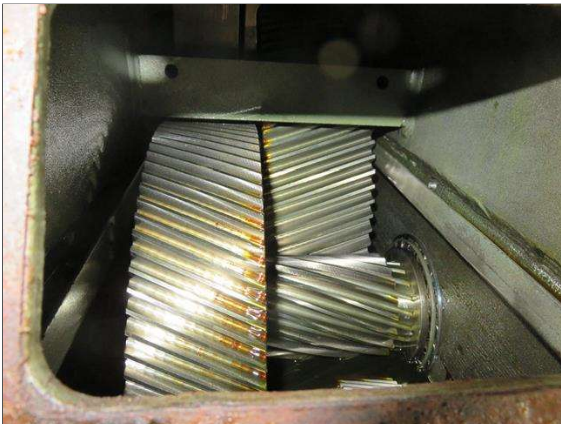
WEST END SPEED REDUCER GEARS GOOD ,FLUID LEVELS GOOD (FLUID SAMPLE TAKEN)
