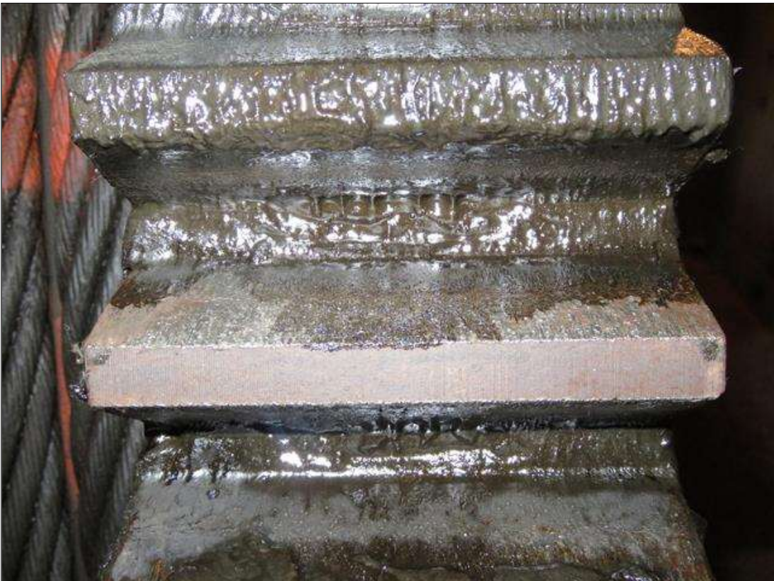
GEAR 271-2 IN WEST TOWER HAS 1/32" GROOVES ON OPEN AND CLOSING SIDE OF TOOTH (NORTH WEST ROOM)
