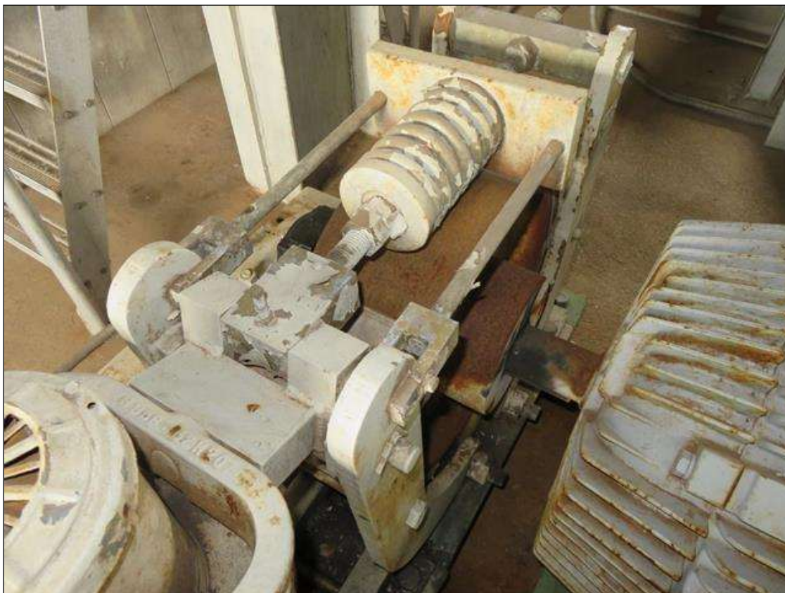
BRAKE #3 OPERATING MACHINERY WEST TOWER HA 1/32" SURFACE RUST TO DRUM.
