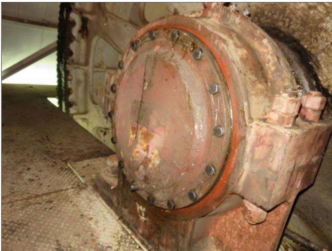
NORTH EAST ROOM SOUTH SIDE OUTSIDE TRUNNION REASSEMBLED AFTER TEAR DOWN AND UT INSPECTION.
