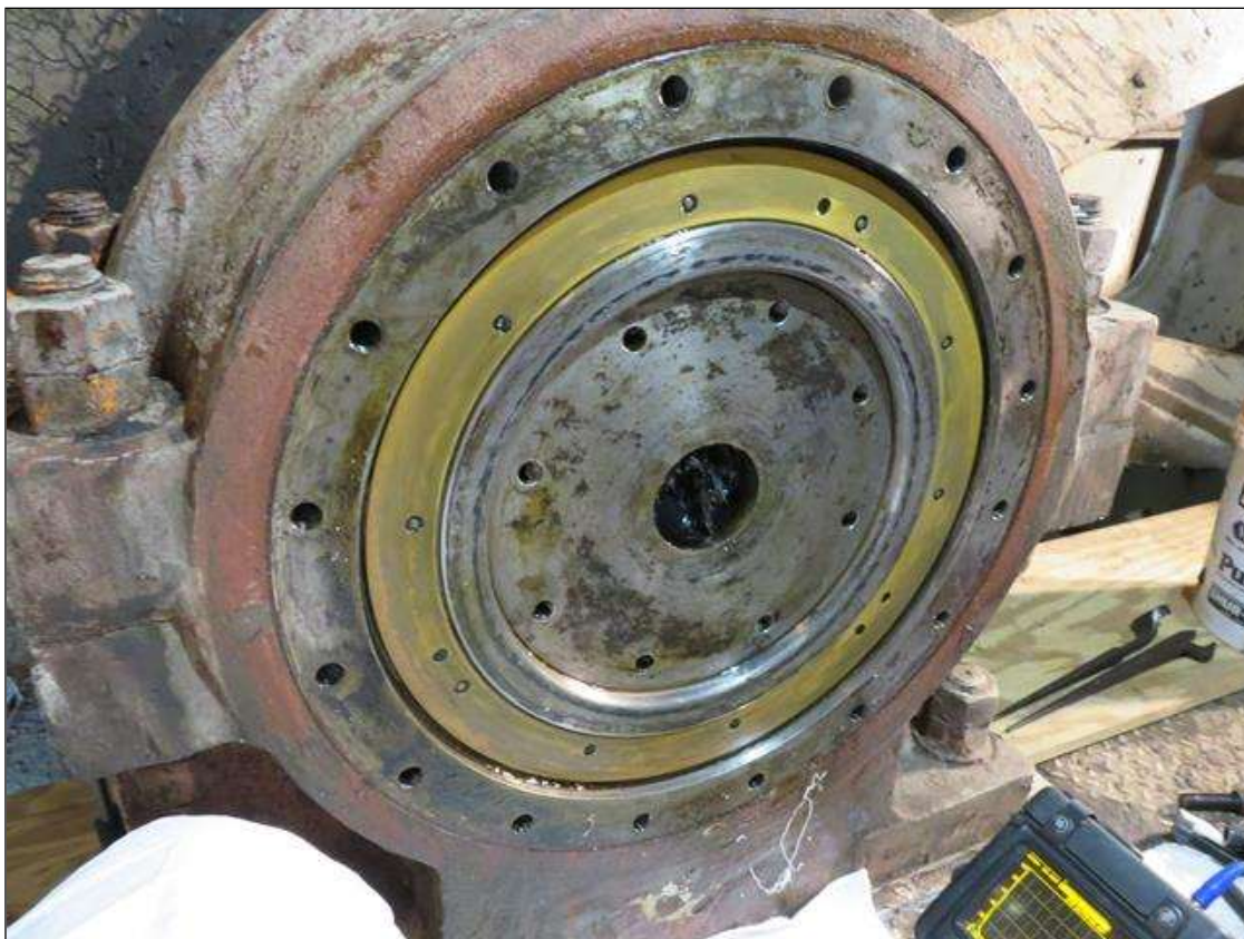
NORTH EAST ROOM SOUTH OUTSIDE TRUNNION WITH INNER PLATE REMOVED FOR TESTING.
