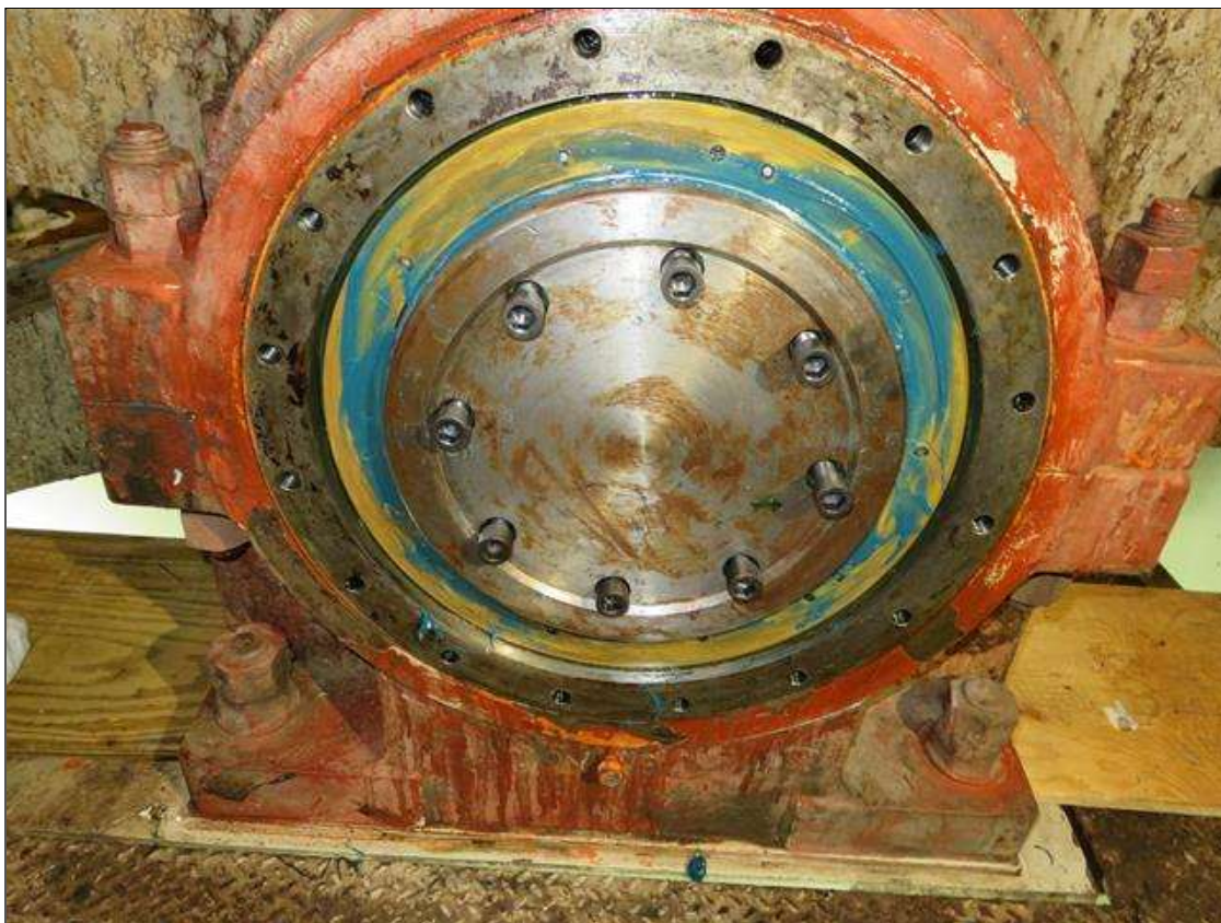
SOUTH EAST ROOM, SOUTH OUTSIDE TRUNNION BEING REASSEMBLED AND LUBED AFTER BEING TESTED WITH ULTRA SONICS MACHINE.
