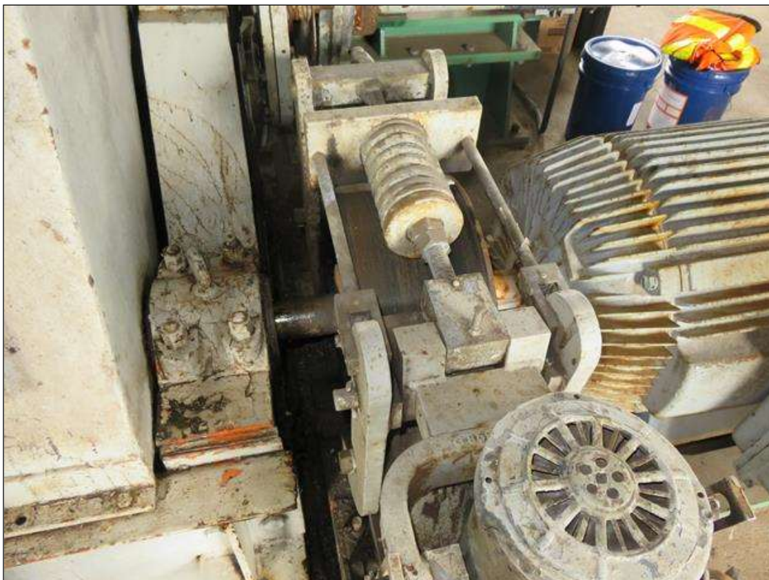
BRAKE #1 OPERATING MACHINE WEST TOWER. (FLUID LEVEL GOOD BUT DIRTY)
