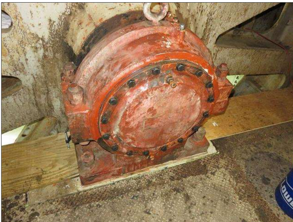
SOUTH EAST ROOM SOUTH SIDE OUTSIDE TRUNNION REASSEMBLED AFTER TEAR DOWN AND UT INSPECTION.
