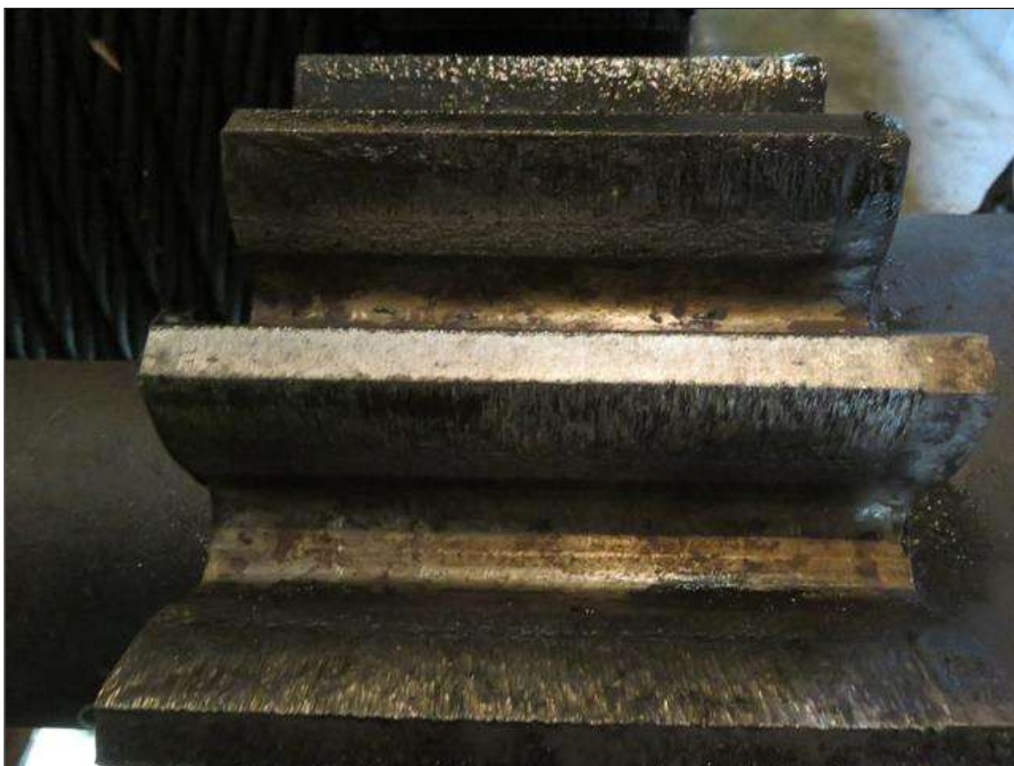
NORTH EAST ROOM GEAR 276 HAS 1/32" GROOVES ON OPEN AND CLOSING SIDE OF TEETH.
