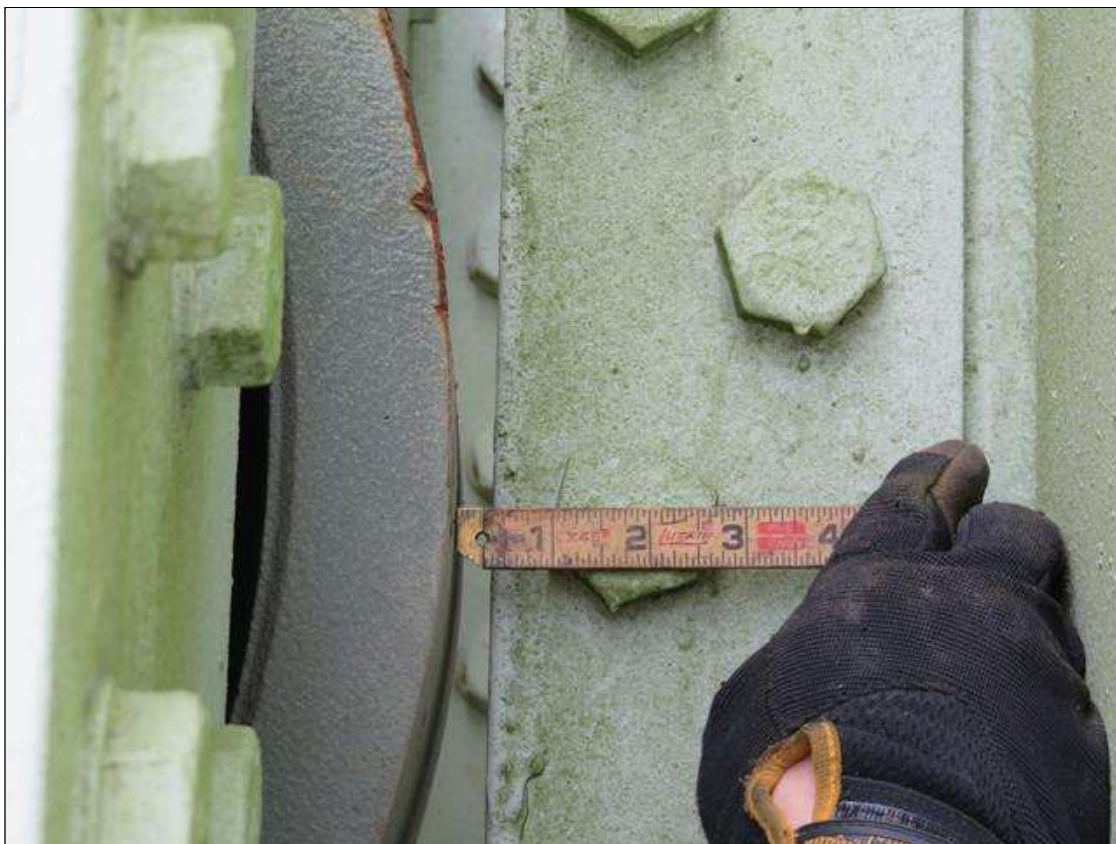
GUIDE ROLLER HAS 3/8" GAP NORTH WEST SIDE
