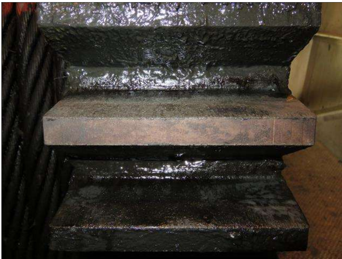
GEAR 271-1 IS IN FAIR CONDITION (MINOR GROOVES ON OPEN AND CLOSING SIDE OF TEETH. (SOUTH WEST ROOM WEST TOWER)
