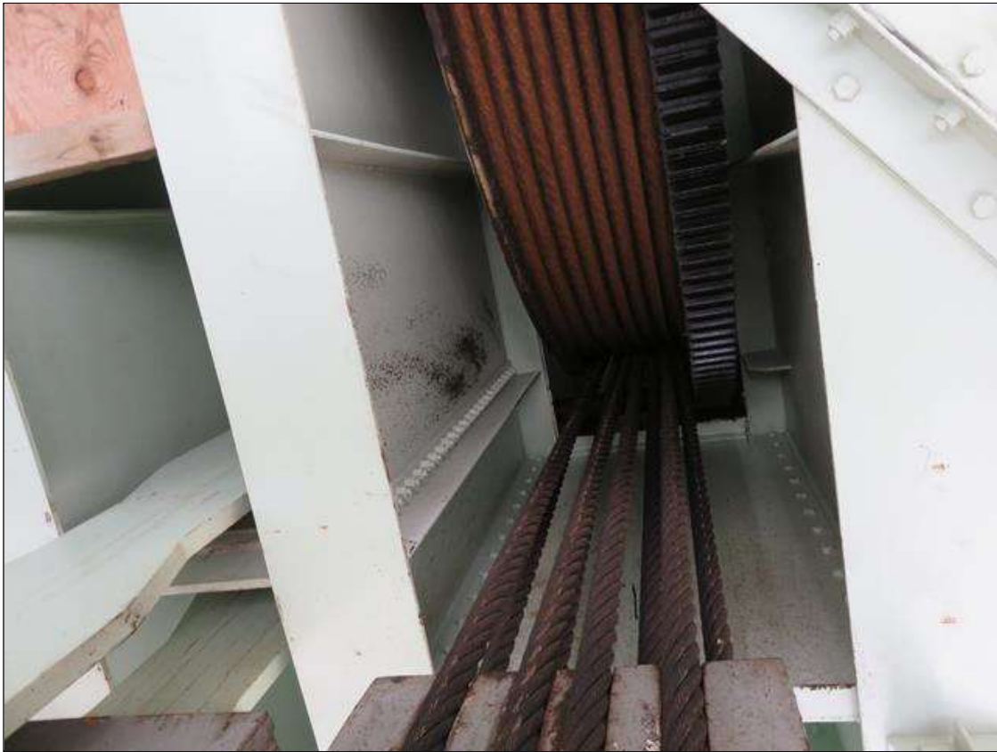
LOOKING UP AT CABLES AND GEARS (EAST TOWER)
