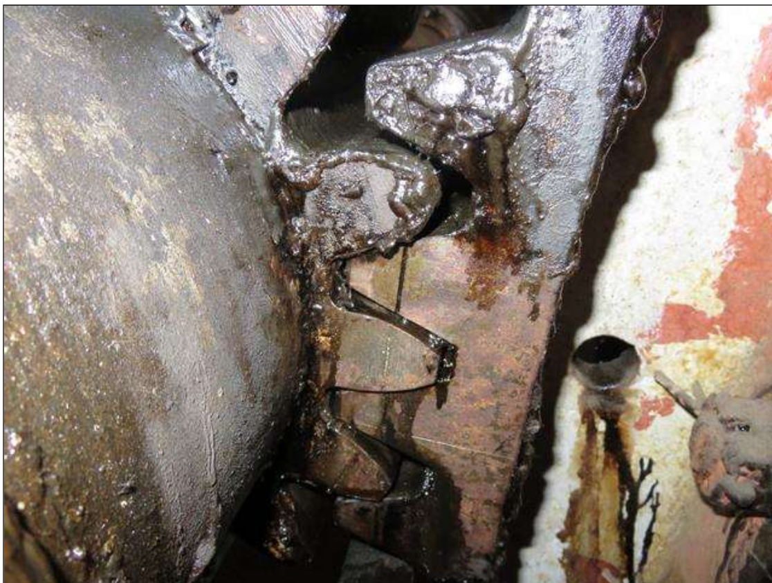
ROOT TO TIP MEASURED .180 FOR GEARS 271-2 & 277 NORTH WEST ROOM (WEST TOWER)
