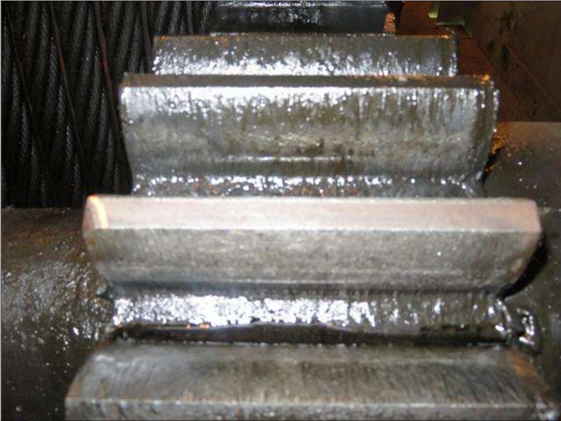
GEAR #277 IN WEST TOWER HAS 1/32" GROOVES ON OPEN AND CLOSING SIDE OF TOOTH & 1/16" CHIP TO LEFT CORNER OF TOOTH. (NORTH WEST ROOM)
