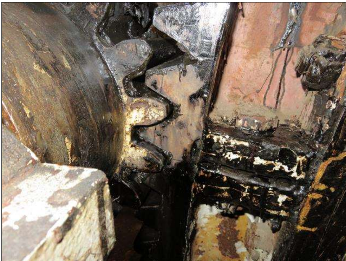
BACKLASH OF .099 WAS MEASURED FOR #271-2 & 278 GEARS IN NORTH EAST ROOM.
