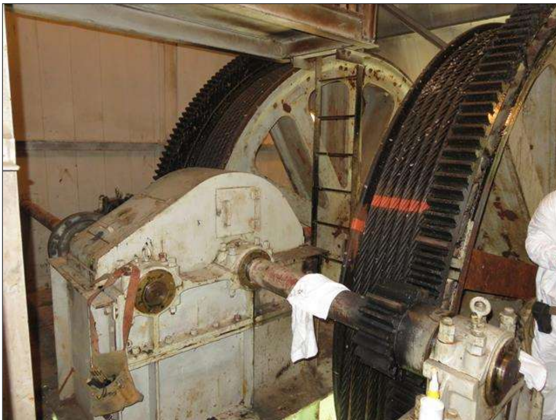
WEST TOWER OPERATING MACHINERY SOUTH SIDE.
