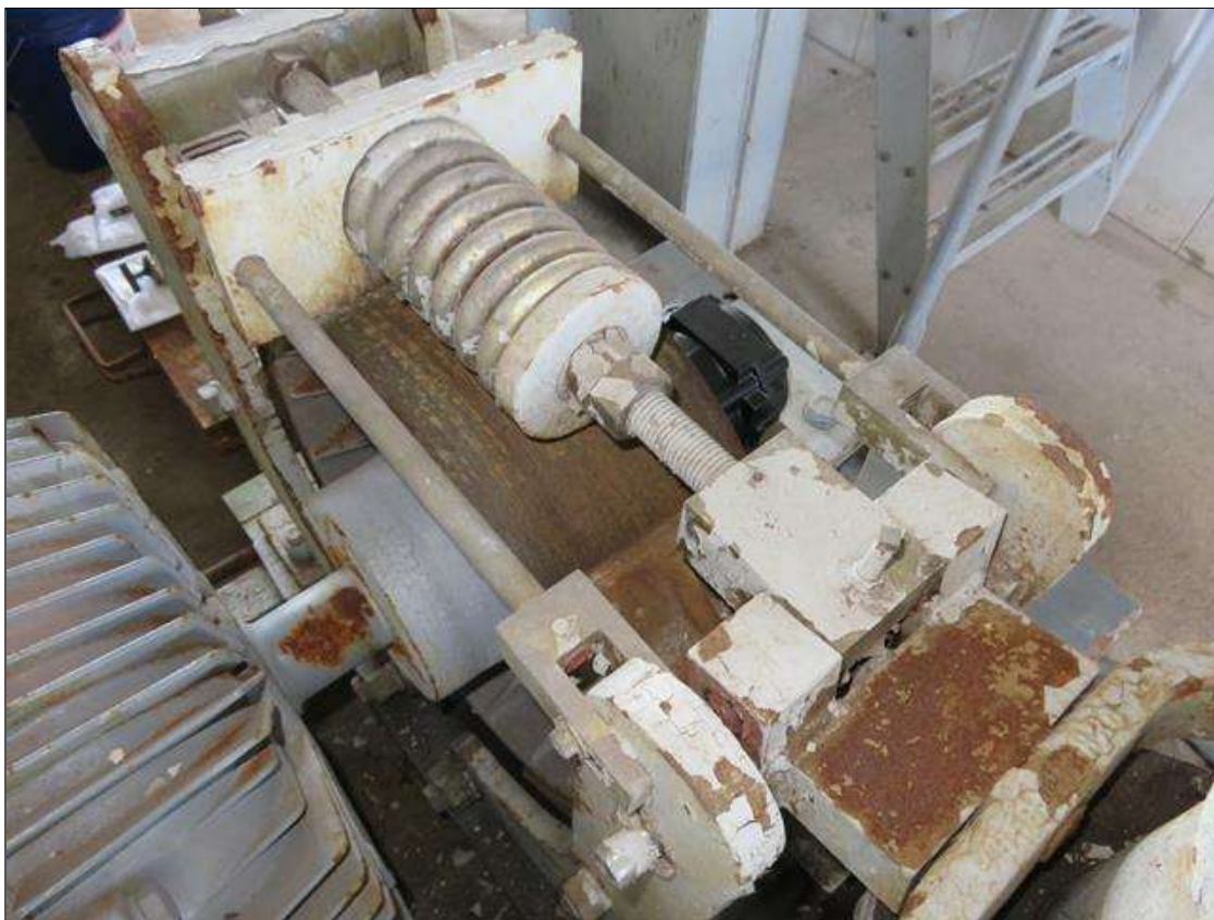
BRAKE #1 EAST OPERATING MACHINERY HAS 1/32" SURFACE RUST ON DRUM (PADS GOOD)
