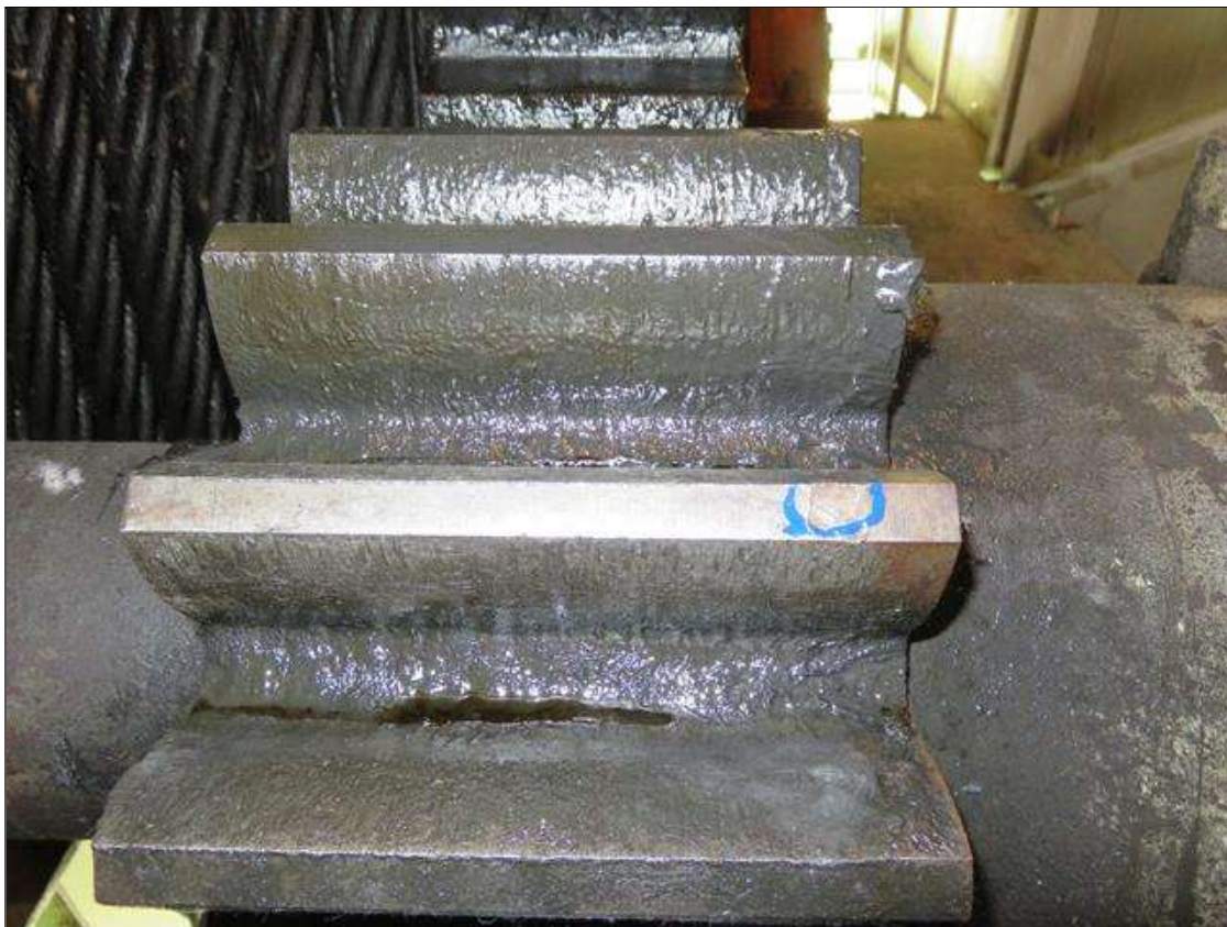
GEAR 277 TOOTH HAS SMALL 1/8" GOUGE IN TOP RIGHT SIDE OF TOOTH SOUTH WEST ROOM (WEST TOWER)
