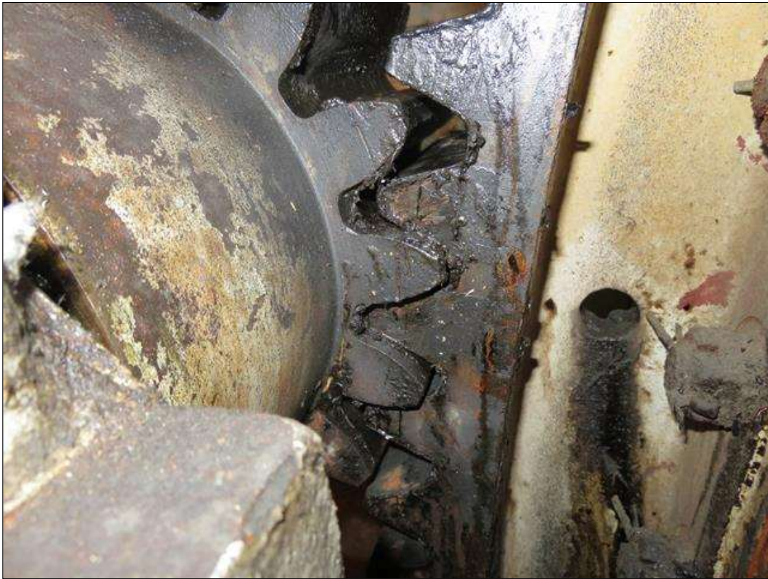
ROOT TO TIP WAS MEASURED .250 FOR GEARS 271-2 & 277 IN SOUTH WEST ROOM (WEST TOWER)
