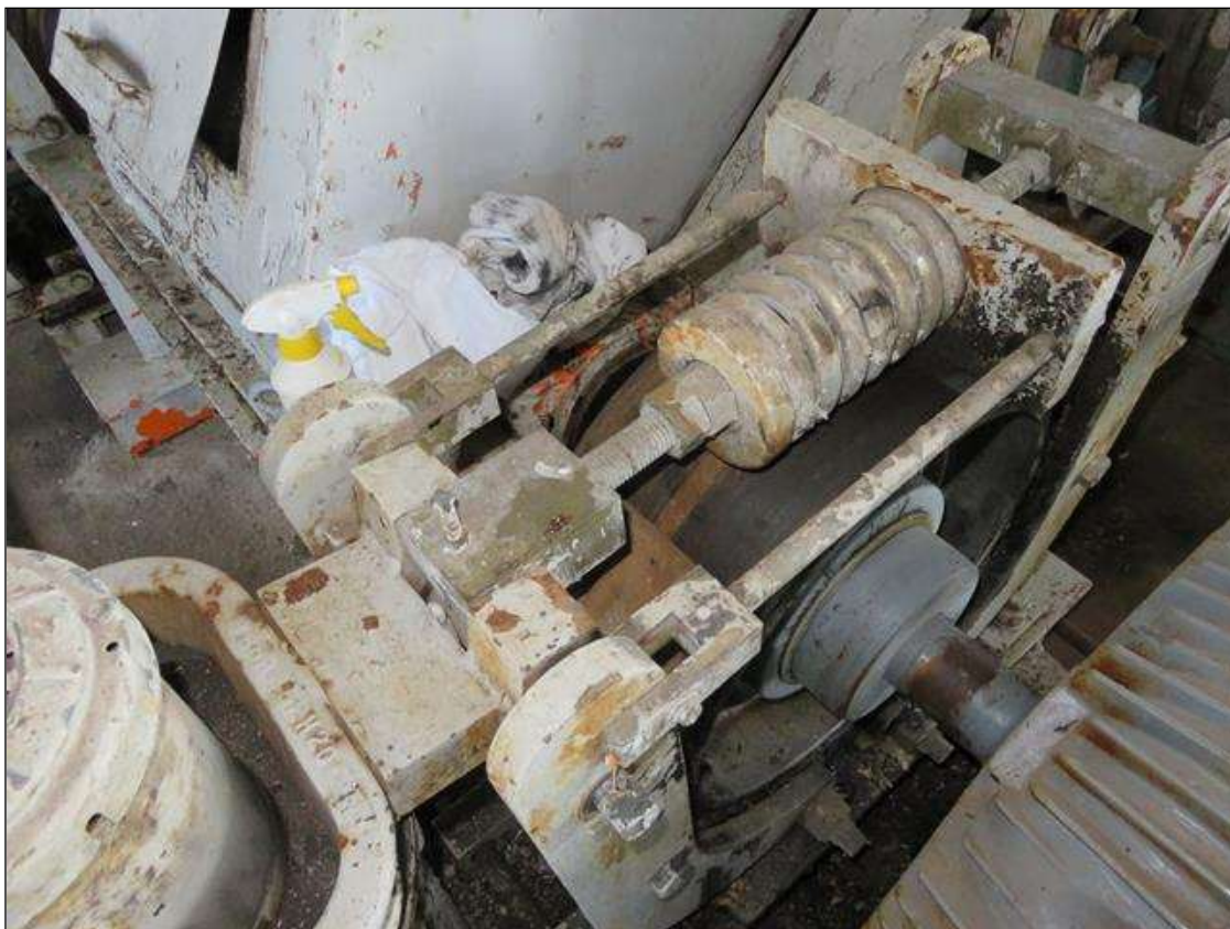
BRAKE #2 EAST OPERATING MACHINERY DRUM AND PADS GOOD. (FLUID LEVEL GOOD BUT DIRTY)
