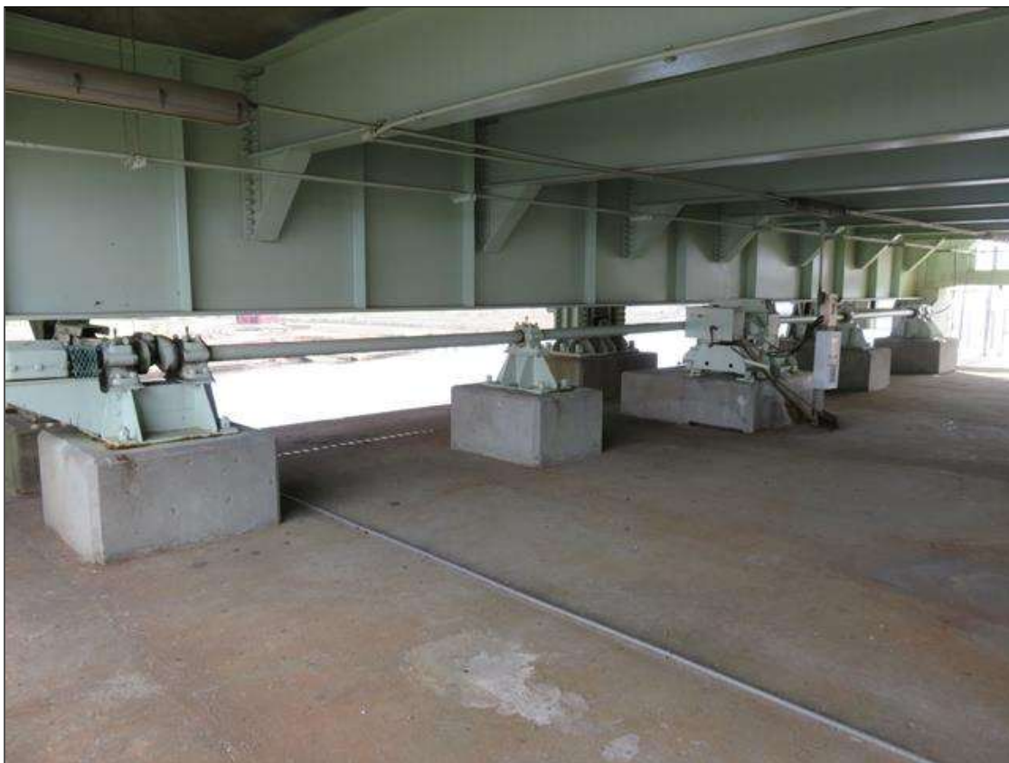
WEST TOWER LOCKING MACHINERY.
