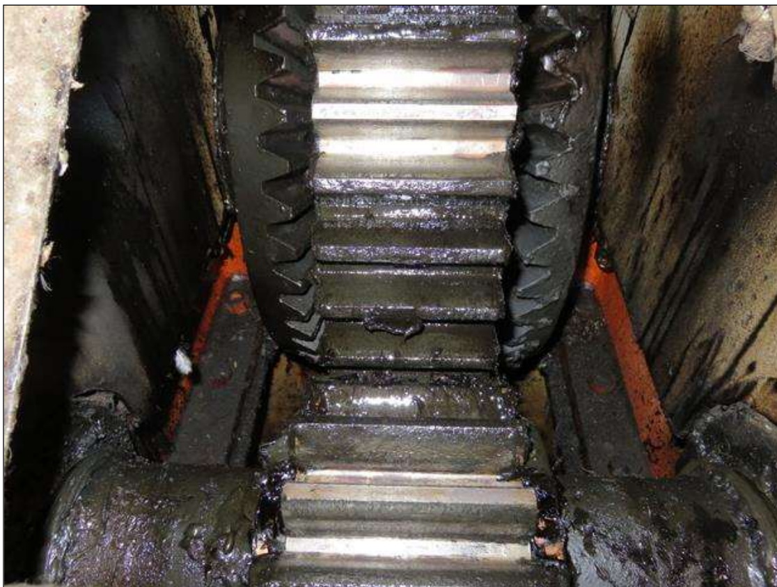
GEARS 278 & 357 IN NORTH EAST ROOM.
