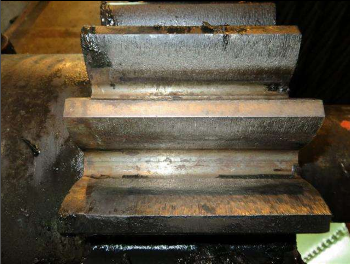
SOUTH EAST ROOM GEAR # 276 HAS 1/32" GROOVES ON OPEN AND CLOSING SIDE FACE OF TOOTH. (ALL SHOW THIS CONDITION #277 IN SOUTH EAST ROOM ALSO.)
