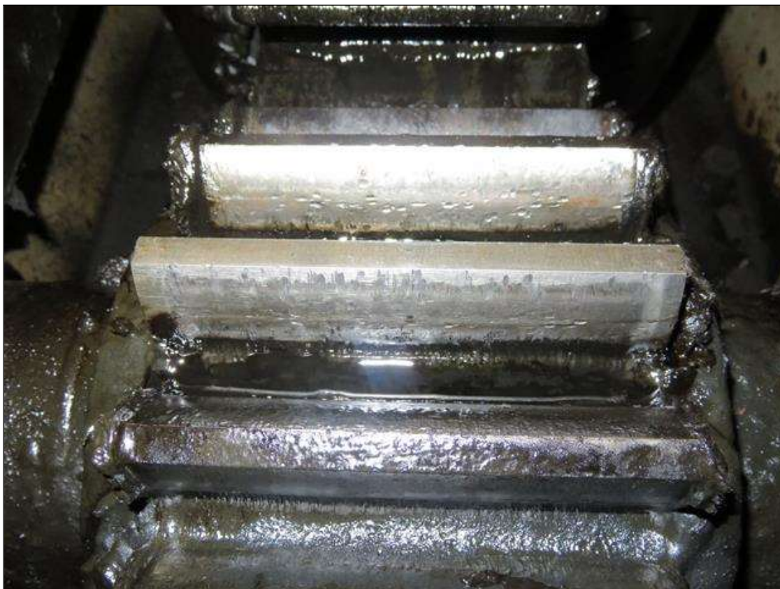
GEARS 278 HAVE SEVERAL SMALL 1/8" KNICKS AND GOUGES ON FACE OF TEETH NORTH WEST ROOM.
