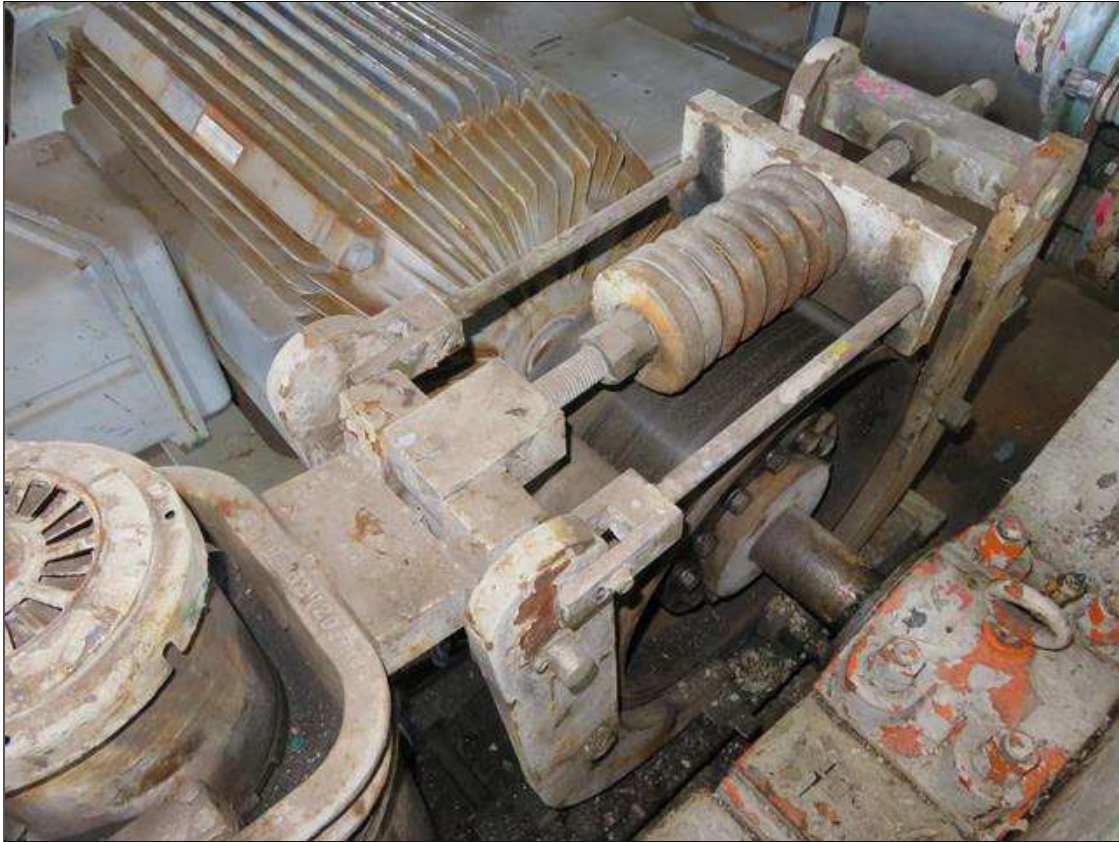
BRAKE #3 EAST OPERATING MACHINERY DRUM AND PADS GOOD.
