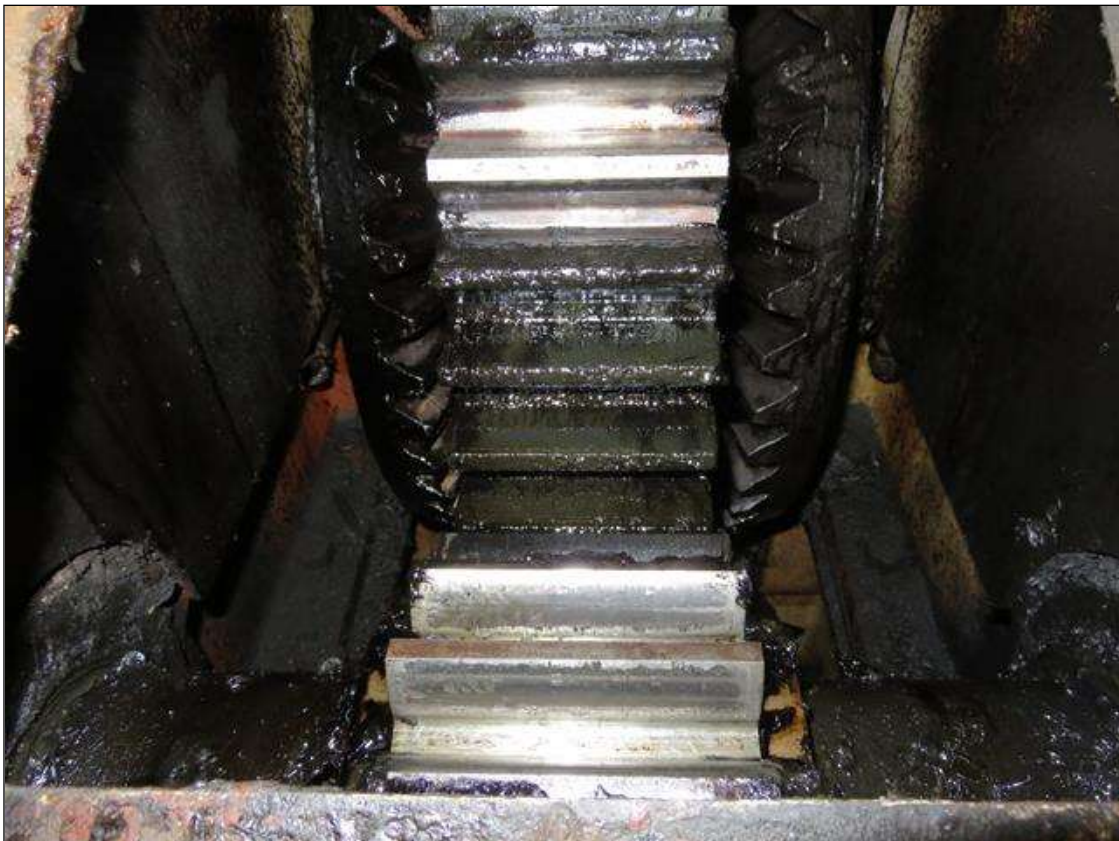
GEARS 278 & 357 SOUTH EAST ROOM.
