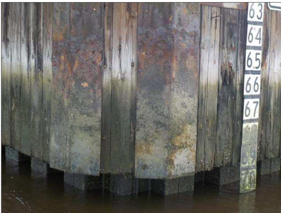
BENT 17, RUST ON COVER PLATES
