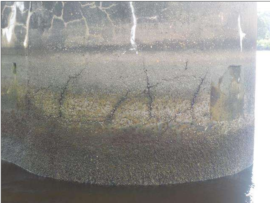
BENT 15, HORZ. /VERTICAL CRACKING TO 1/8" FULL LENGTH TZ
