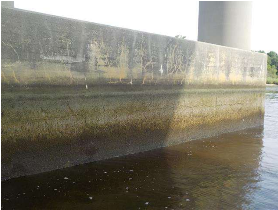
BENT 14, HORZ. CRACK 1/8", WITH VERTICAL CRACK 1/16" FULL LENGTH TZ
