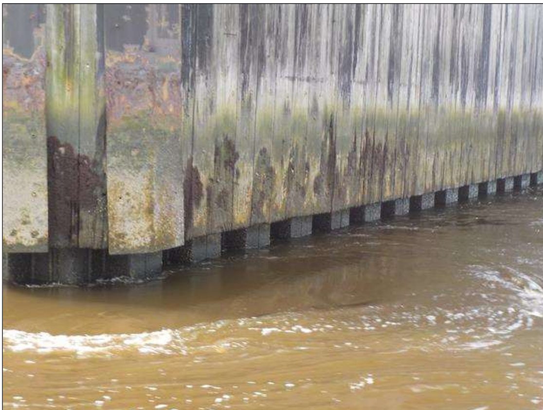
DECAYING TIMBERS BENT 17- VERTICALS
