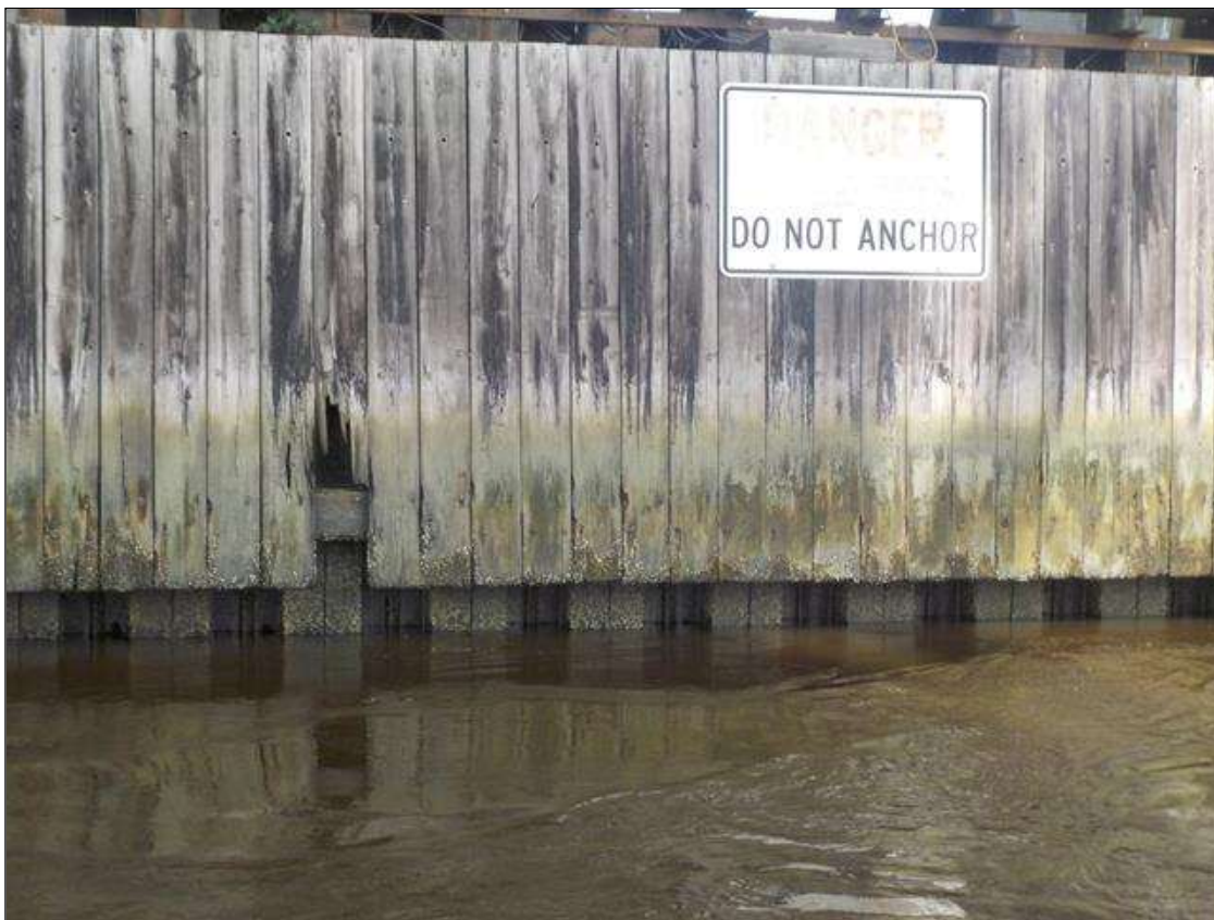
BENT 16, DECAY ON TIMBER- VERTICALS
