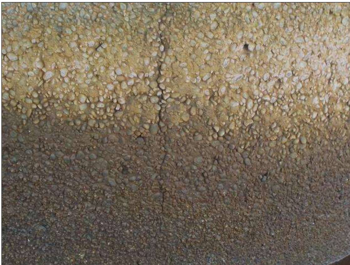
BENT 13, C-2, CRACK-1/16" SPALLED TO 1/8", EAST FACE. NORTH AND SOUTH SIMILAR-3 CRACKS.
