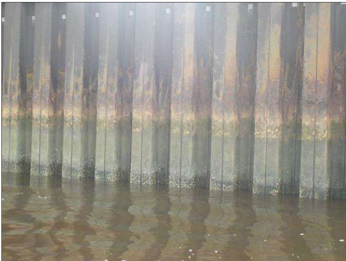
BENT 16, RUST BLISTERS ON SHEET PILE
