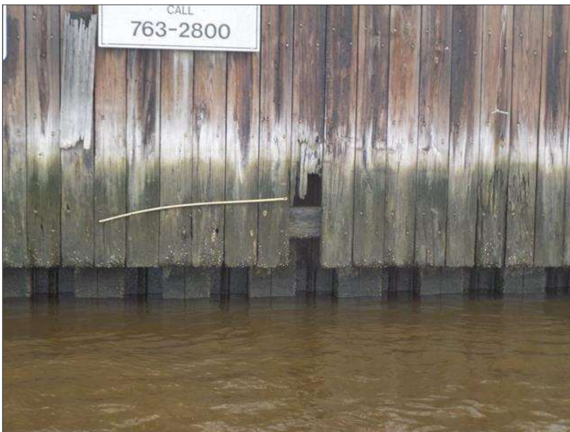
BENT 17 DECAY ON TIMBER- VERTICAL
