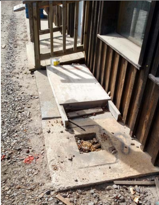
Concrete pad showing outline of former gasoline dispenser and product line (in hole).
