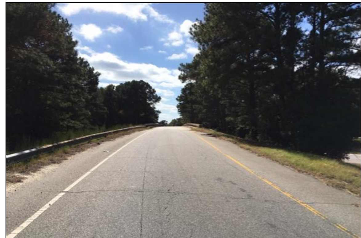
PHOTOGRAPH NO. 4: EAST APPROACH TO END BENT NO.2 ON -L- ALIGNMENT, LOOKING WEST
