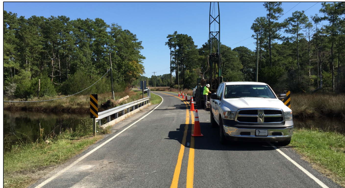
LOOKING UPSTATION ALONG -L-. DRILL RIG SETUP ON B1-B. EB1-A COMPLETED AND VISIBLE FOREGROUND LEFT.
