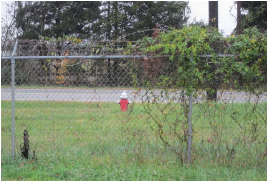
Water and sewer located along W. Center Street in Study Area
