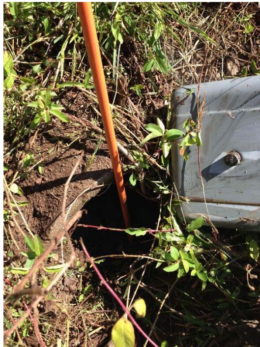
South end of reinforced concrete pipe in Study Area (near the southwest corner of the site)
