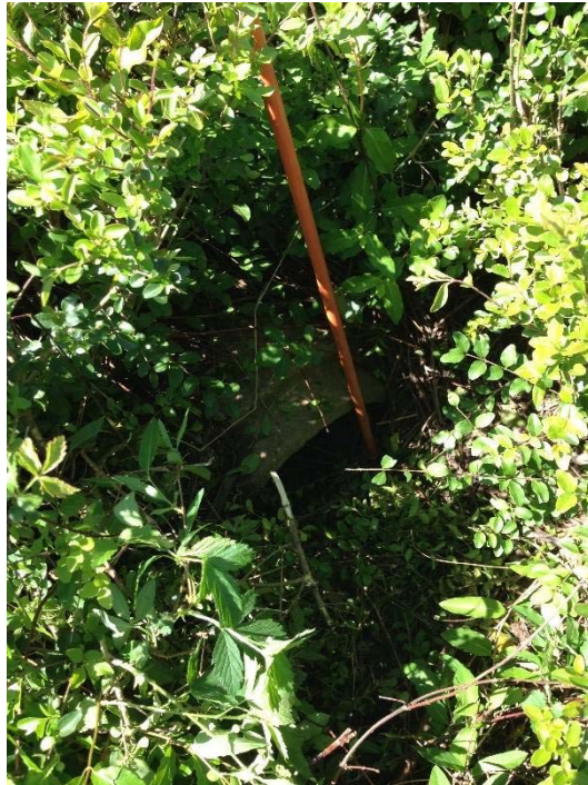
North end of reinforced concrete pipe in Study Area (near the southwest corner of the site)
