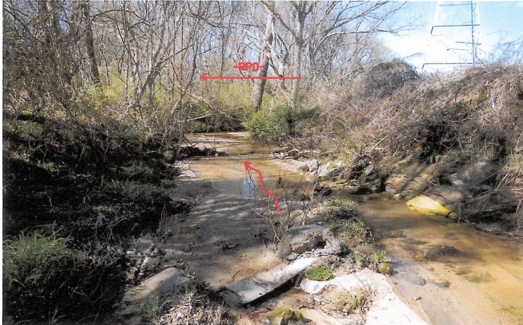
View Facing North (Downstream) Along Tributary L-8 at Proposed -RPD- Culvert Location (Photo taken from BSR)
