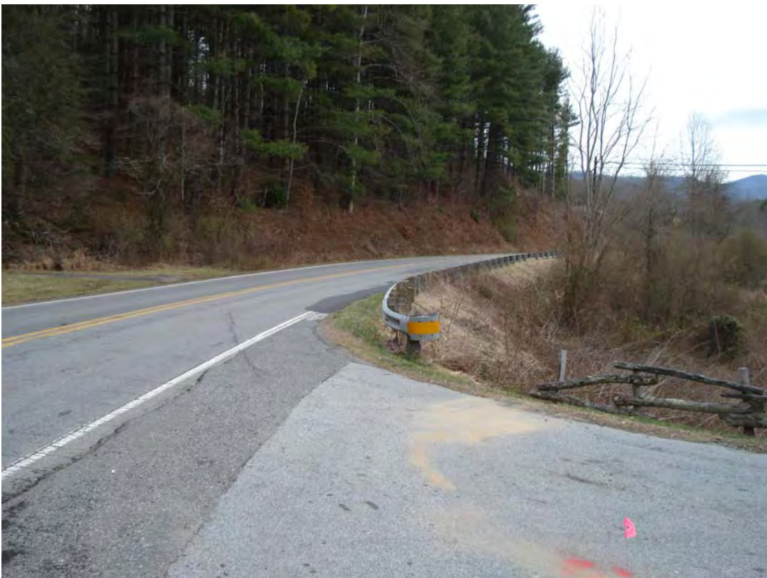
Photograph 2: View looking south at frontage for Parcel 053 extending beyond pavement that was not included in the subsurface investigation due to inaccessibility and no indication of previous development.
