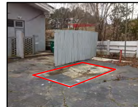
Location of Probable UST (Approximately 2.5-3.0' bls)
