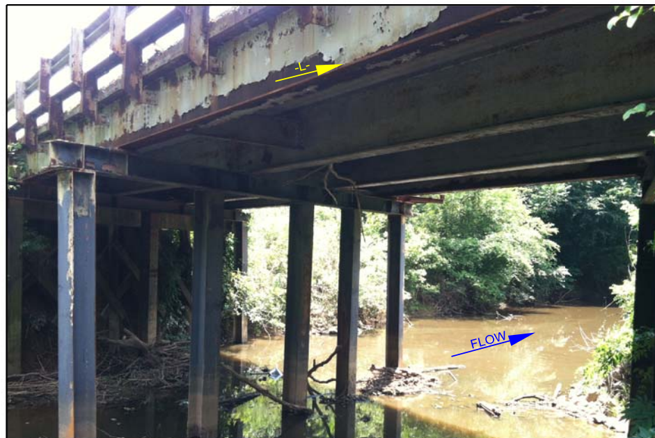
PHOTOGRAPH TAKEN FROM EAST OF END BENT 2 LOOKING LEFT AND SHOWING EXISTING INTERIOR BENTS
