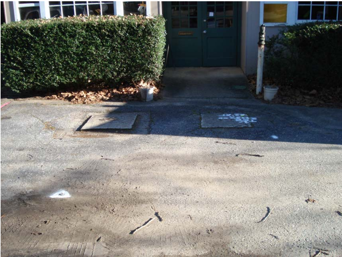
Photograph 7 : View looking southeast at covers for two abandoned septic tanks located at front entrance to onsite real estate office.
