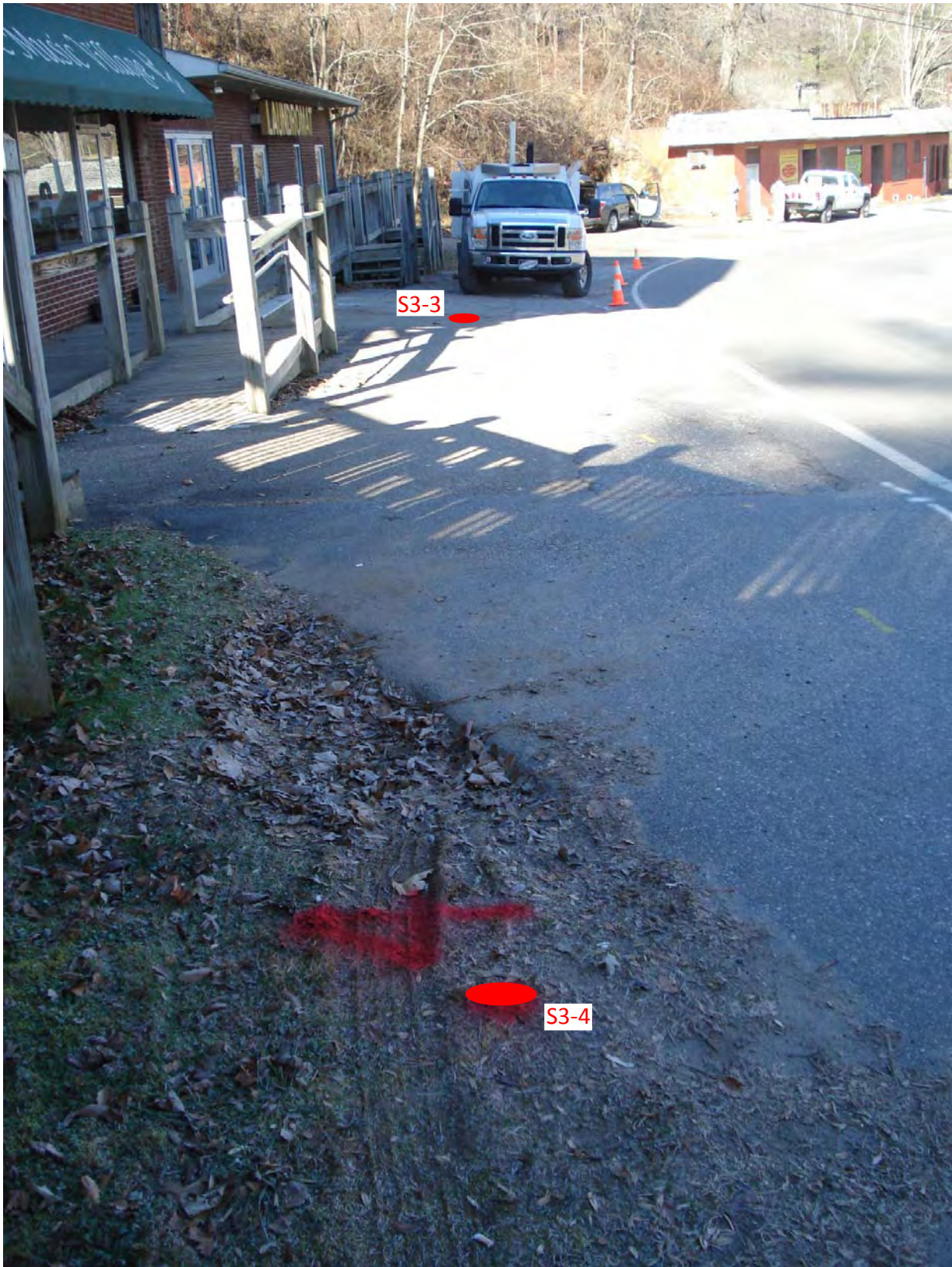
Photograph 3 : View looking northwest at soil boring locations S3-3 and S3-4 at Parcel 003. Aztec Drive is shown on right, and Parcel 005 is shown in the background.
