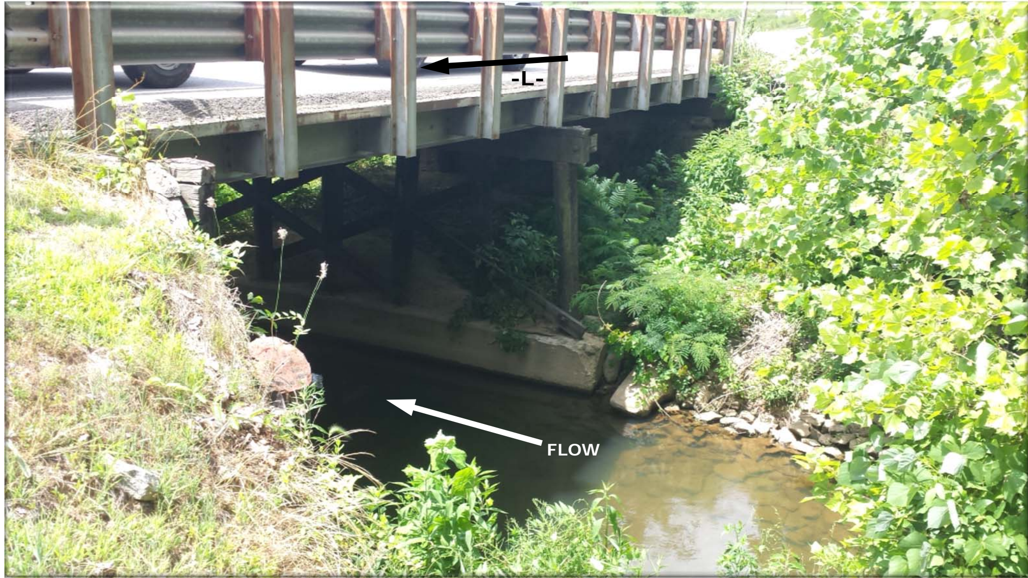
PHOTOGRAPH 1: BRIDGE 169 ON SR 1148 (-L-) OVER GUM CREEK (LOOKING WEST FROM NORTH SIDE).
