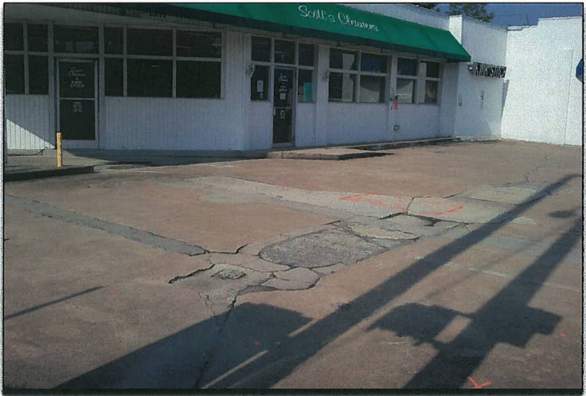
From Northeast property corner looking west-southwest across front of Scott's Cleaners and Former Amoco. Note obvious former dispenser locations in center of picture and former bay doors (3) on front of building converted to windows.
