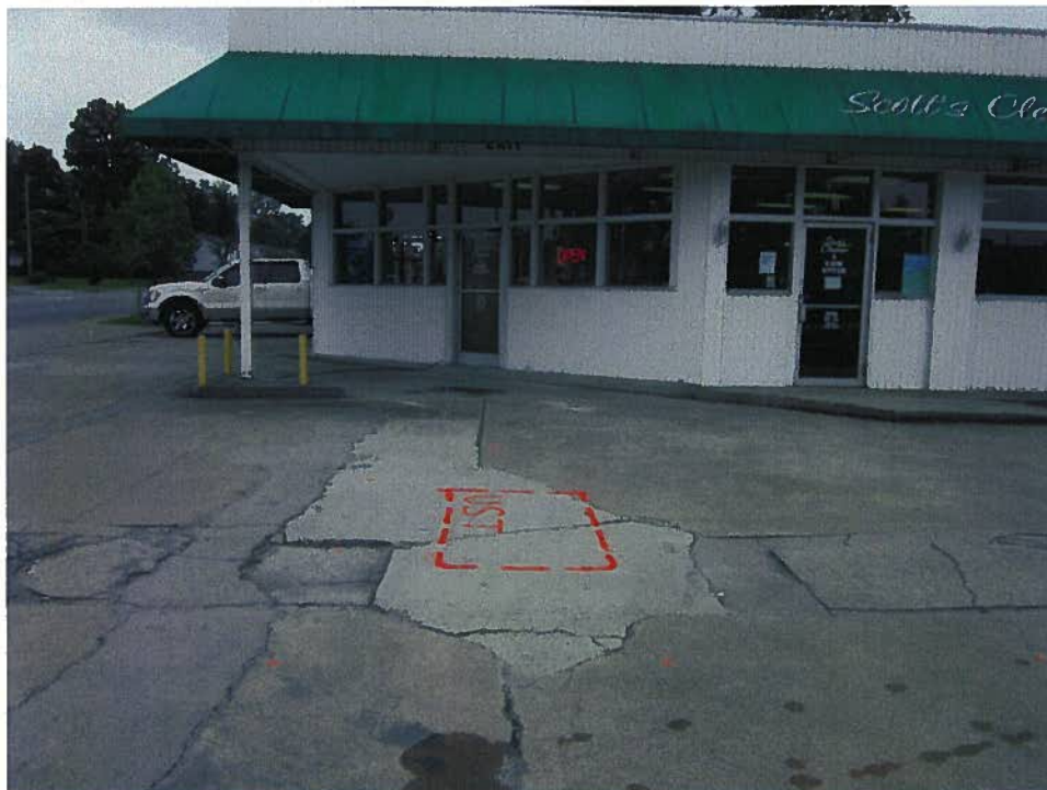
Parcel 105 (Vincent Peele Property LLC), looking south. Photo shows approximate marked location of probable UST No. 1 near the northeast corner of the parcel.
