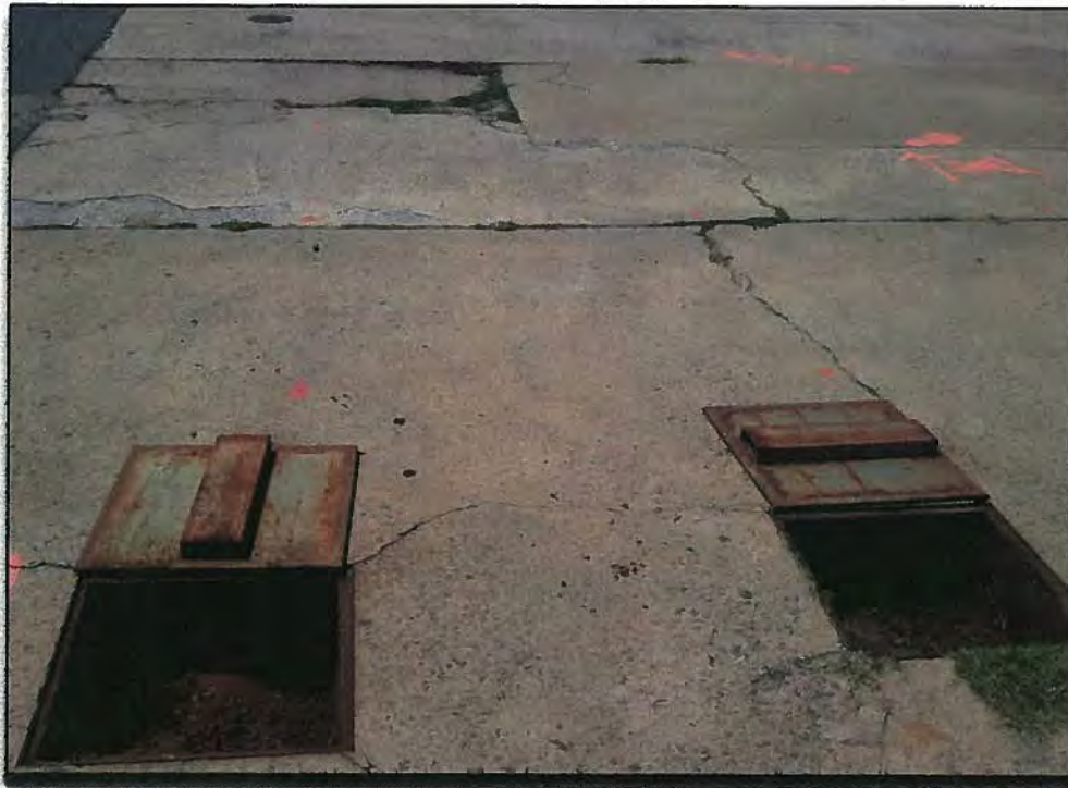
From near northern edge of concrete pad looking South, former UST access vaults filled with concrete in foreground, Eastern UST access manhole visible in background on the left.
