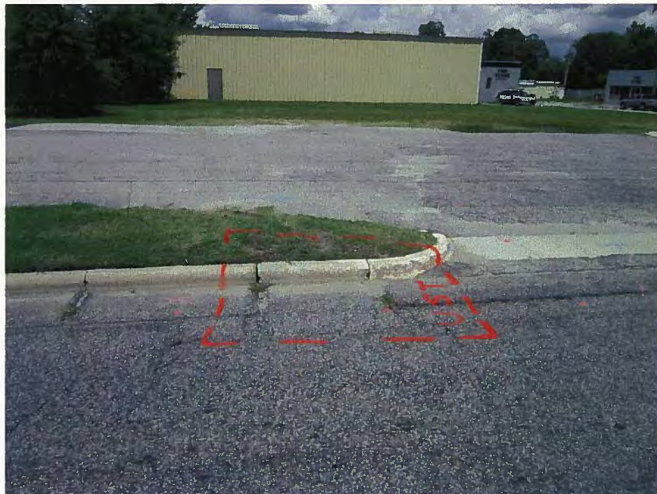
Parcel 101 (Walter L. Williams Property), looking north. Photo shows approximate marked location of probable UST No. 1 near the southwest corner of the parcel.
