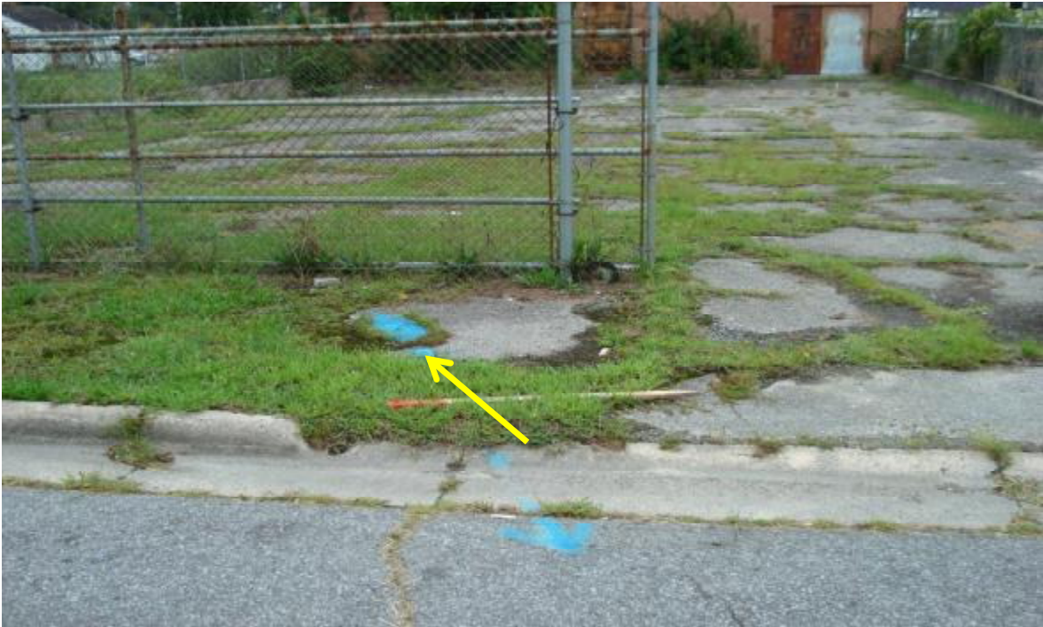
Water meter with service to building on Parcels 55 and 172
