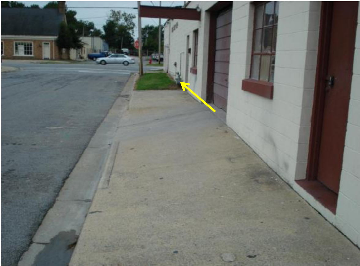
Gas meter and service to building along Spruce Street
