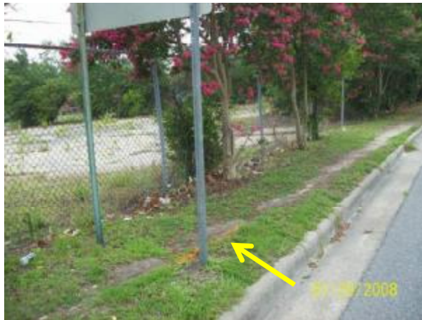
Property shown from Farmville Blvd looking west Picture shows fiber optic cable delineated in orange
