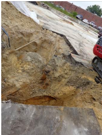
Photo #11 UST Extents Determined
