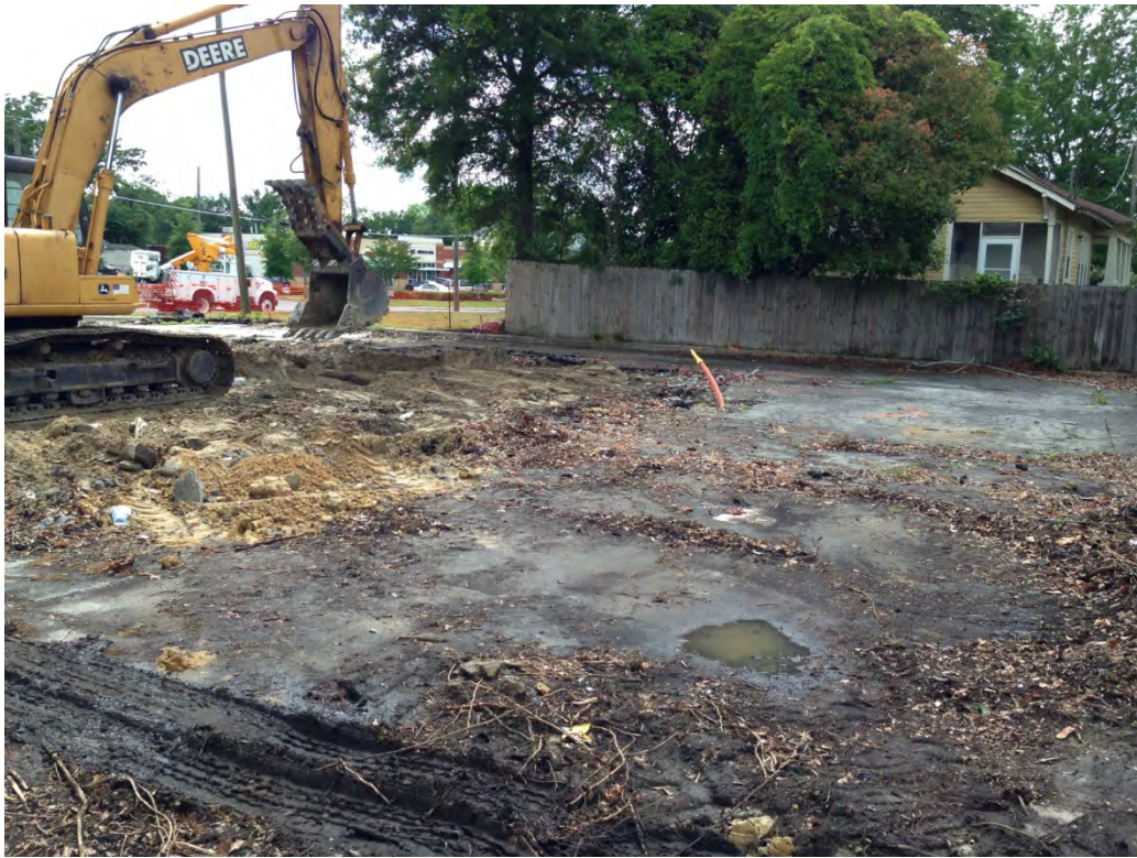
Photograph 1: View of Stadium Cleaners prior to excavation. View is to the Southwest.
