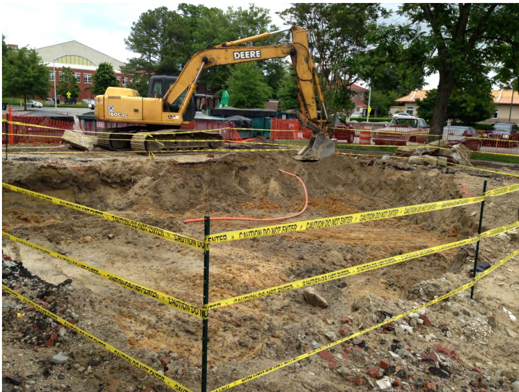
Photograph 4: View of the Stadium Cleaners excavation in progress. View is to the Northeast.
