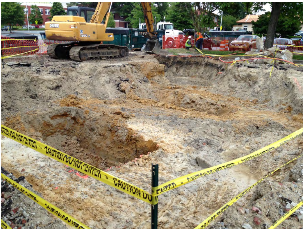
Photograph 6: View of the Stadium Cleaners excavation in progress. View is to the Northeast.
