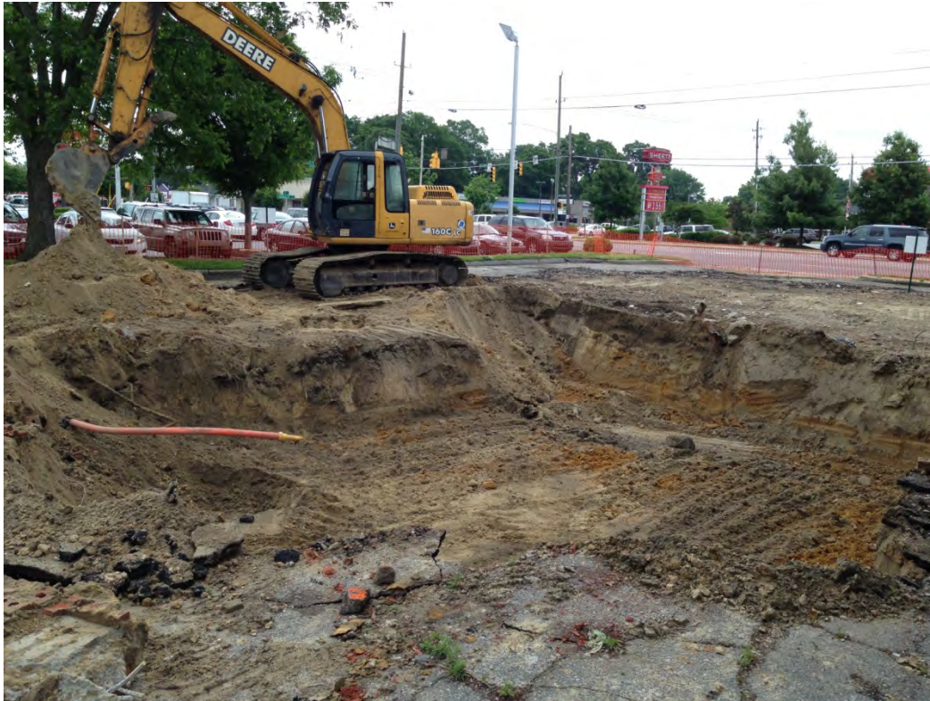
Photograph 3: View of the Stadium Cleaners excavation in progress. View is to the Southeast.
