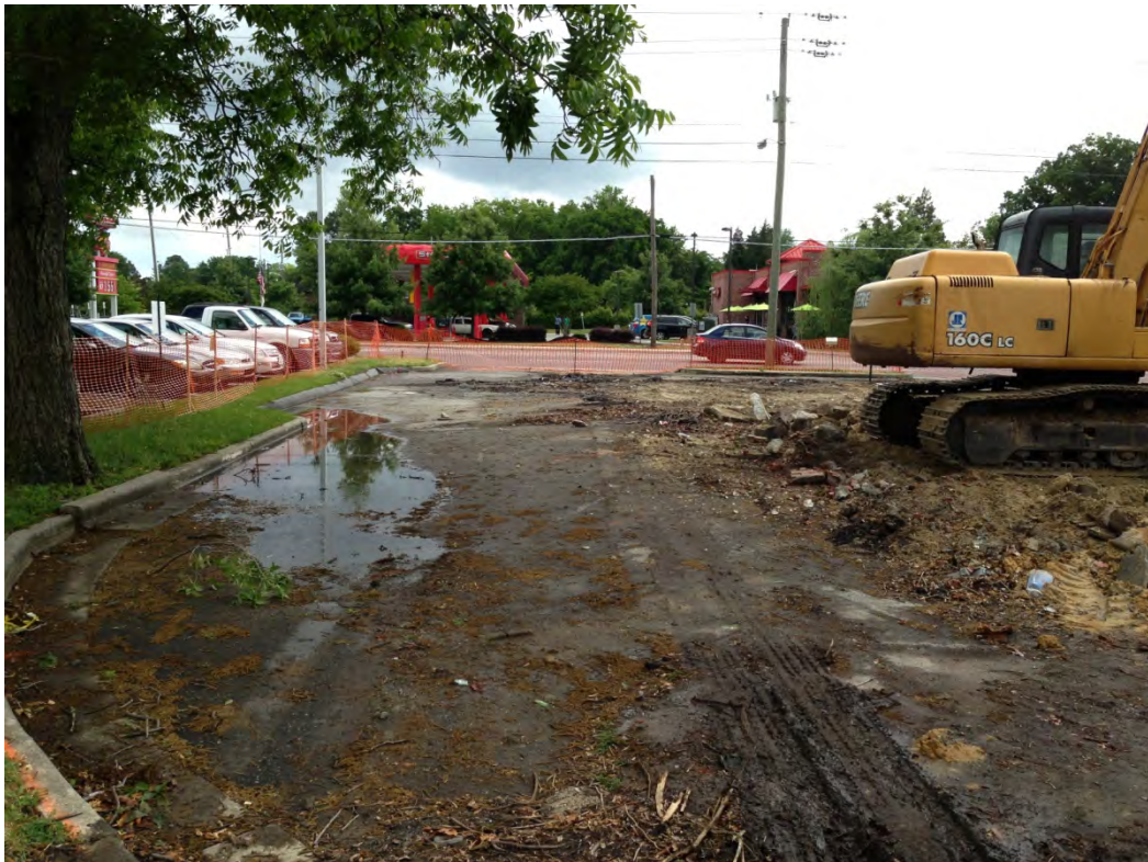
Photograph 2: View of Stadium Cleaners prior to excavation. View is to the South.
