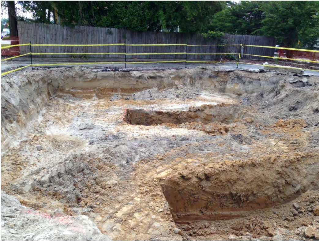
Photograph 5: View of the Stadium Cleaners excavation in progress. View is to the West.
