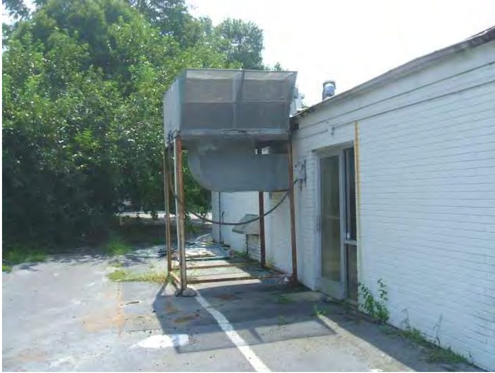
A monitoring well is located in the bottom portion of the picture. An old ventilation duct can be seen protruding from the rear of the building.
