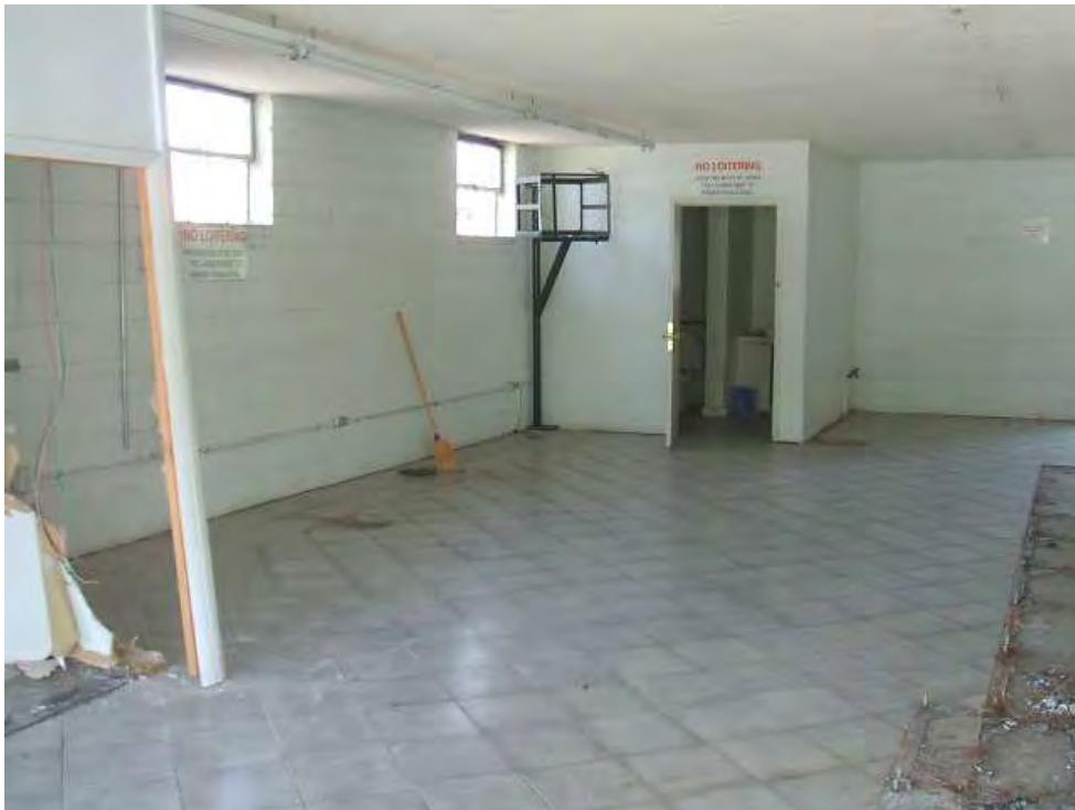
A view looking toward the Northwest rear of the facility where a bathroom is located.
