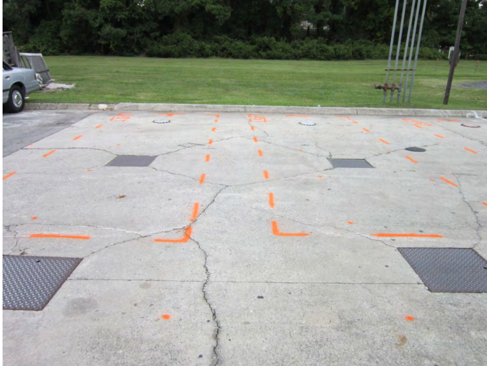
Parcel 48 (RI CS5, LLC Property), looking north. Photo shows approximate marked location of known UST Nos. 1 and 2 near the northwest corner of the building.
