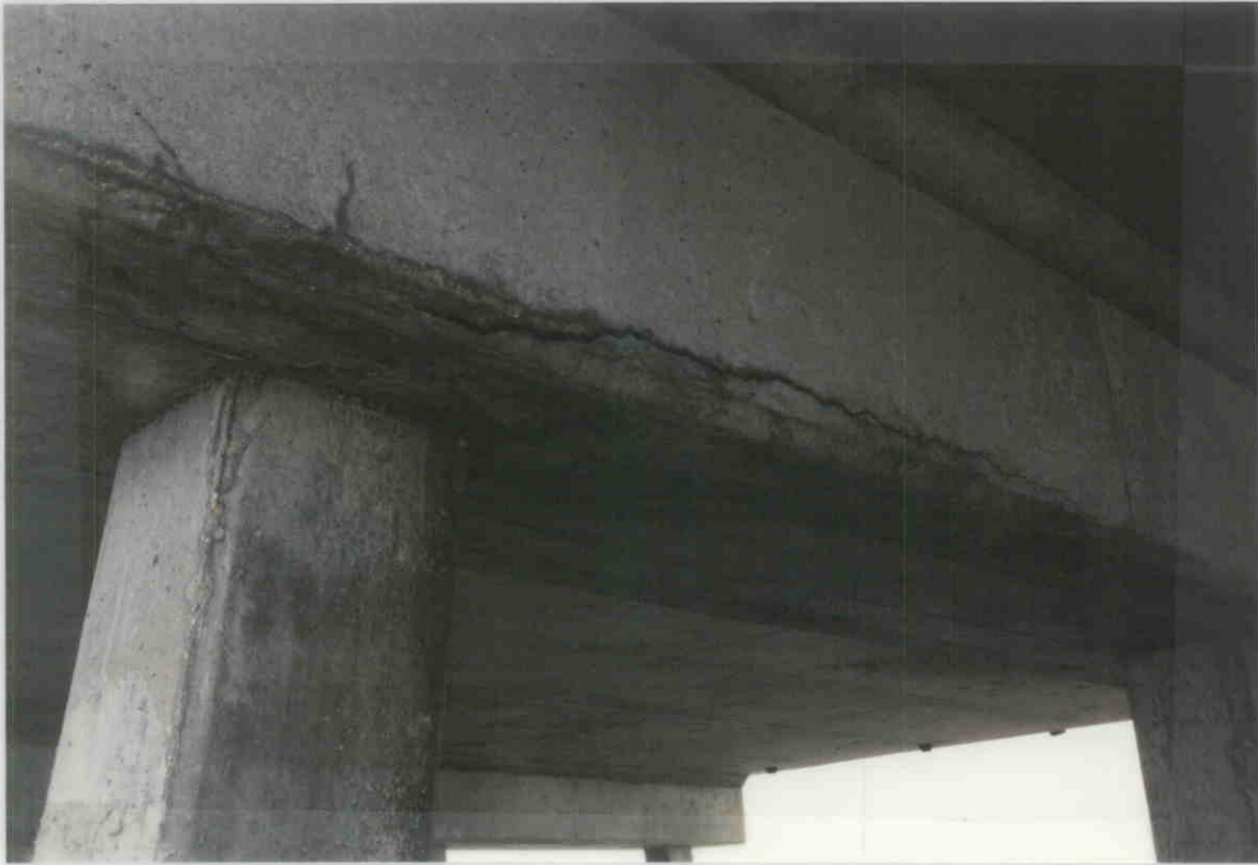
SIM. CRACKS/DELAM. @ RANDOM CAPS.
