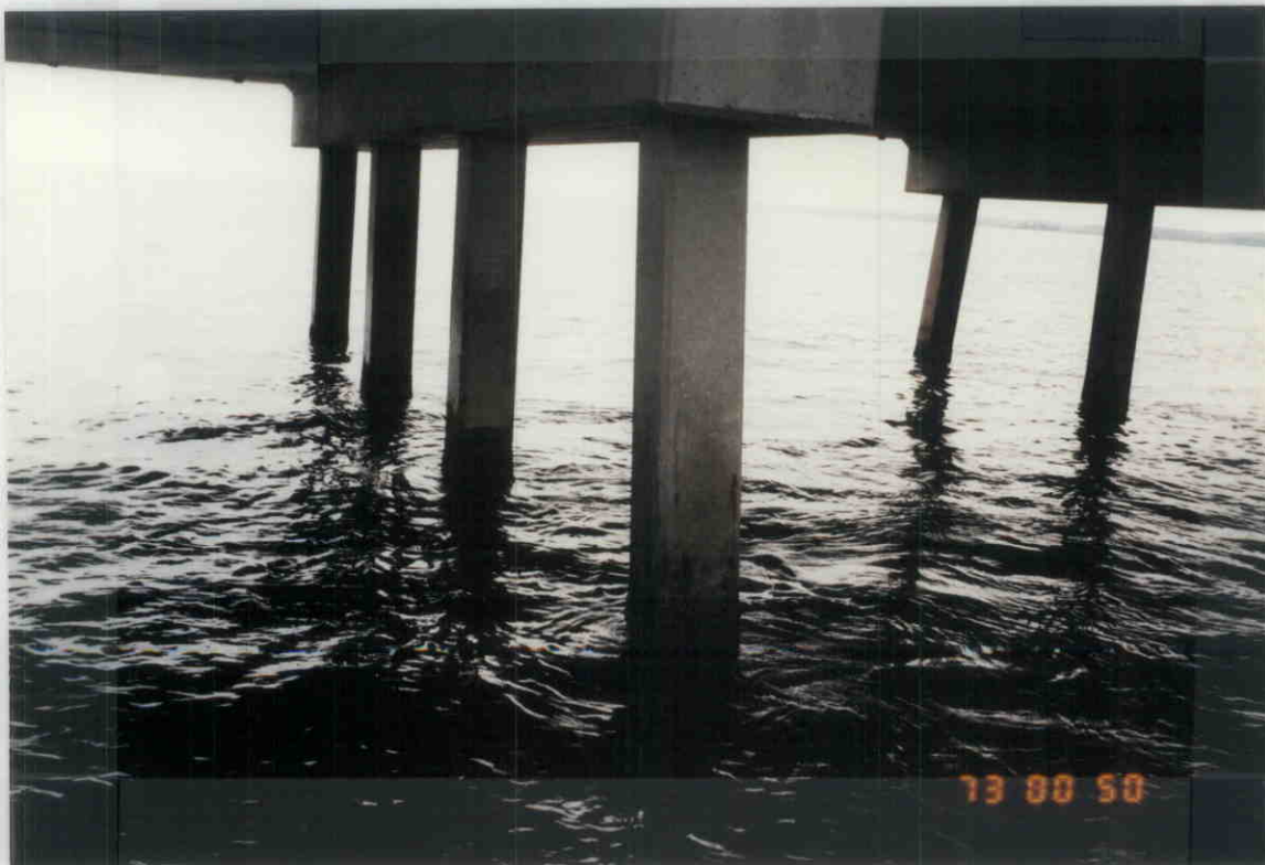
SIM. CRACKS WITH RUST STAINS.
