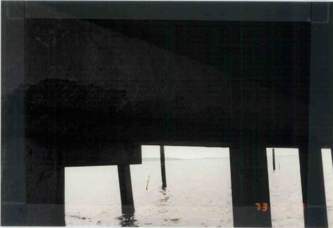
SIM. SPALLS @ BT. CAPS. (BT.4, SPAN4)
