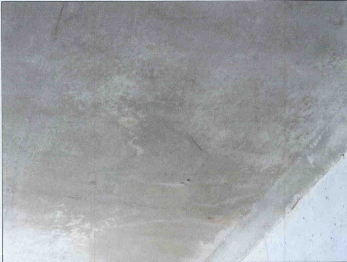
SPAN 16 DECK UNDERSIDE CRACKED & DELAMINATED 1-1/2' OUT FROM BT.15 CAP BETWEEN PILES 3 & 4.
