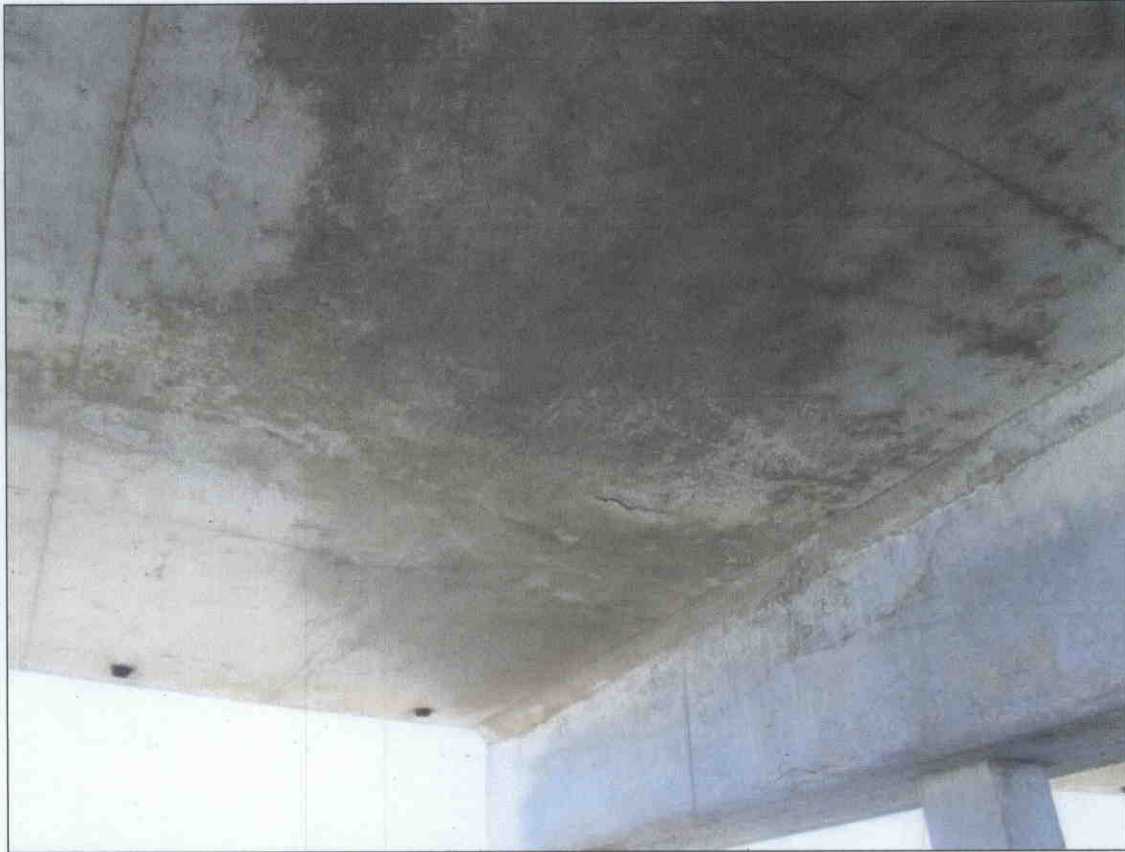
SPAN 21 DECK UNDERSIDE CRACKED & DELAMINATED 2' OUT FROM BT.20 CAP BETWEEN PILES 3 & 4.
