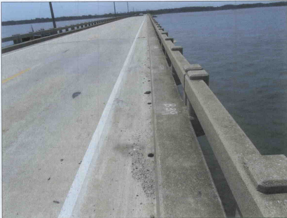
SCATTERED DEBRIS ALONG THE LEFT CURB.
