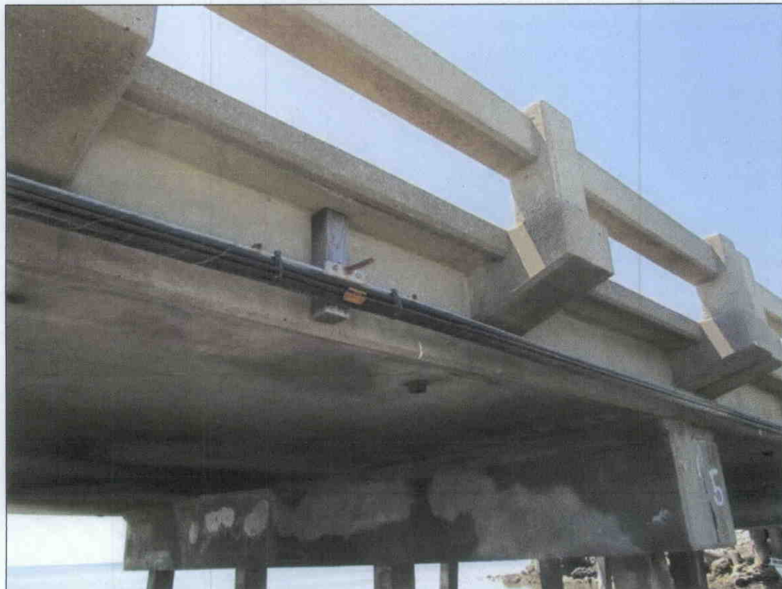
CABLE UTILITY ALONG THE NORTH SIDE.
