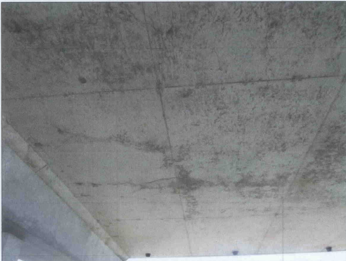
SPAN 29 DECK UNDERSIDE LONGITUDINALLY CRACKED & DELAMINATED 3- 4' BACK FROM BT.28 CAP RIGHT OF PILE 3.
