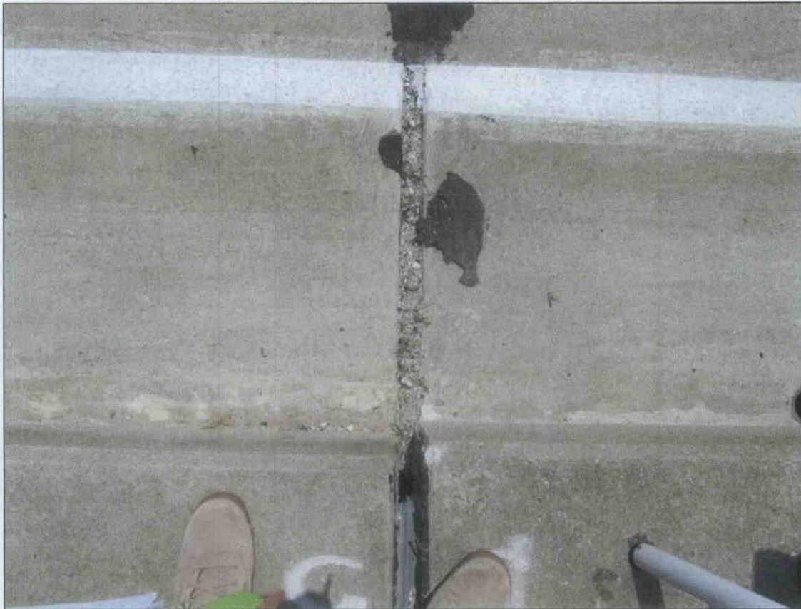
JOINT MATERIAL MISSING & FILLED WITH DEBRIS @ THE LEFT SHOULDER @ BT.5. SIMILAR @ THE RIGHT SHOULDER & RANDOM BTS.
