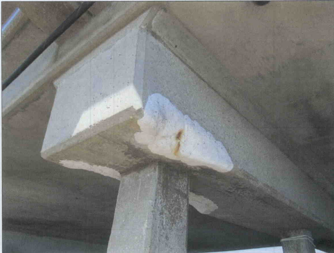
BT.3 CAP REPAIR NEAR THE RIGHT END IN SPAN 4 HAS RUST STAIN BLEEDING THRU.
