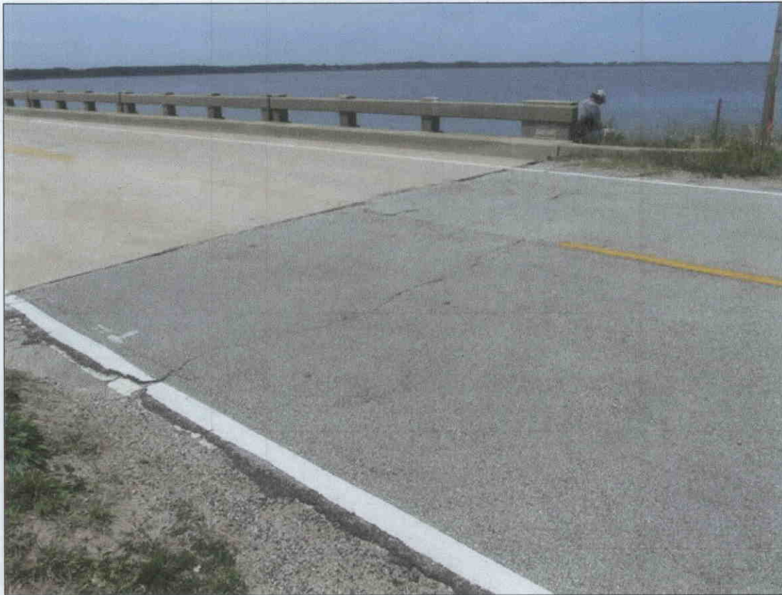
EAST APPROACH TRANSVERSE CRACKED & WEARING SURFACE IS HIGHER THAN THE SPAN 47 DECK CAUSING IMPACT.
