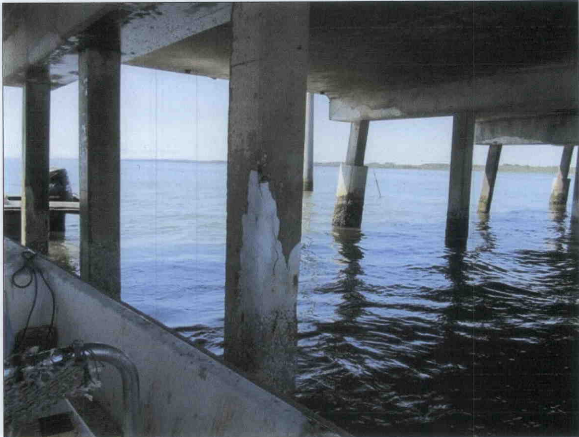
PILE 2 @ BT.34 PATCHED, CRACKED & DELAMINATED @ THE NE CORNER.
