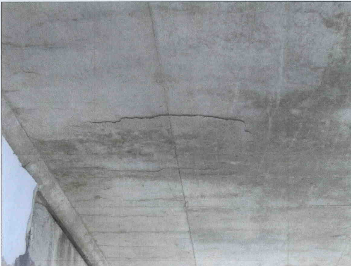
SPAN 20 DECK UNDERSIDE CRACKED & DELAMINATED 3' BACK FROM BT.20 CAP BETWEEN PILES 1 & 2.
