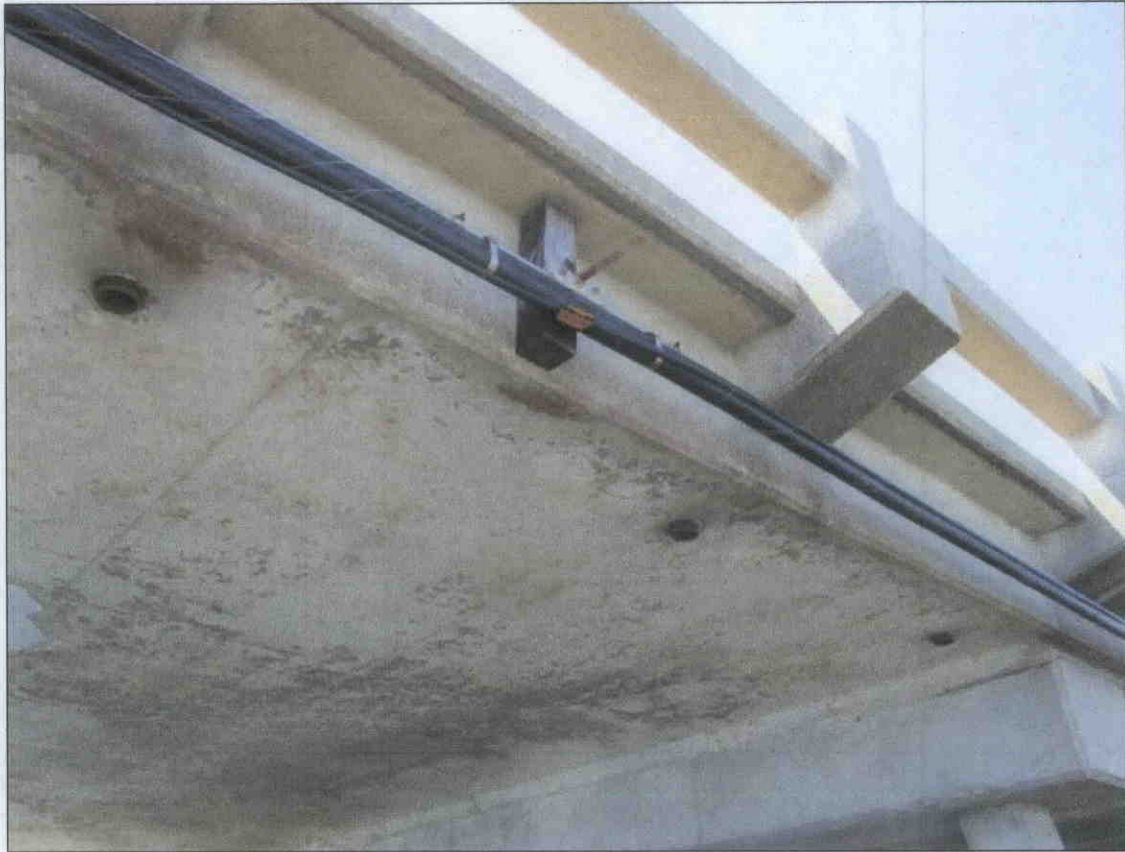
SPAN 30 DECK UNDERSIDE DELAMINATED ALONG THE LEFT EDGE @ MIDSPAN.
