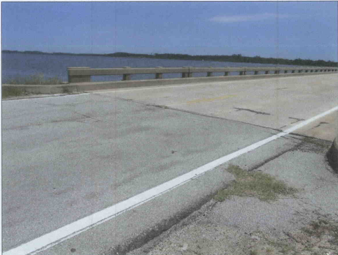
WEST APPROACH TRANSVERSE CRACKED & UNEVEN.
