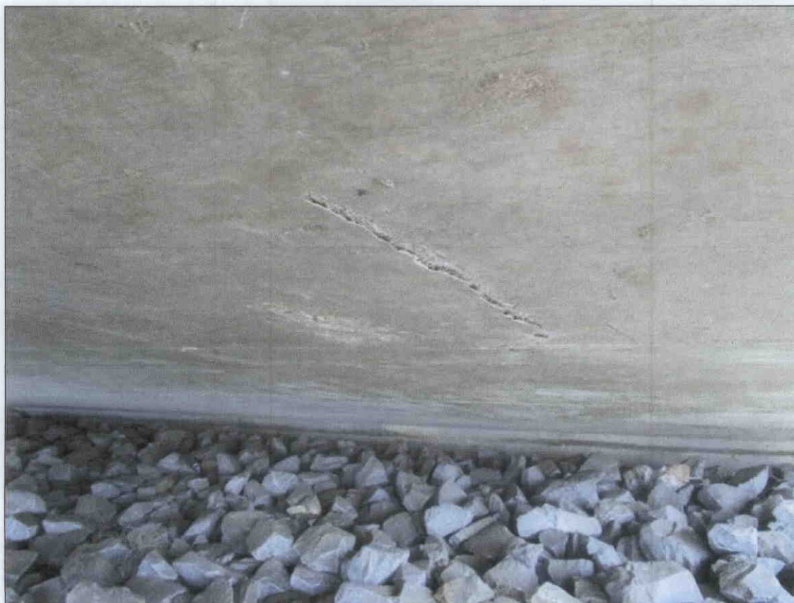
SPAN 47 DECK CRACKED & DELAMINATED 6' OUT FROM BT.46 & 4' FROM THE RIGHT EDGE OF DECK.
