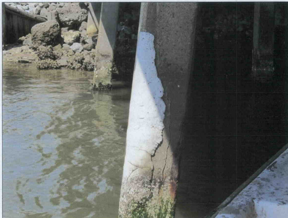
PILE 4 @ BT.3 PATCHED & VERTICALLY CRACKED WITH RUST STAINS.
