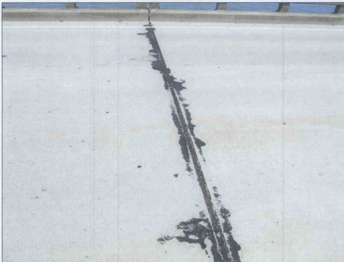
STANDARD JOINT MATERIAL DETERIORATED & PULLED LOOSE ALONG THE EDGES @ BT.10.
