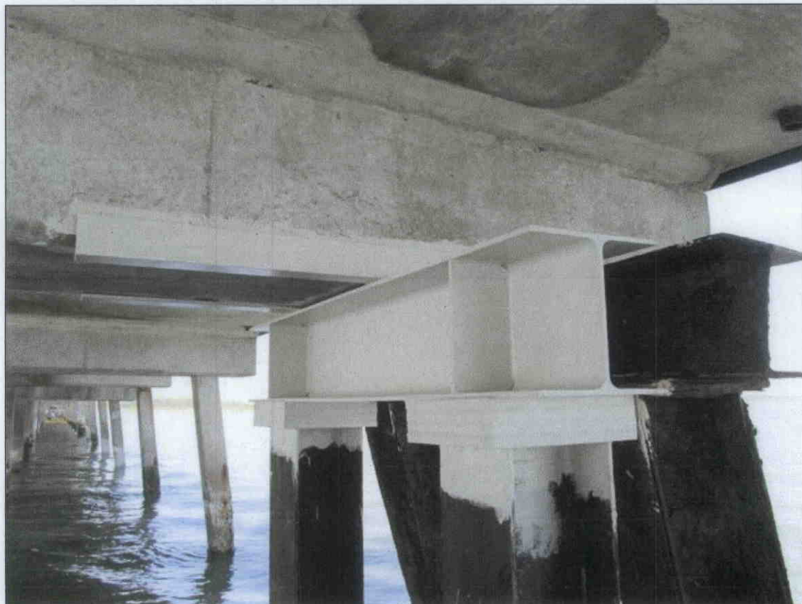
BT.40 REPLACEMENT CRUTCHBENT WITH NEW CAP & STEEL BEARING PLATES @ THE PILE 1 POSITION.
