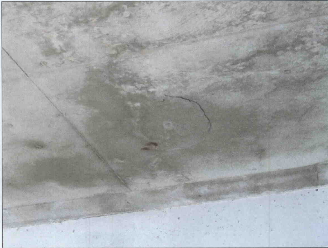
SPAN 12 DECK UNDERSIDE CRACKED & DELAMINATED WITH RUST STAIN 3' OUT FROM BT.11 CAP BETWEEN PILES 3 & 4.
