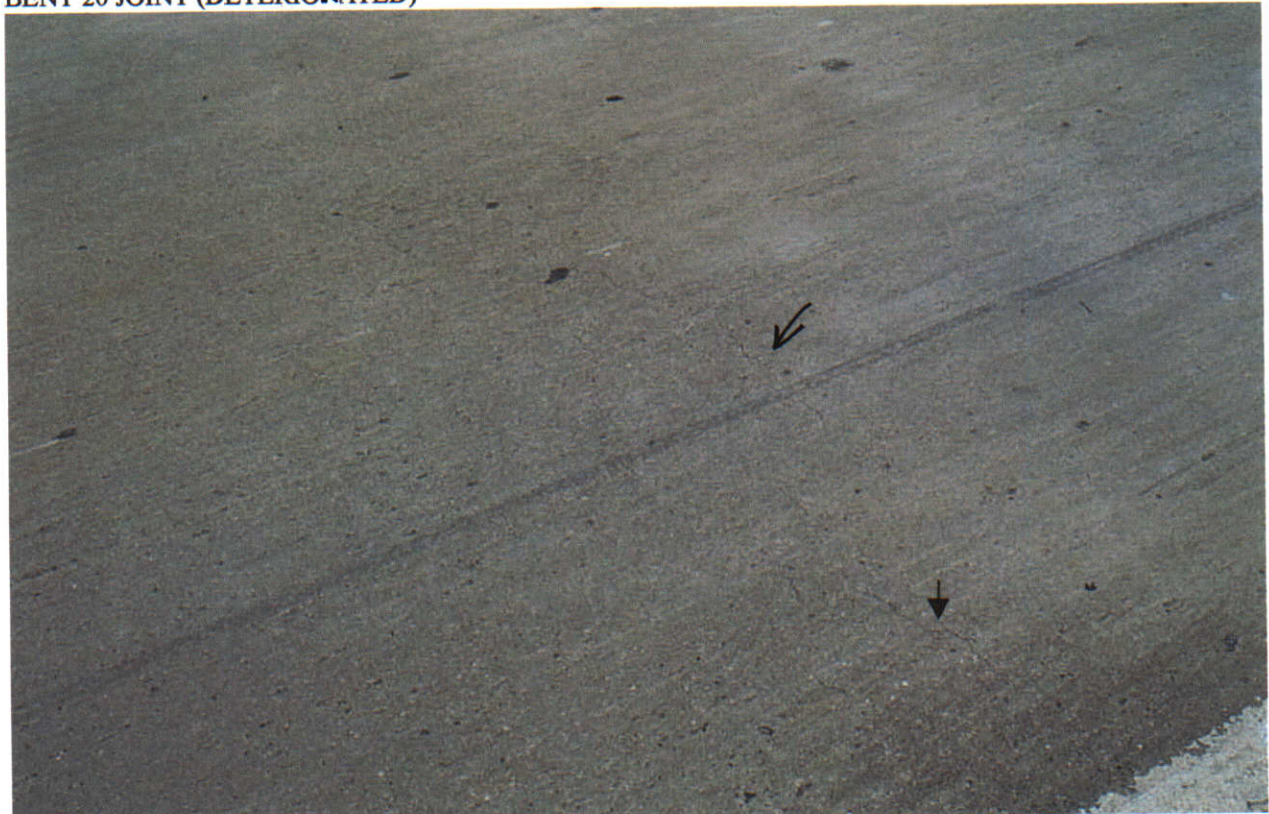
TRANSVERSE CRACKED OVER BENT 9 IN THE E.B.L.
