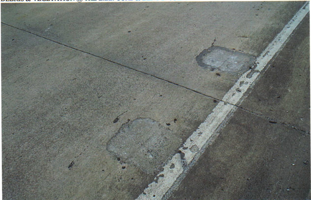
DECK PATCHES IN THE N.B.L. @ SPANS 40 & 41, BENT 40
