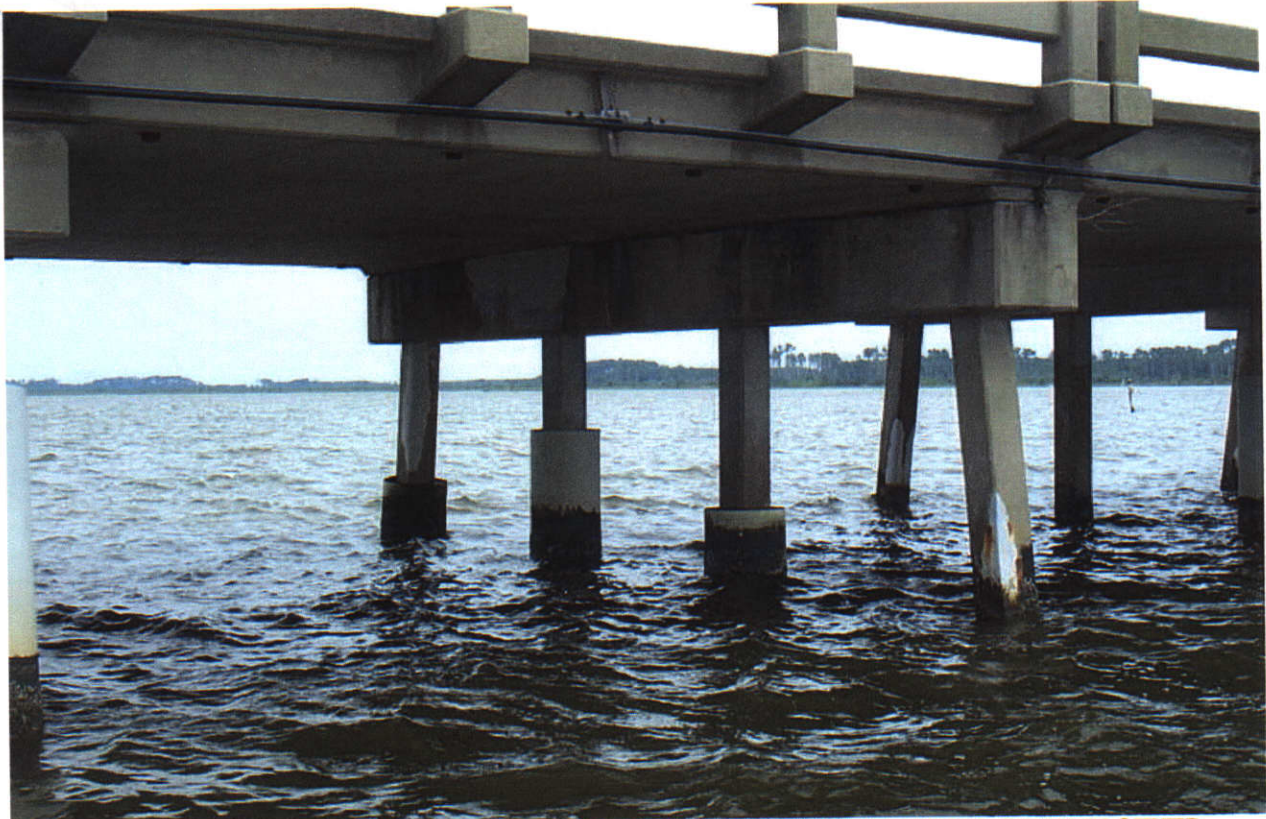
SPAN 20 SIDE OF BENT 20 (PILES 1, 2 & 3 ENCASED) (SIMILAR ENCASED PILES @ MANY OTHER BENTS)
