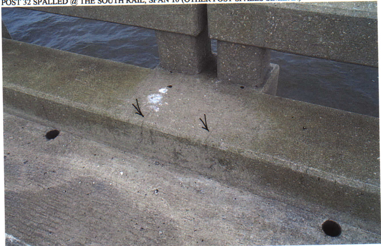
NORTH CURB CRACKED @ BENT 41
