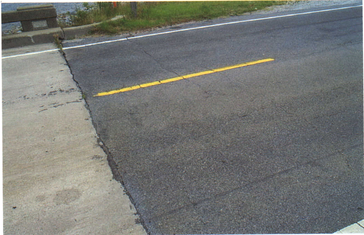
EAST APPROACH (TRANSVERSE CRACKED & MINOR SETTLED)
