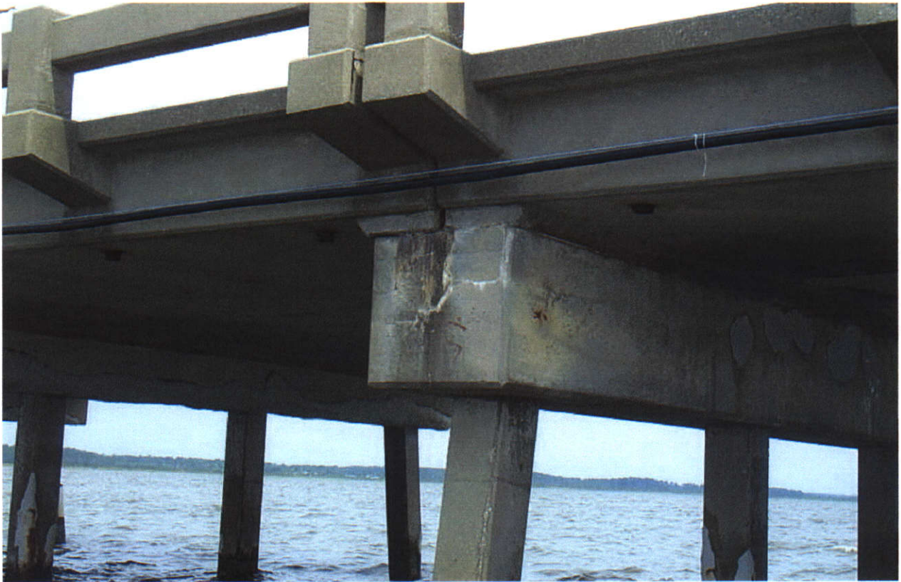
CRACKED W/ EFFLO. @ THE SOUTH END OF BENT 5 (OTHERS SIMILAR)
