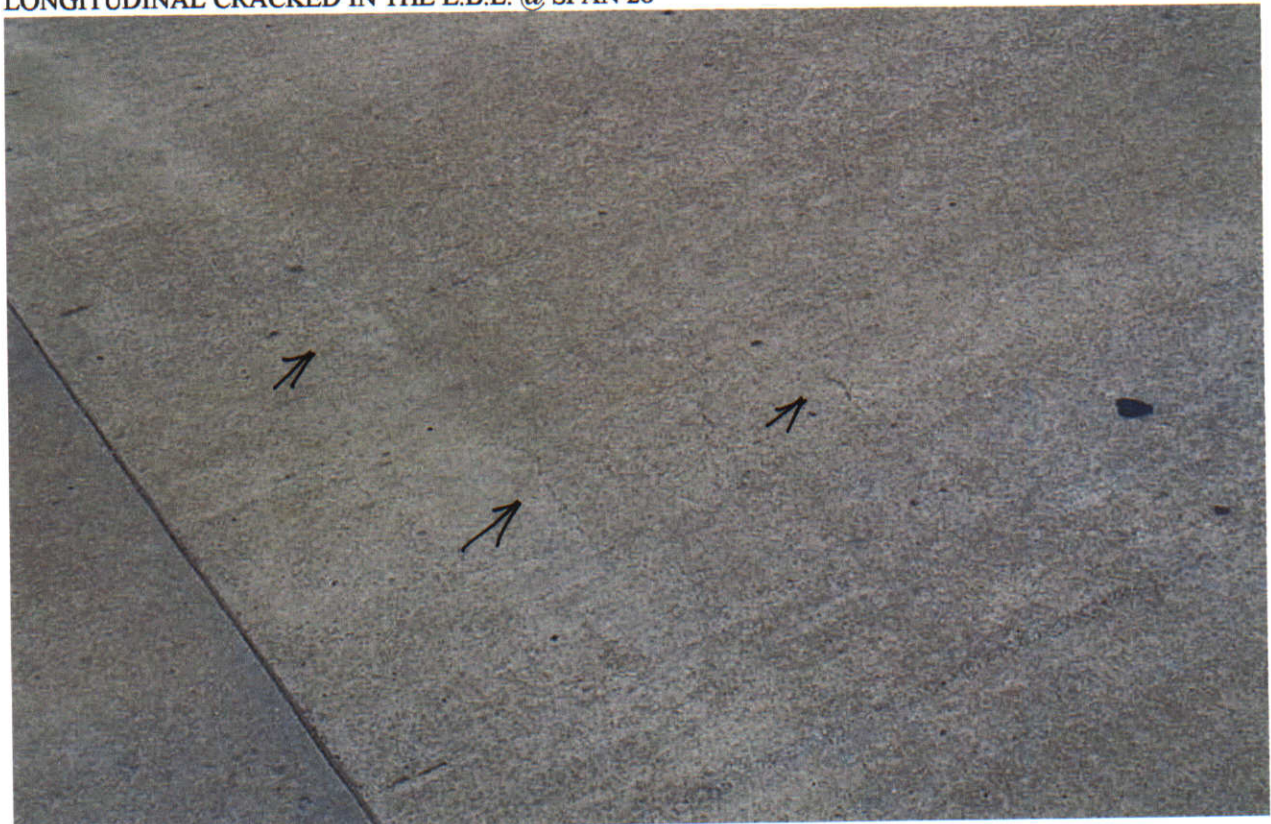
TRANSVERSE CRACKED IN THE E.B.L. @ SPAN 31
