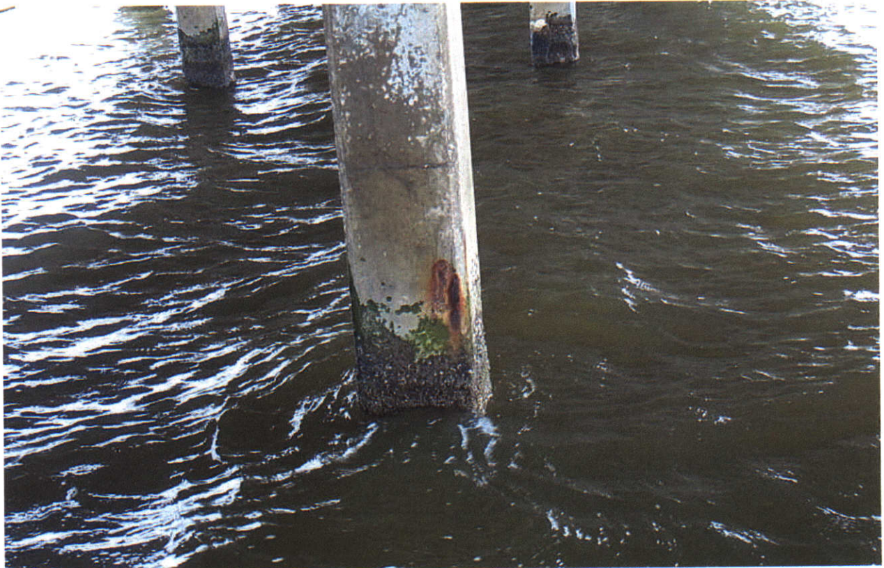
PILE 3 CRACKED & RUST STAINED @ SPAN 42 SIDE OF BENT 42
