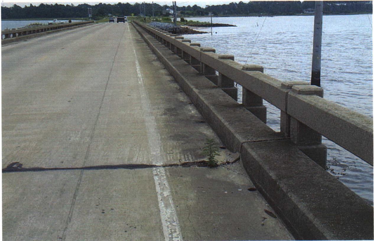
DEBRIS & VEGETATION @ THE E.BL. CURB & BENT 27 JOINT
