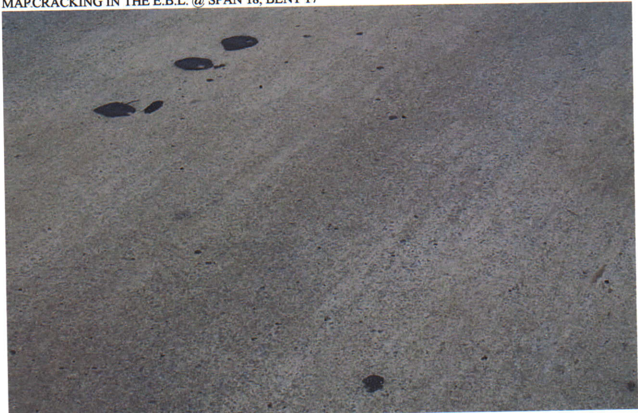
SCALING IN THE E.B.L. @ SPAN 20
