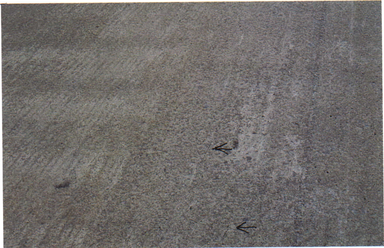
LONGITUDINAL CRACKED IN THE E.B.L. @ SPAN 28
