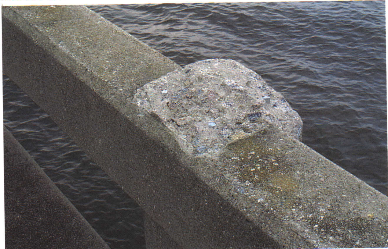
POST 32 SPALLED @ THE SOUTH RAIL, SPAN 10 (OTHER POST SPALLS SIMILAR)
