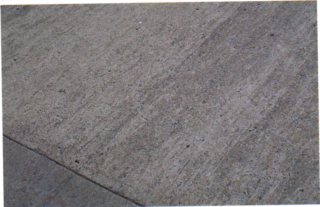
MAPCRACKING IN THE E.B.L. @ SPAN 18, BENT 17
