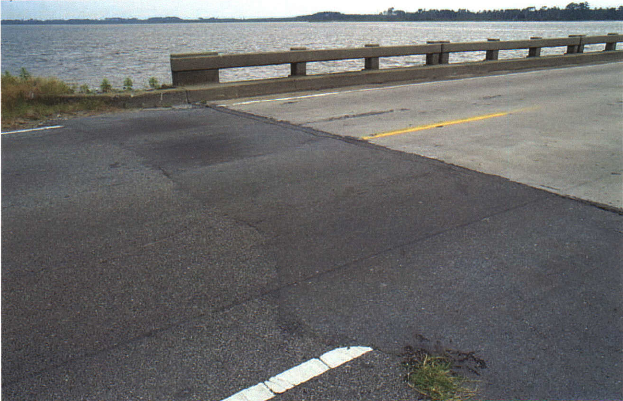
WEST APPROACH (TRANSVERSE CRACKED & MINOR SETTLED)
