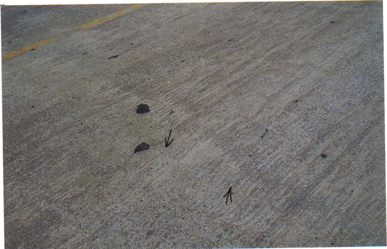
TRANSVERSE CRACKED IN THE E.B.L. @ SPAN 32
