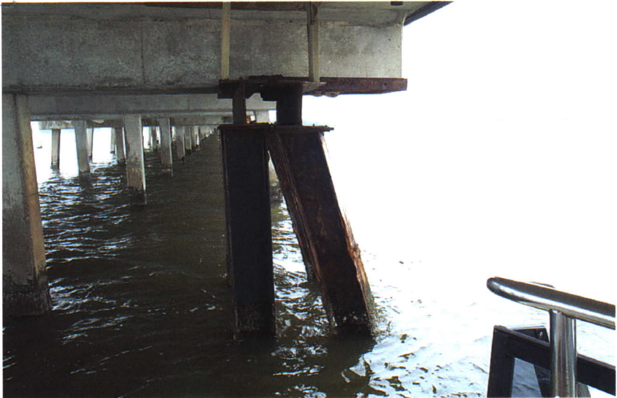
MARINE GROWTH & MINOR CORROSION ON REPLACEMENT STEEL CRUTCHBENT @ PILE POSITION, BENT 40
