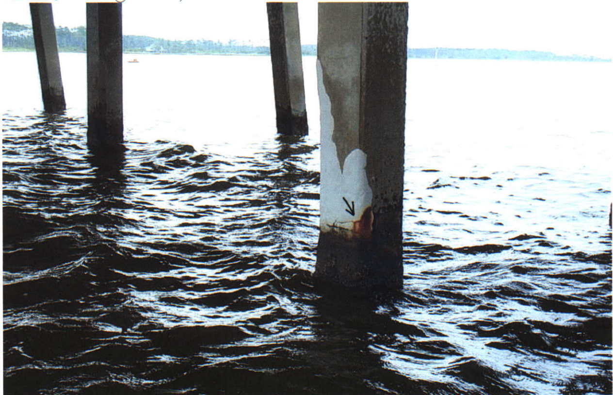
REPAIR CRACKED W/ RUST STAIN ON PILE 2 @ BENT 34
