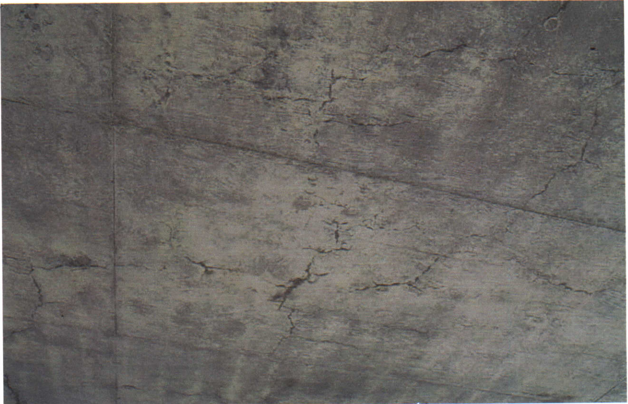
HAIRLINE CRACKED @ SPAN 13 UNDERSIDE (SIMILAR THRU OUT MOST SPANS)
