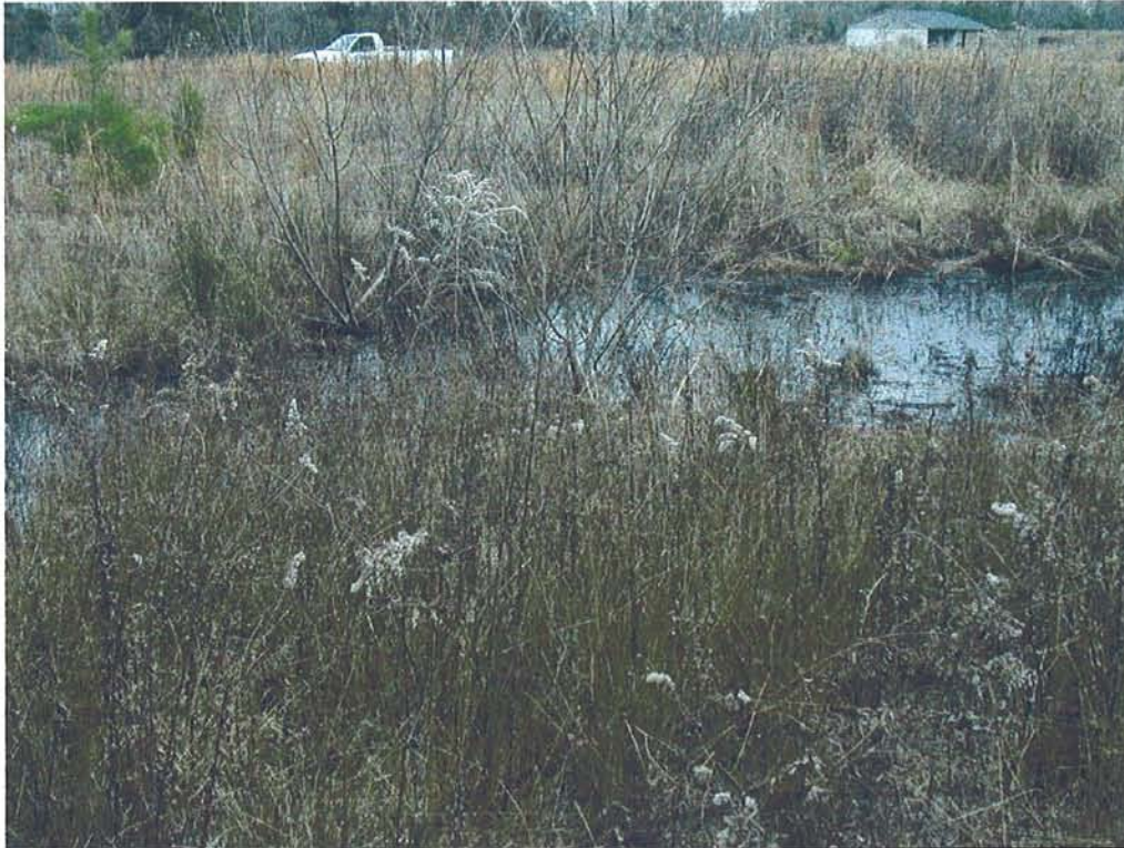
Photograph No. 3: One of three areas of ponding on the landfill cap. This area is approximately 1/10 of an acre.
