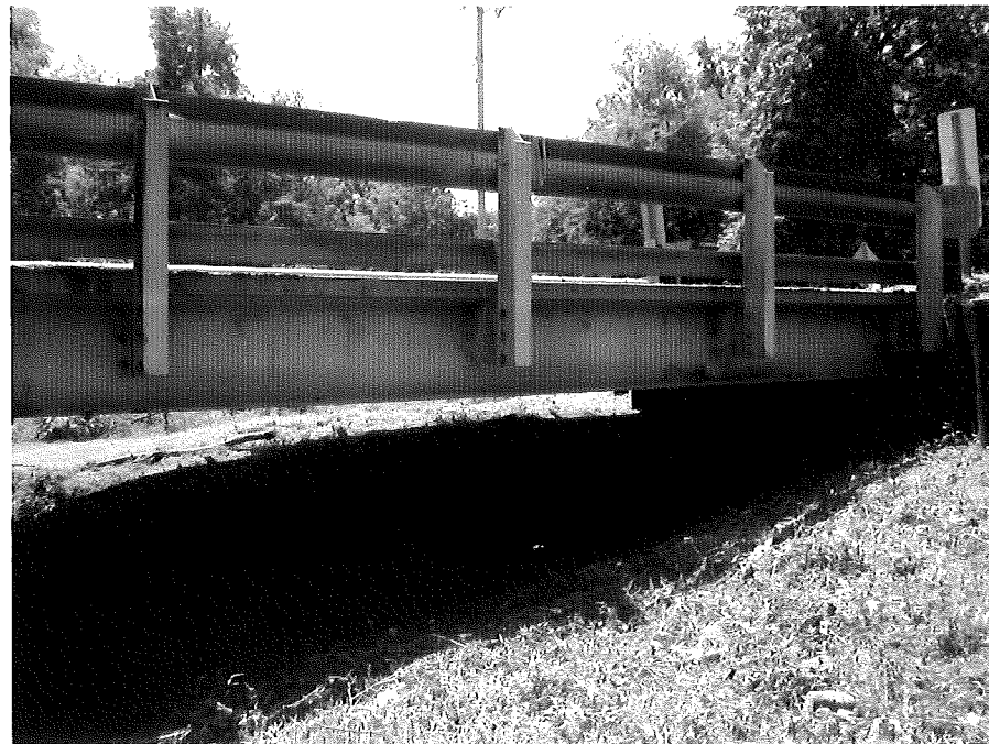
Photograph No. 6: This photograph was taken from the left side of the -L- alignment, looking southeast, across proposed Interior Bent No. 2.
