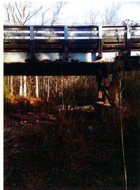
Photograph No. 6 Looking North across Bent No. 1 Bridge No. 178 in Moore County
