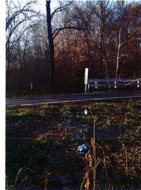
Photograph No. 7 Looking South across End Bent No. 2 Bridge No. 178 in Moore County
