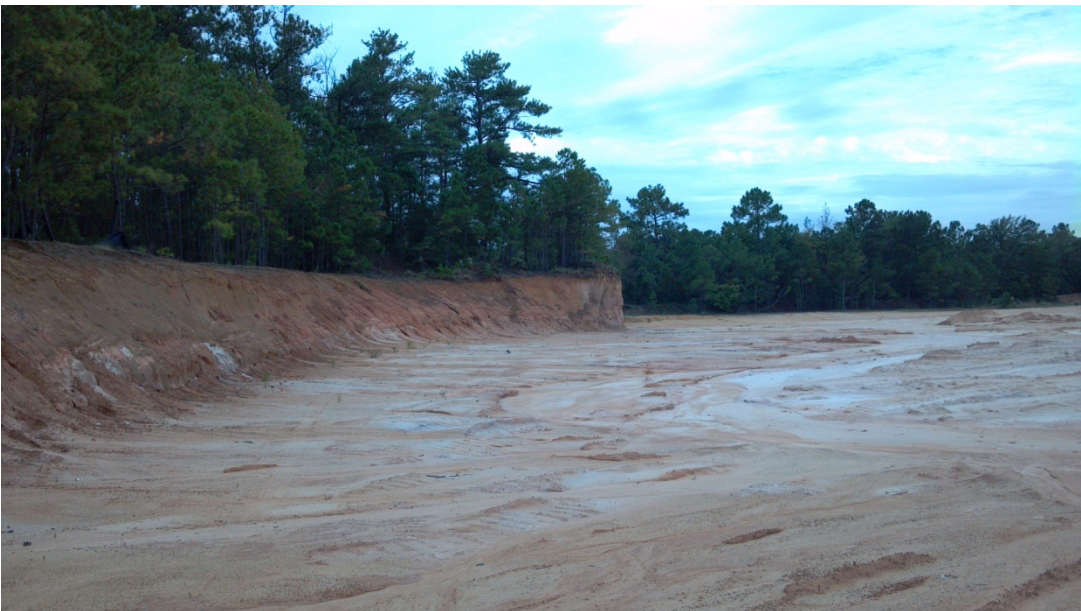
Photo #6: The southwestern portion of the site showing the current borrow pit area And depth of borrow pit excavation.
