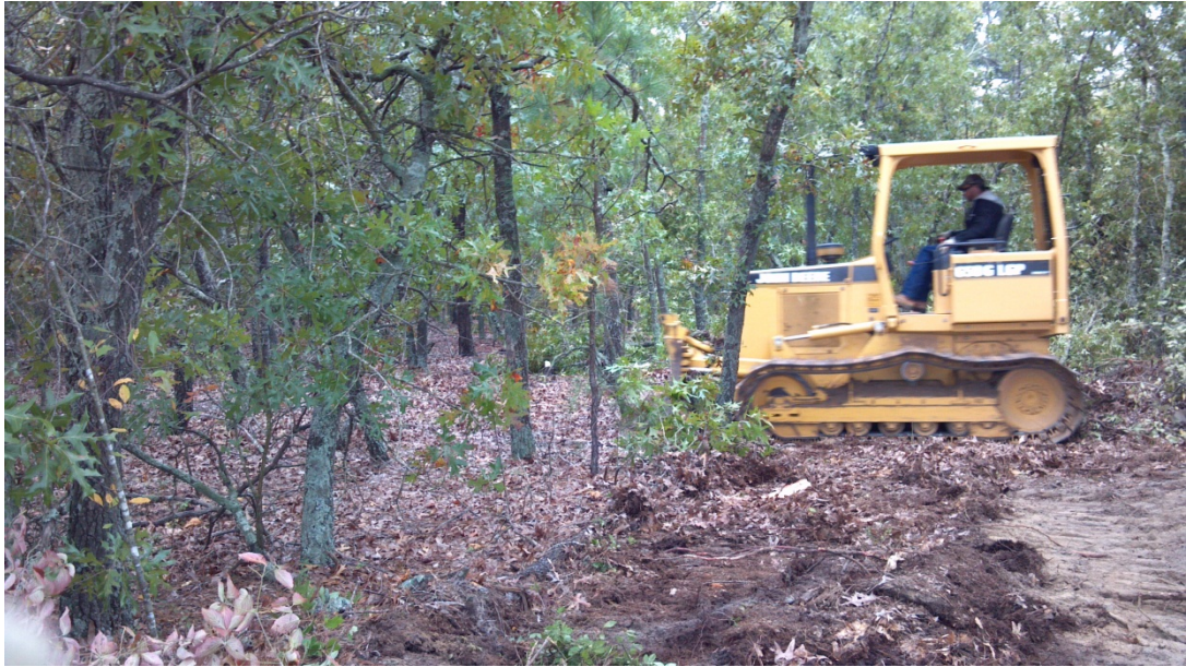
Photo #12: Dozer being used to clear path to borings where difficult access was encountered.
