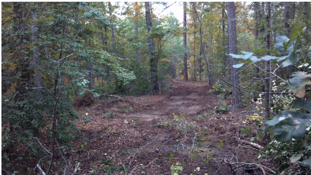
Photo #13: View of typical path upon completion of clearing with the dozer.
