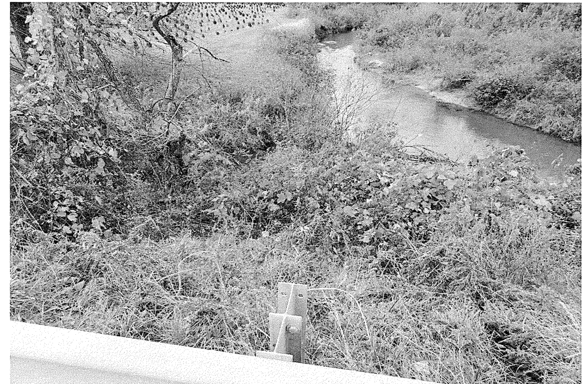
Looking down the embankment left of -L- from road side at B1
