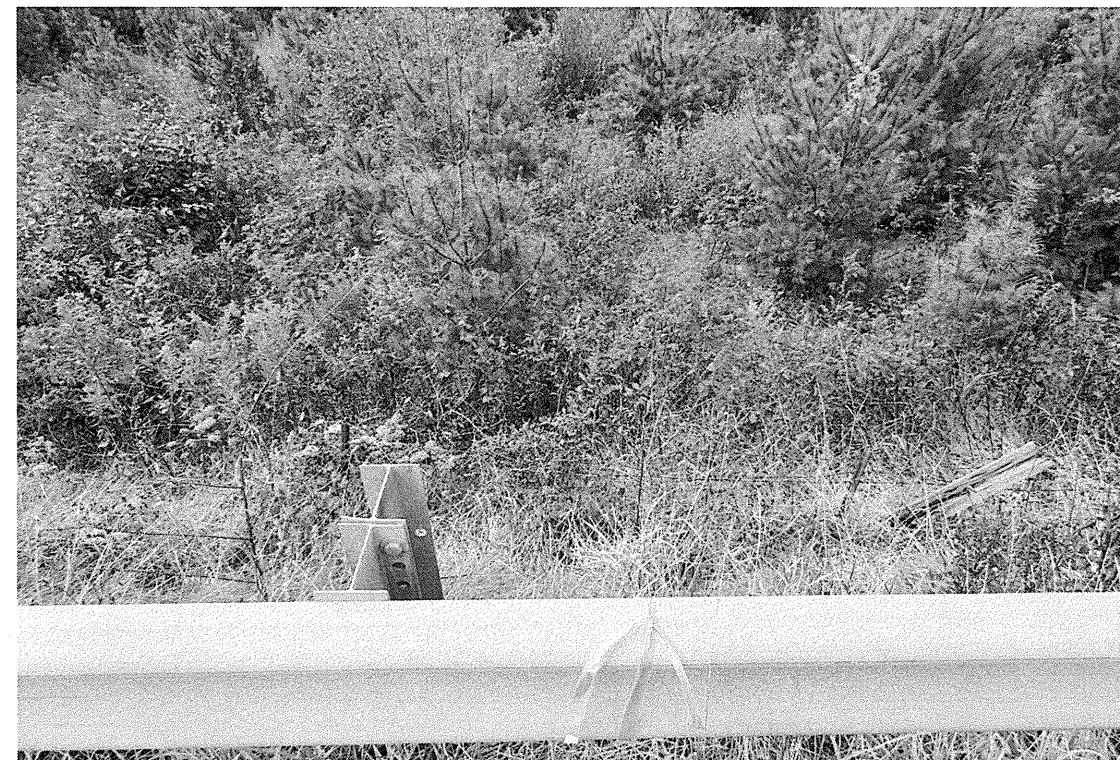
Looking down the embankment left of -L- from road side at EB2
