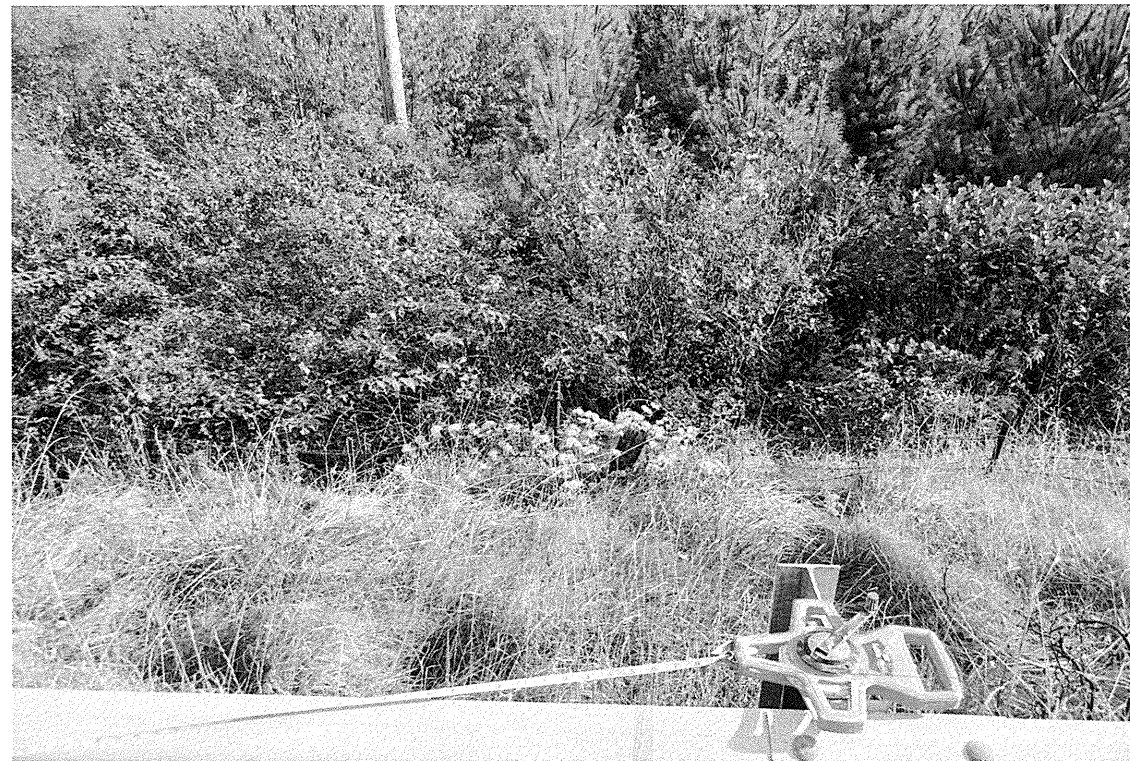
Looking down the embankment right of -L- from road side at EB1.
