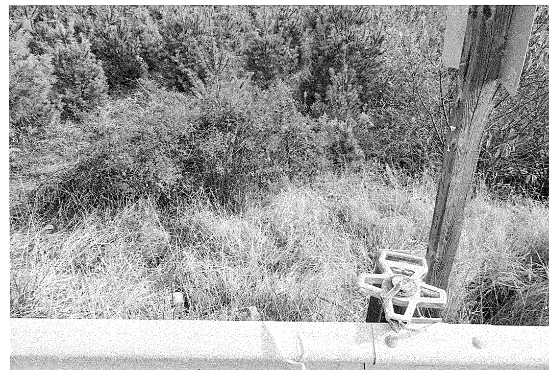
Looking down the embankment right of -L- from road side at EB2
