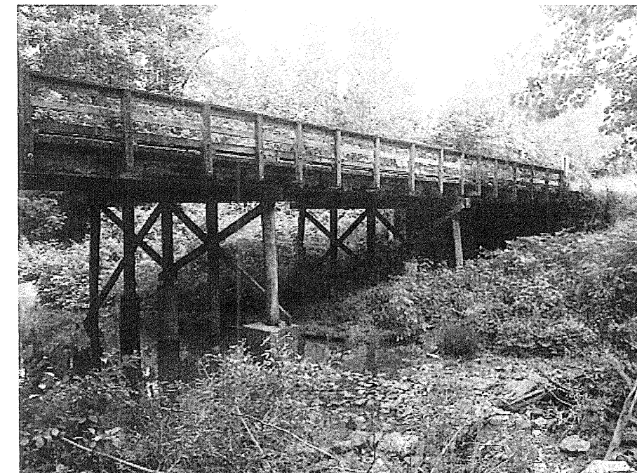
Photograph No. 4: View looking upstream towards existing Bents 1 and 2 and End Bent 2
