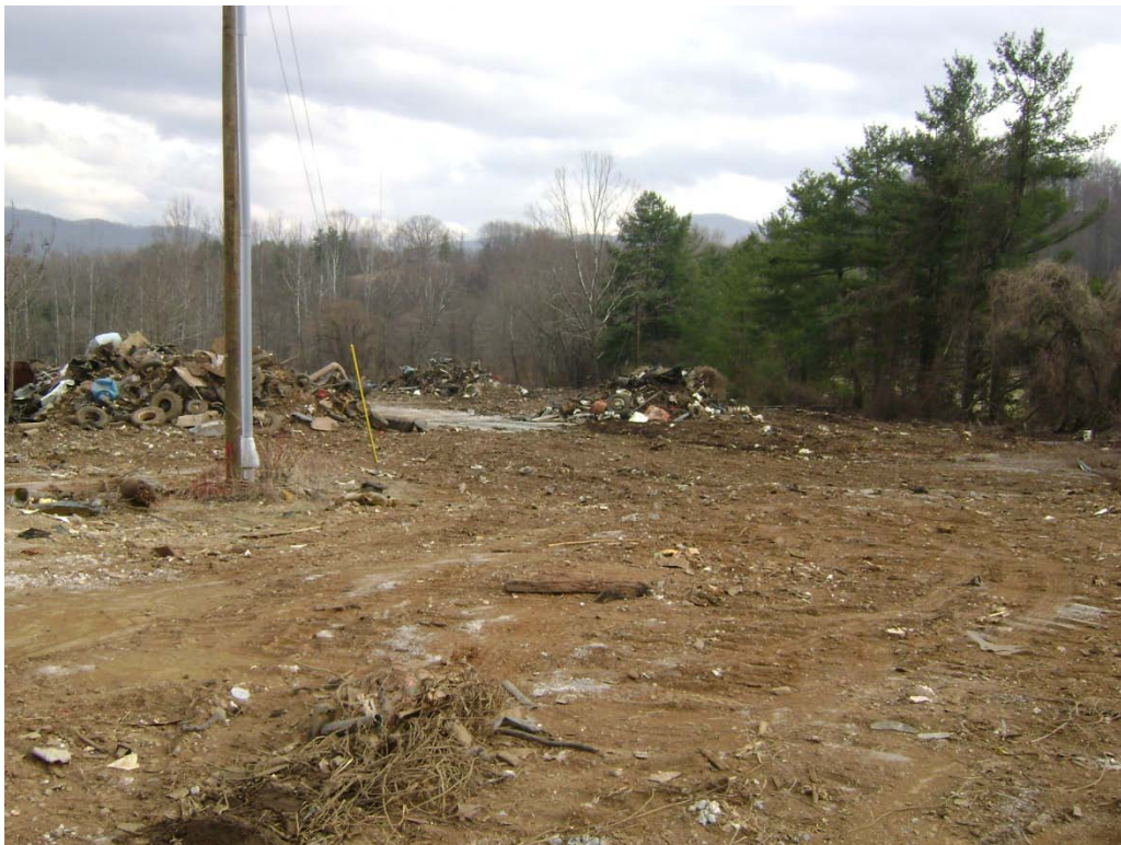
Photograph 10: View of debris pile (Area 31 behind utility pole) and surface soils mixed with small pieces of waste/debris.
