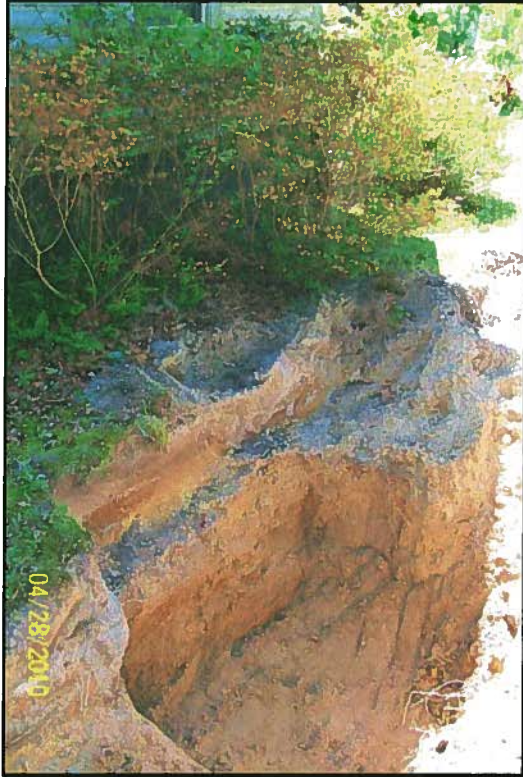
UST Excavation – Looking west across excavation towards north side of former Sellers residence
