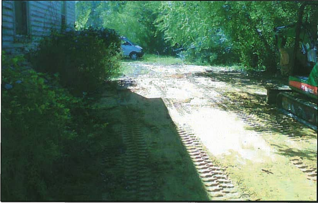
UST excavation area backfilled and compacted – Looking west from near northeast corner of former Sellers residence
