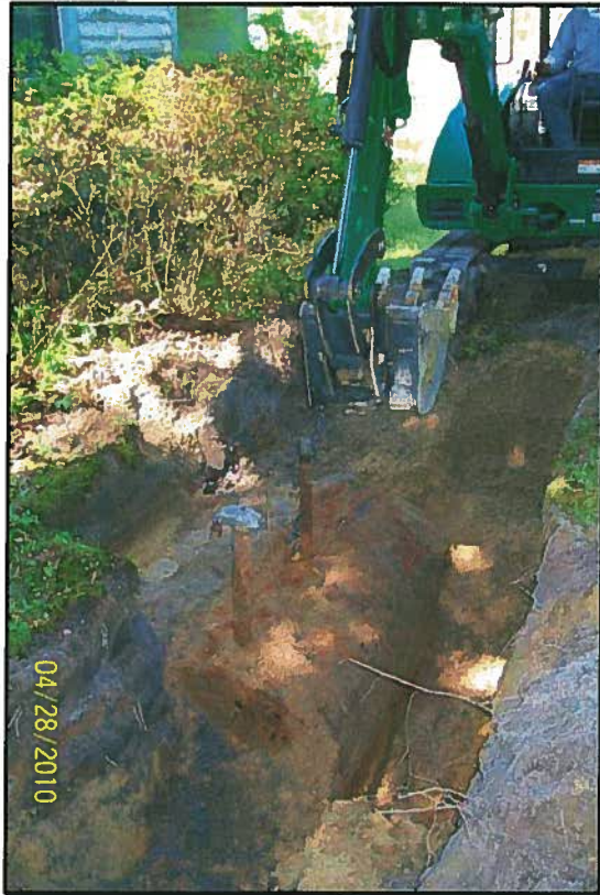
UST Excavation – Looking west along north side of former Sellers residence and UST excavation
