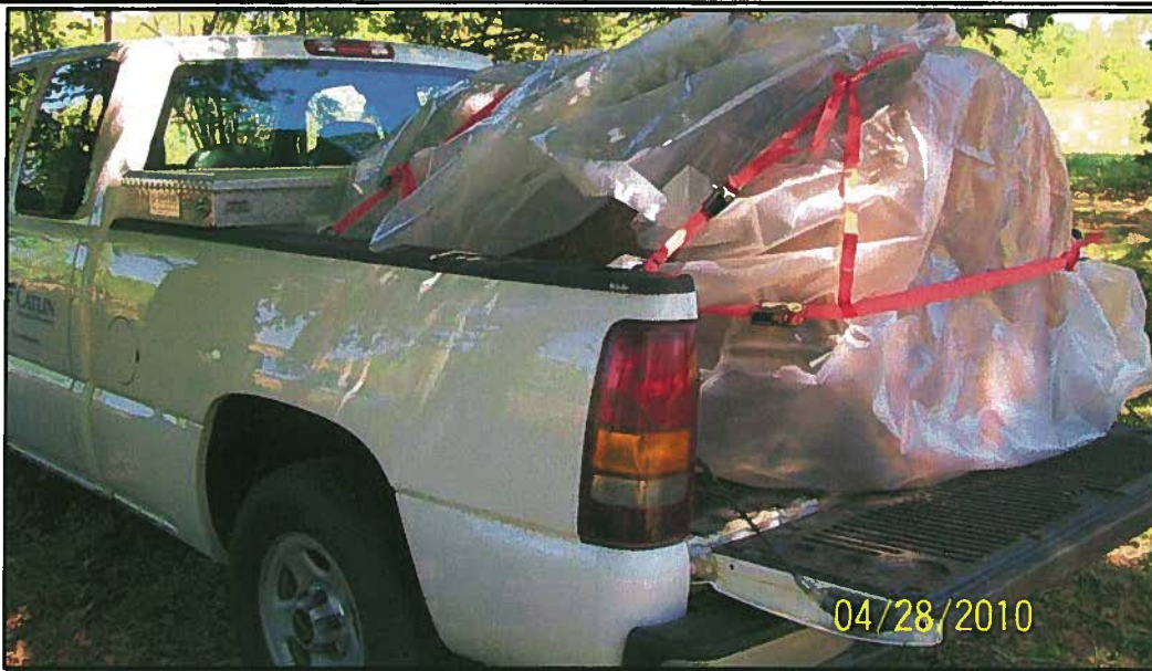
Removed UST loaded for transport to Southeast Response and Remediation for proper disposal
