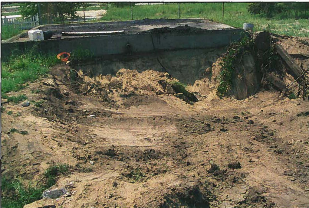
Looking west across oil-water separator excavation after collapsing sidewalls
