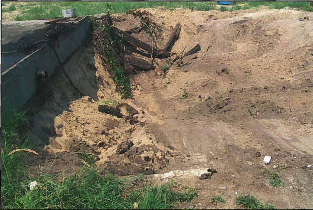
Looking north across oil-water separator excavation after collapsing sidewalls
