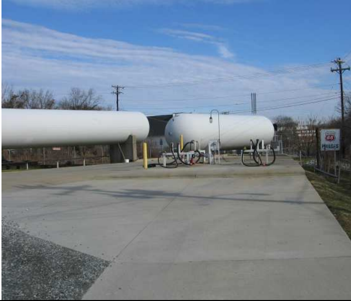
Main propane storage tanks at the eastern edge of the property.
