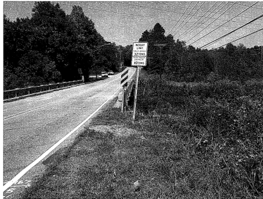
Photograph No. 1: General site view looking northeast along east side of existing bridge
