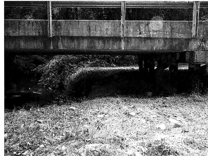
Photograph No. 3: View looking southwest at proposed Bent 1 showing remnants of old concrete structure
