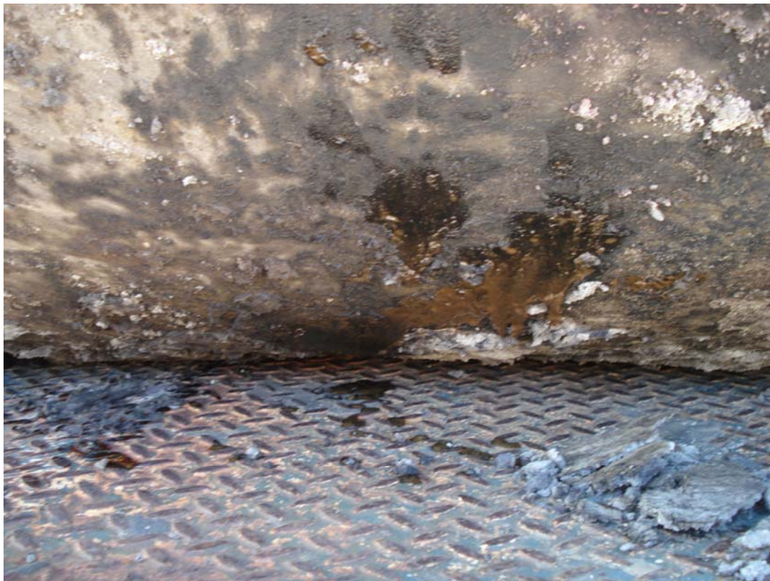
Photograph 7: View of bottom of UST #002 showing staining from release.
