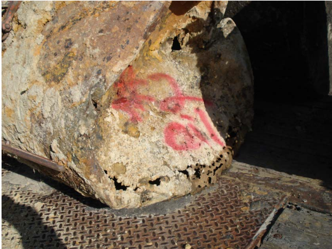
Photograph 8: View of east end of UST #003 showing corrosion.
