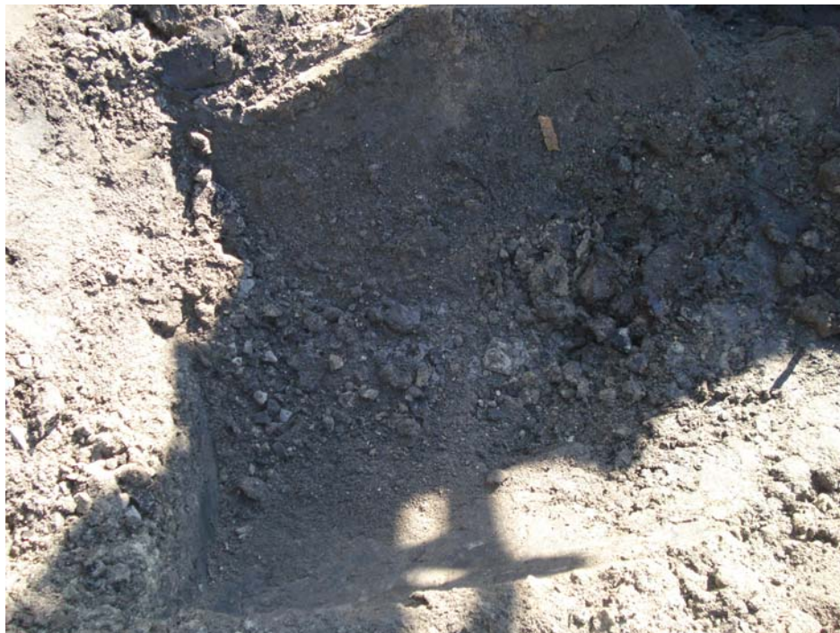
Photograph 4: View looking west at stained soil in former location of UST #002 prior to overexcavation.
