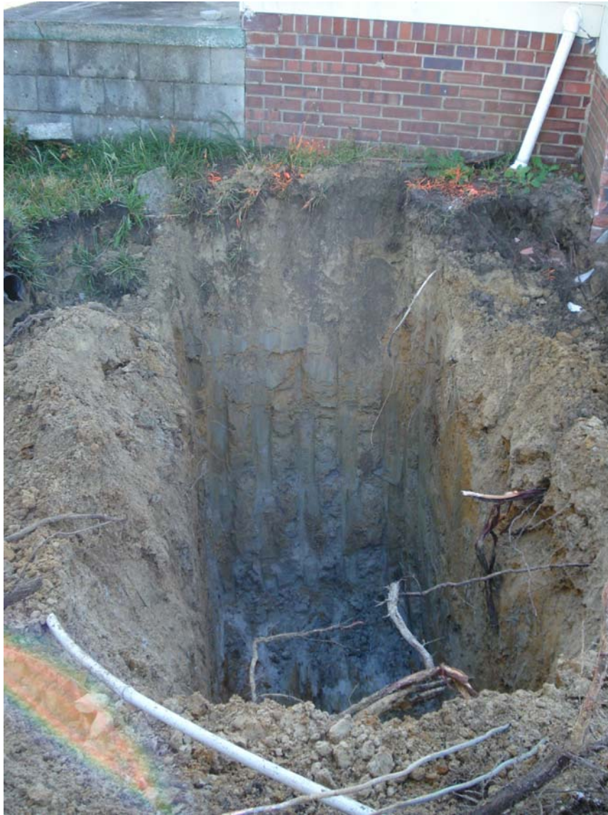
Photograph 5: View looking east at stained soil near bottom of east wall of UST #003 excavation.
