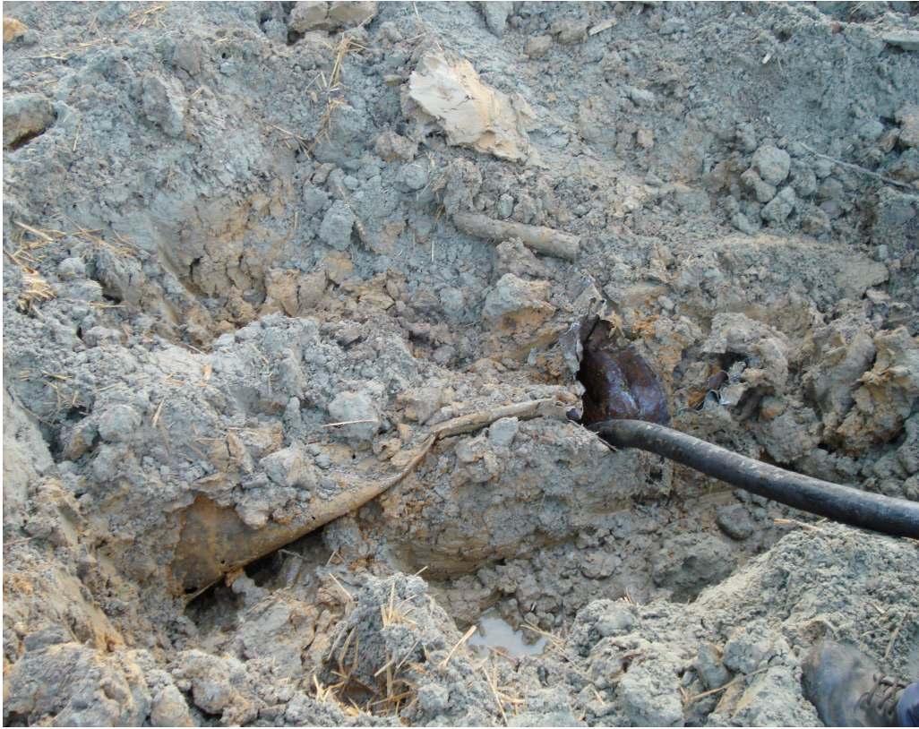
Photograph 1: Withdrawal of UST contents through hole created by contractor prior to UST removal.
