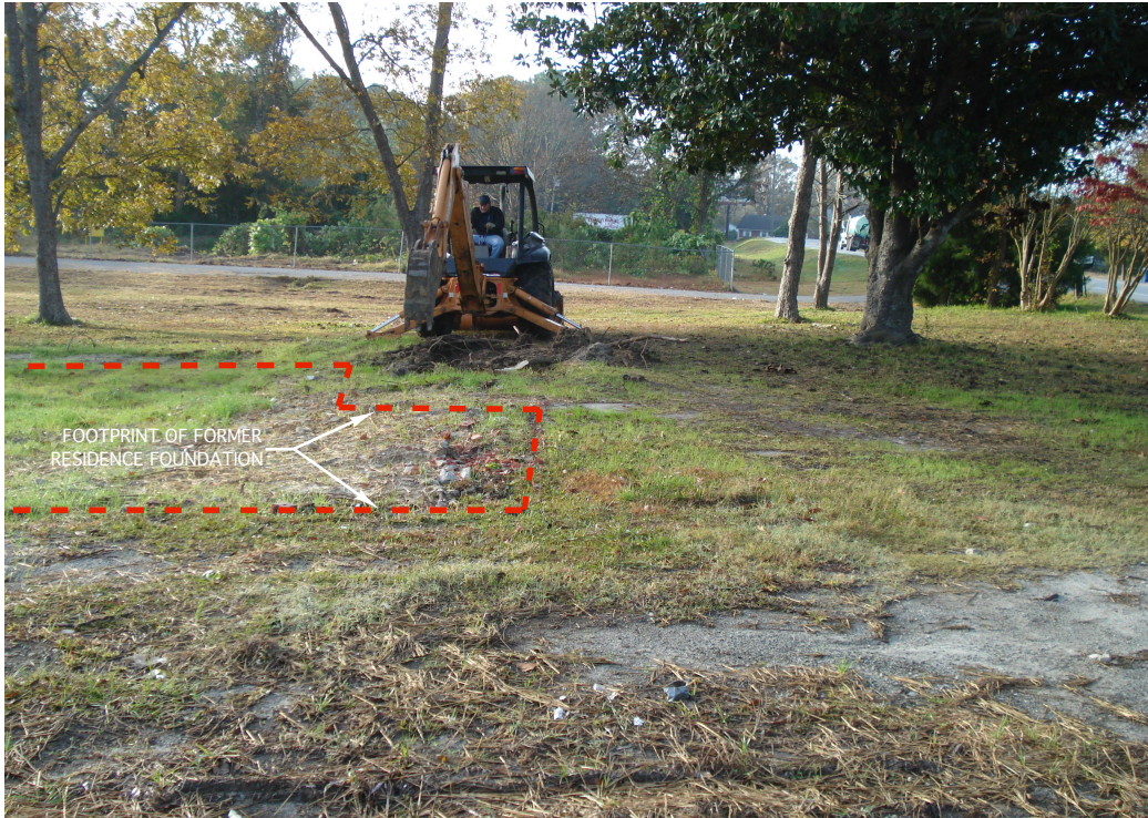
Photograph 1: View looking south at beginning of excavation activities along southwest corner of former residence.
