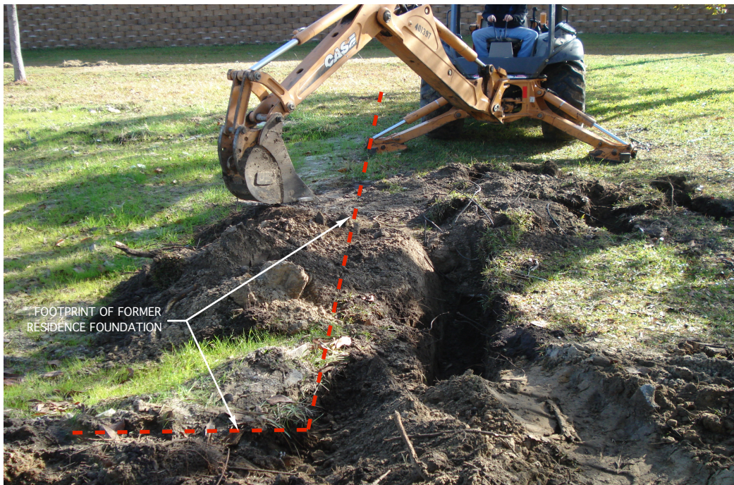
Photograph 2: View looking east at beginning of excavation activities along south side of former residence foundation.
