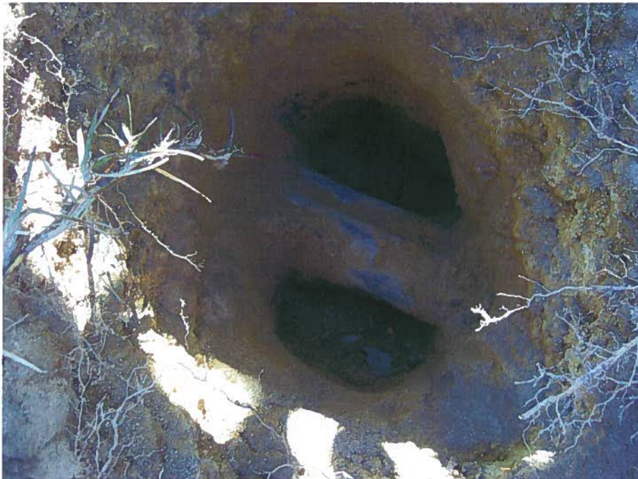
Photograph 6 – Photo of pipes coning from the UST field heading towards Legion Road.
