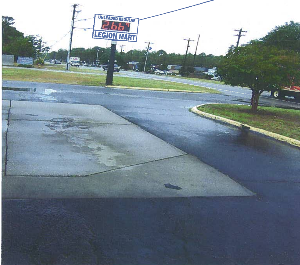
Photograph 3 – View looking south. A sample was collected from the two corners of the concrete pad.
