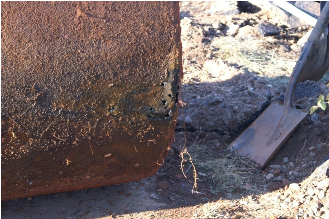
Photograph 4: View of UST corrosion, (formerly base of south end of tank).
