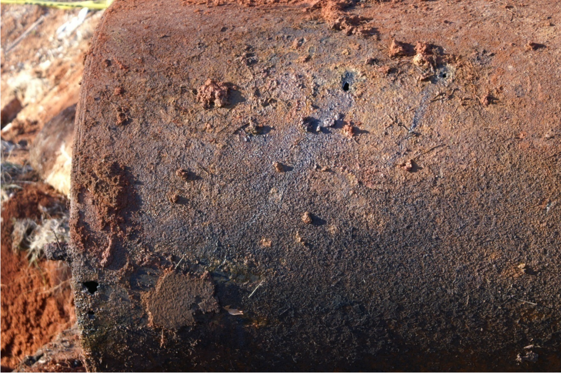
Photograph 3: View of UST corrosion, (formerly base of north end of tank).
