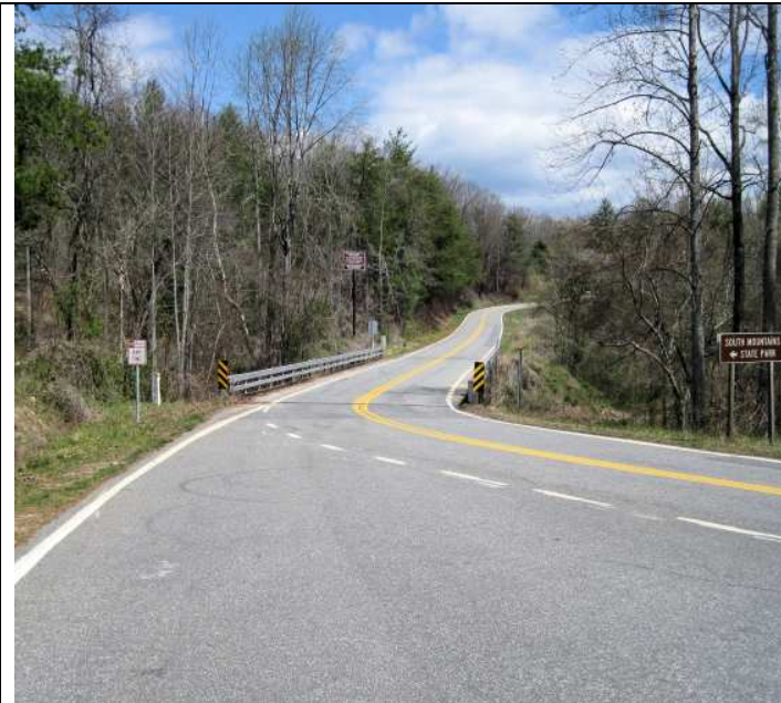
Bridge 38 over Jacob Fork River on SR 1901 (Wards Gap Road). View to the northeast.
