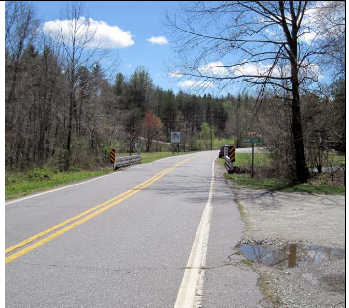
Bridge 175 over White Oak Creek on SR 1901 (Wards Gap Road). View to the south.
