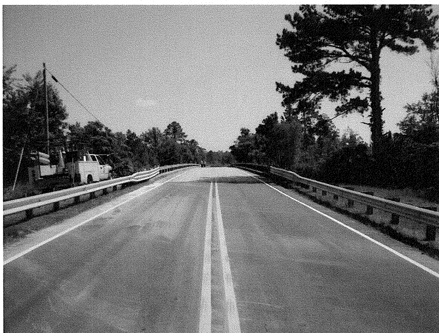
Photograph No. 1: This photograph was taken from the south approach, right of the -L- alignment, looking north.
