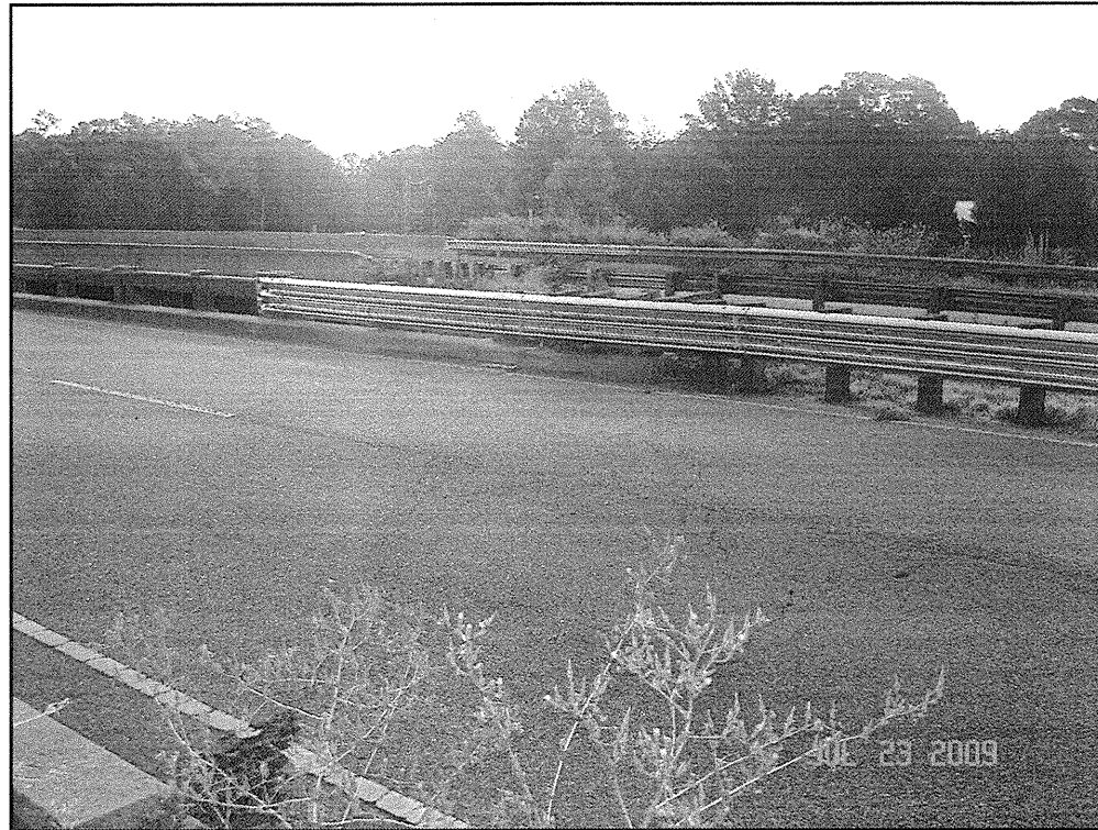
PHOTOGRAGH No. 5: Taken from the left side of the -L- alignment, looking east across proposed End Bent #1 of the replacement bridge
