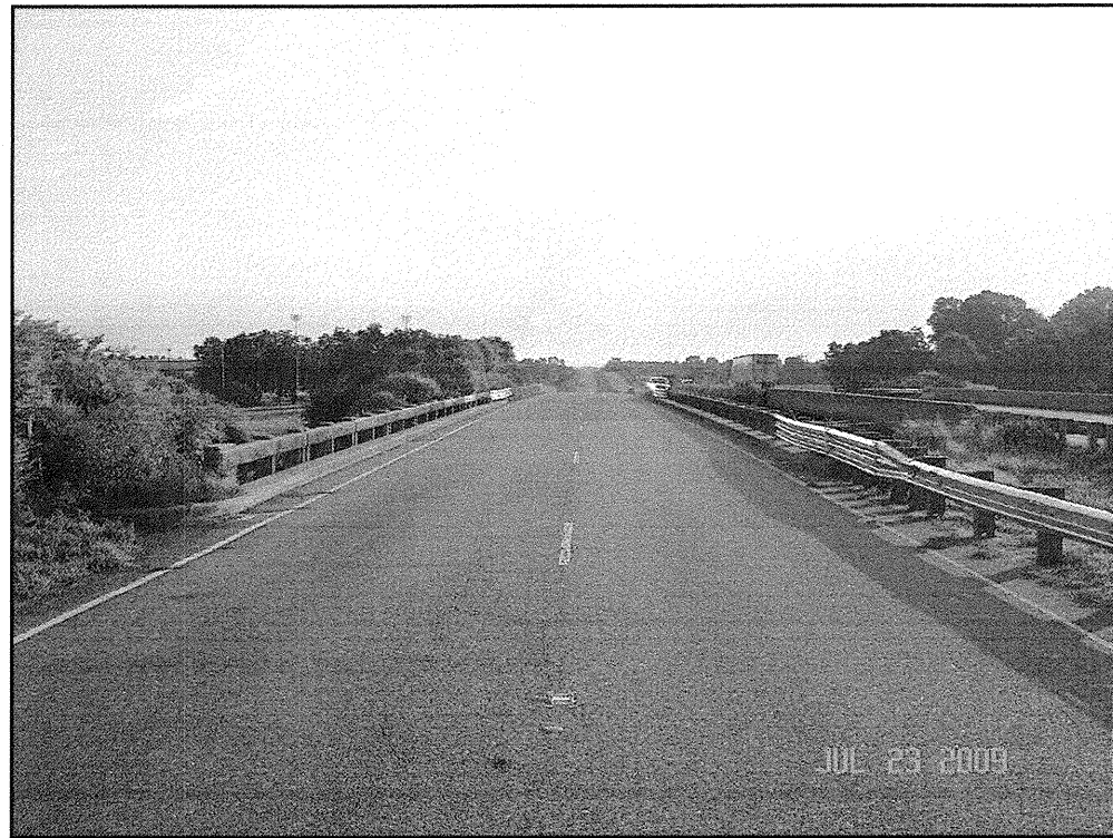
PHOTOGRAGH No. 6: Taken from the southwest approach of the replacement bridge End Bent #1, along the -L- alignment, looking northeast, at the existing bridge
