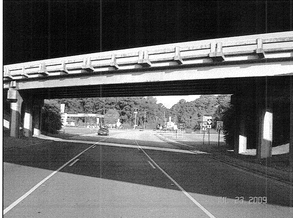
PHOTOGRAGH No. 8: Taken along the -Y- alignment, looking west, at the existing bridge
