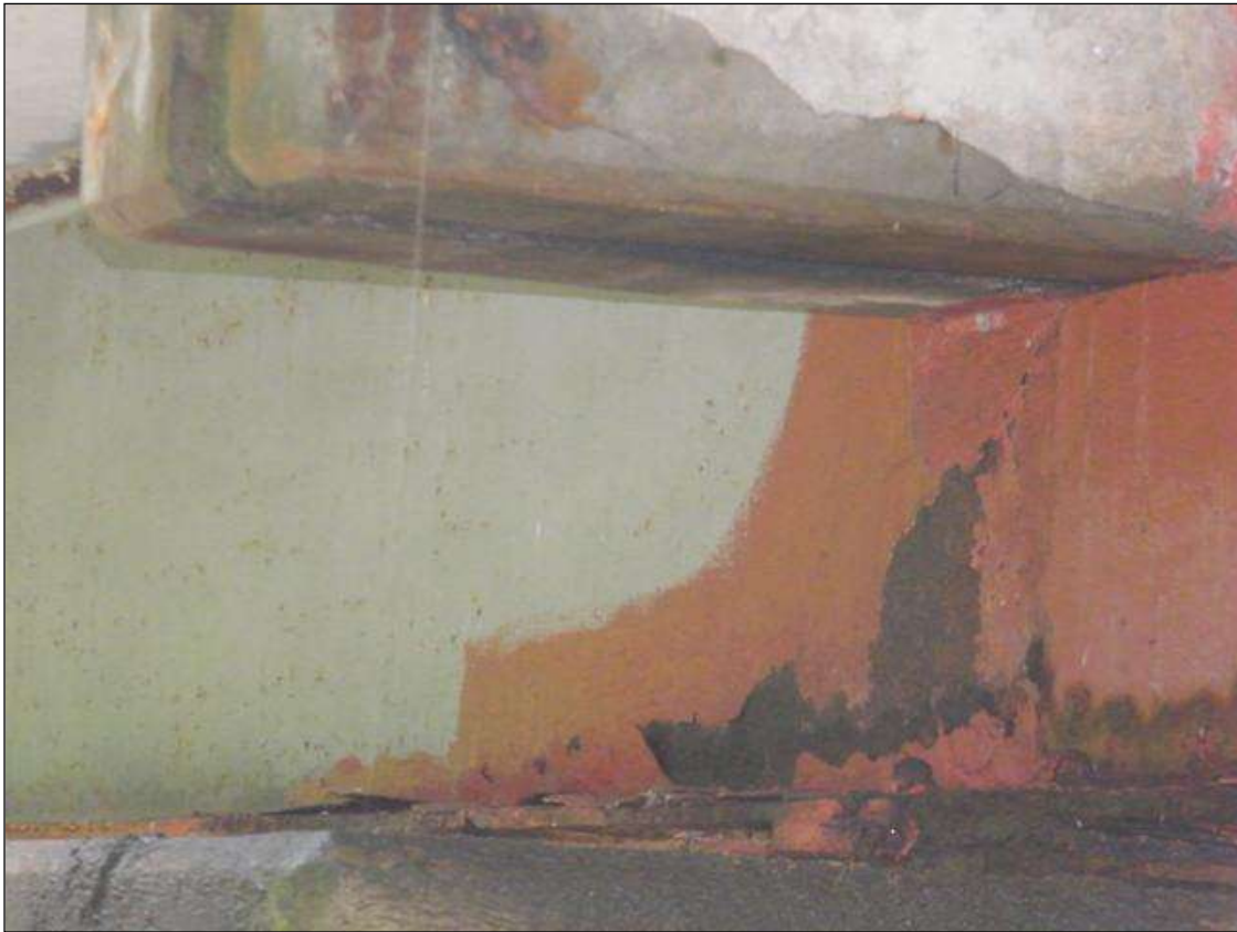
BEAM 1, SPAN 2 HAS AREAS OF PAINT PEELING WHERE SCALED AREA WAS PAINTED OVER
