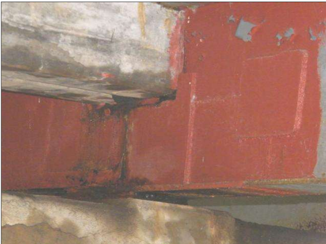
TEMP. REPAIRS, BEAM 2, SPANS 1,2 HAS BEEN PLATED ALONG THE WEB AT PIER 1
