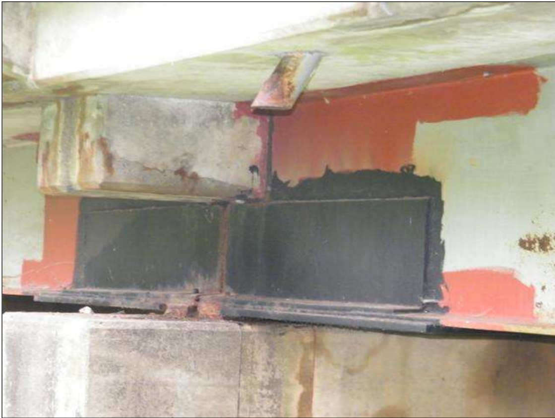
TEMP. REPAIRS, BEAM 4 IN SPANS 2,3 IS PLATED ALONG THE WEB AND BOTTOM AT PIER 2
