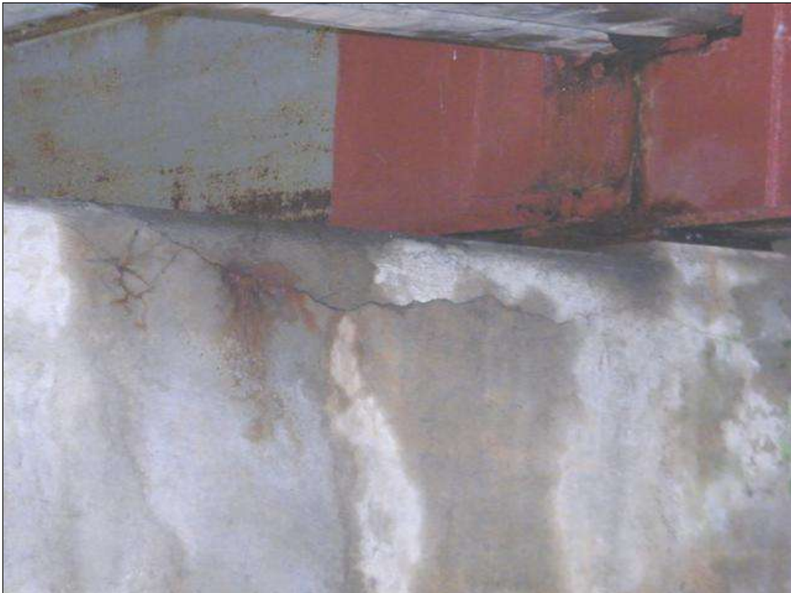
PIER 1 CAP HAS H/L HORIZONTAL CRACKING BETWEEN PILES 2 THRU 4
