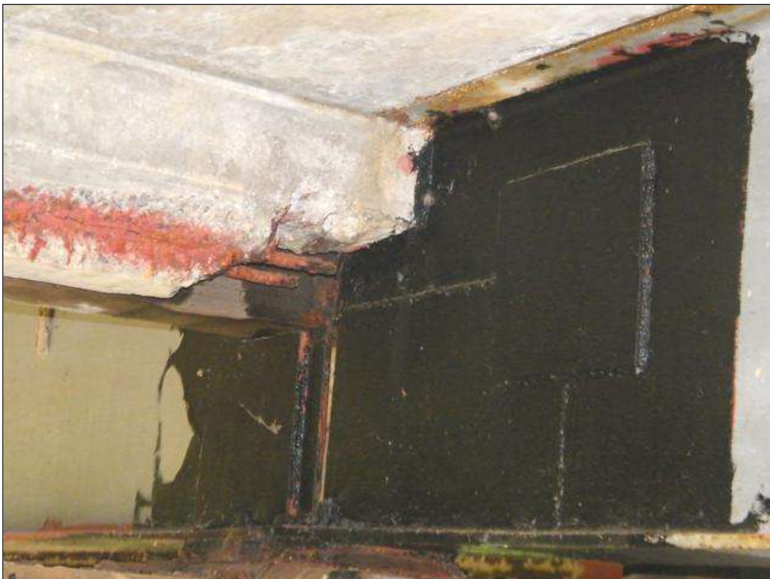
TEMP. REPAIRS, BEAM 3 IN SPANS 2,3 IS PLATED ALONG THE WEB AT PIER 2
