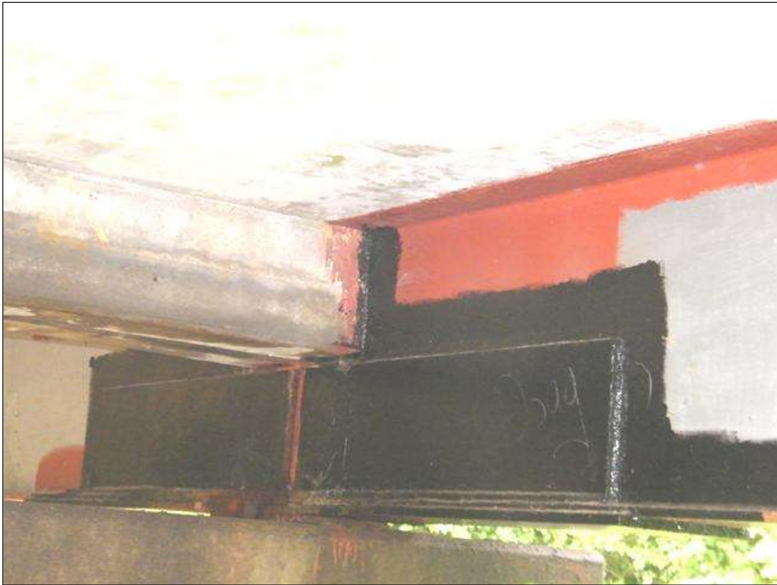
TEMP. REPAIRS, BEAM 1 IN SPANS 2,3 IS PLATED ALONG THE WEB AND BOTTOM AT PIER 2
