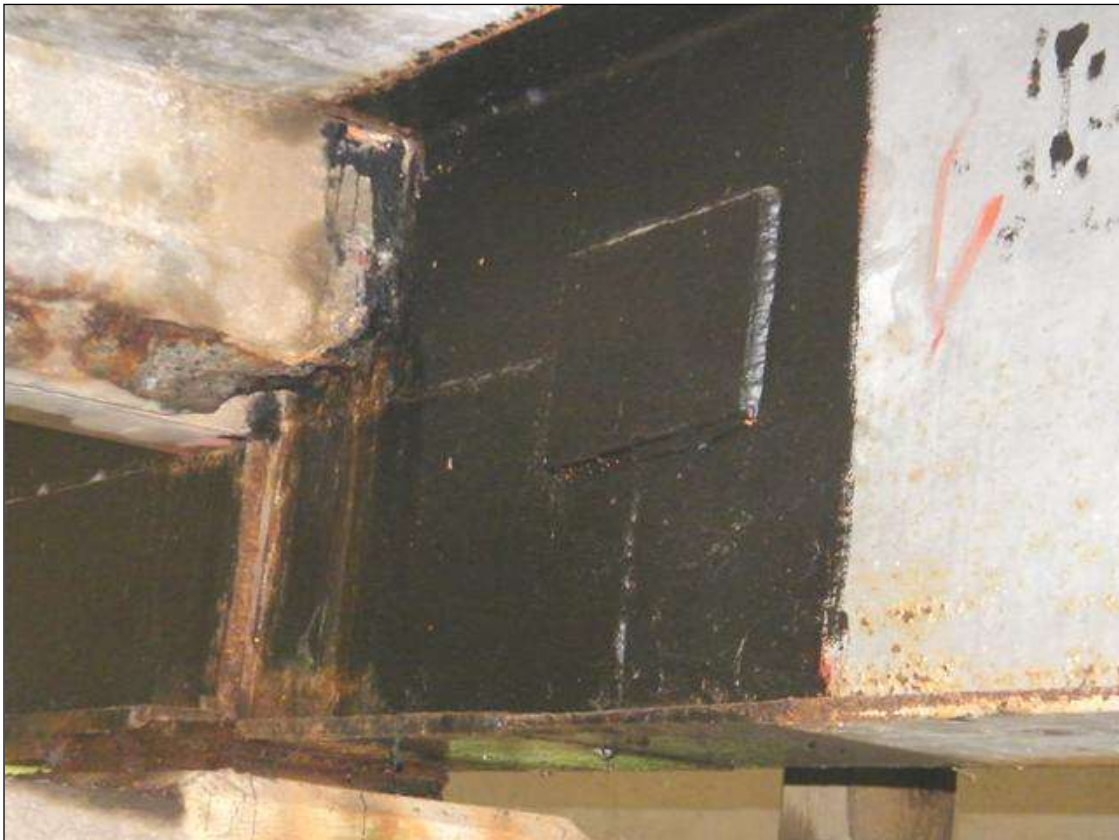
TEMP. REPAIR, BEAM 2, SPAN 3 @ PIER 2 HAS BEEN PLATED ALONG THE WEB
