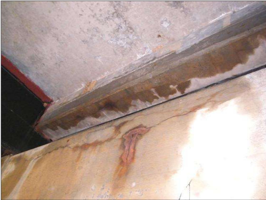
PIER 2 CAP HAS A HORIZ. H/L CRACK ON THE SOUTH FACE AT BAY 2
