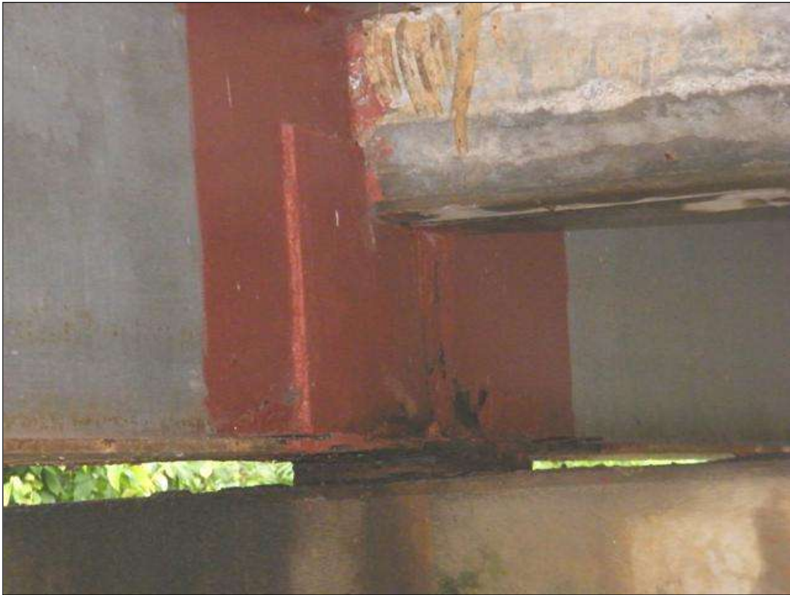
TEMP. REPAIR, BEAM 1, SPAN 1 HAS BEEN PLATED ALONG THE WEB AT PIER 1
