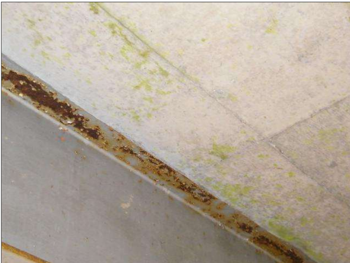
BEAM 3, SPAN 2 HAS SURFACE RUST IN SPOTS ALONG LENGTH
