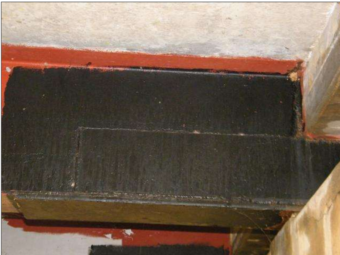
TEMP. REPAIR, BEAM 2, SPAN 2 HAS BEEN PLATED ALONG THE WEB AT PIER 2
