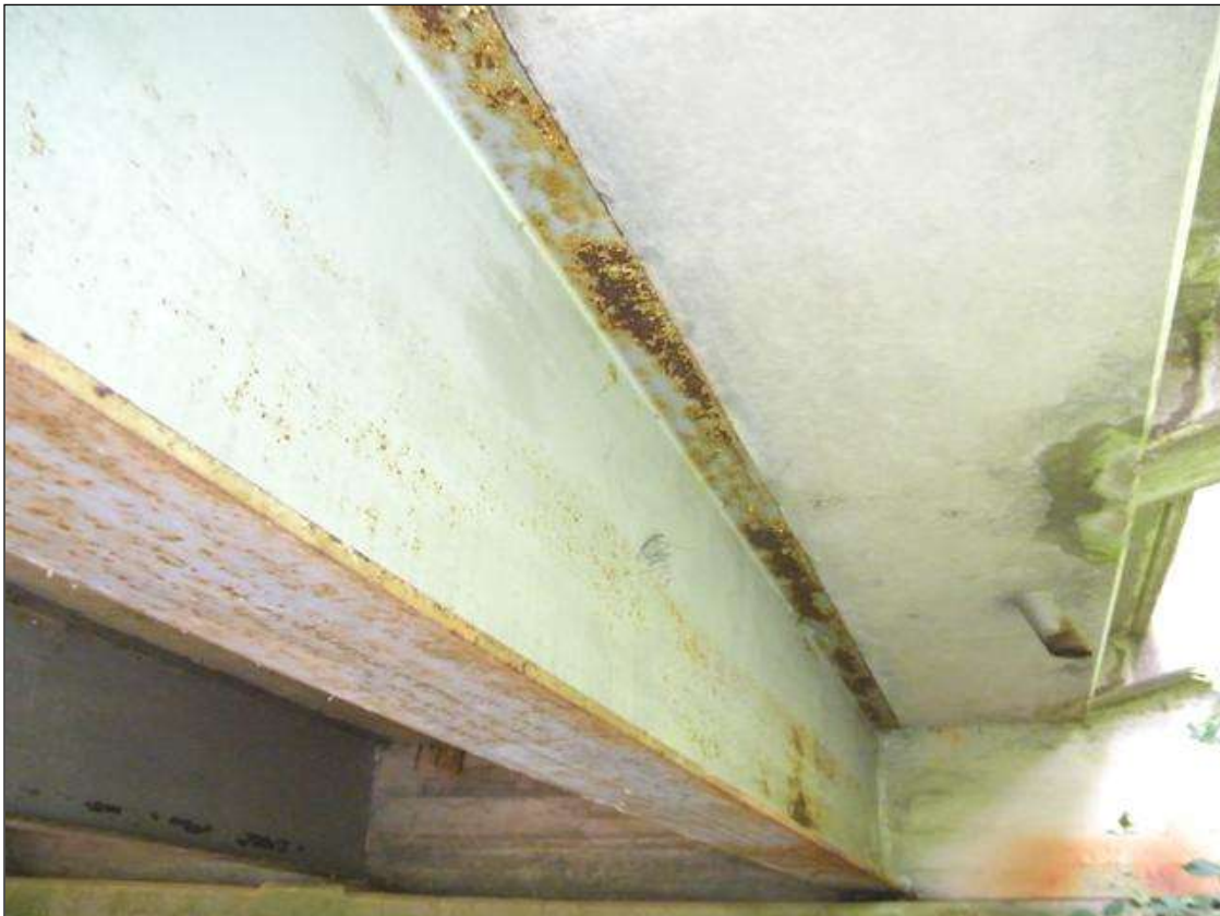
BEAM 1, SPAN 1 HAS SURFACE RUST ALONG LENGTH
