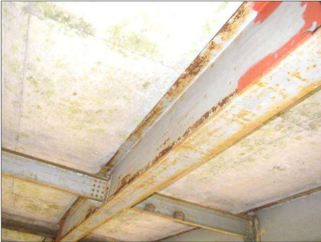
BEAM 2, SPAN 2 HAS SURFACE RUST IN SPOTS ALONG LENGTH
