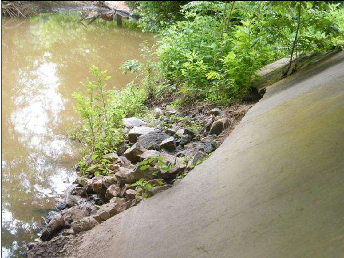
SOUTH SLOPE PROTECTION HAS SECTION MISSING ON RIGHT SIDE AND BOTTOM , RIP-RAP HAS BEEN ADDED AT MISSING SECT .
