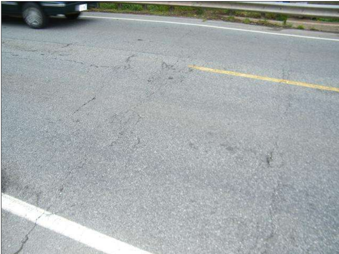
SOUTH APPROACH ROADWAY IS CRACKED
