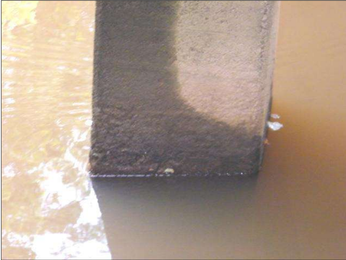
PILE ENCASEMENTS HAVE UP TO 1" DEEP SURFACE PITTING ALONG THE W/L
