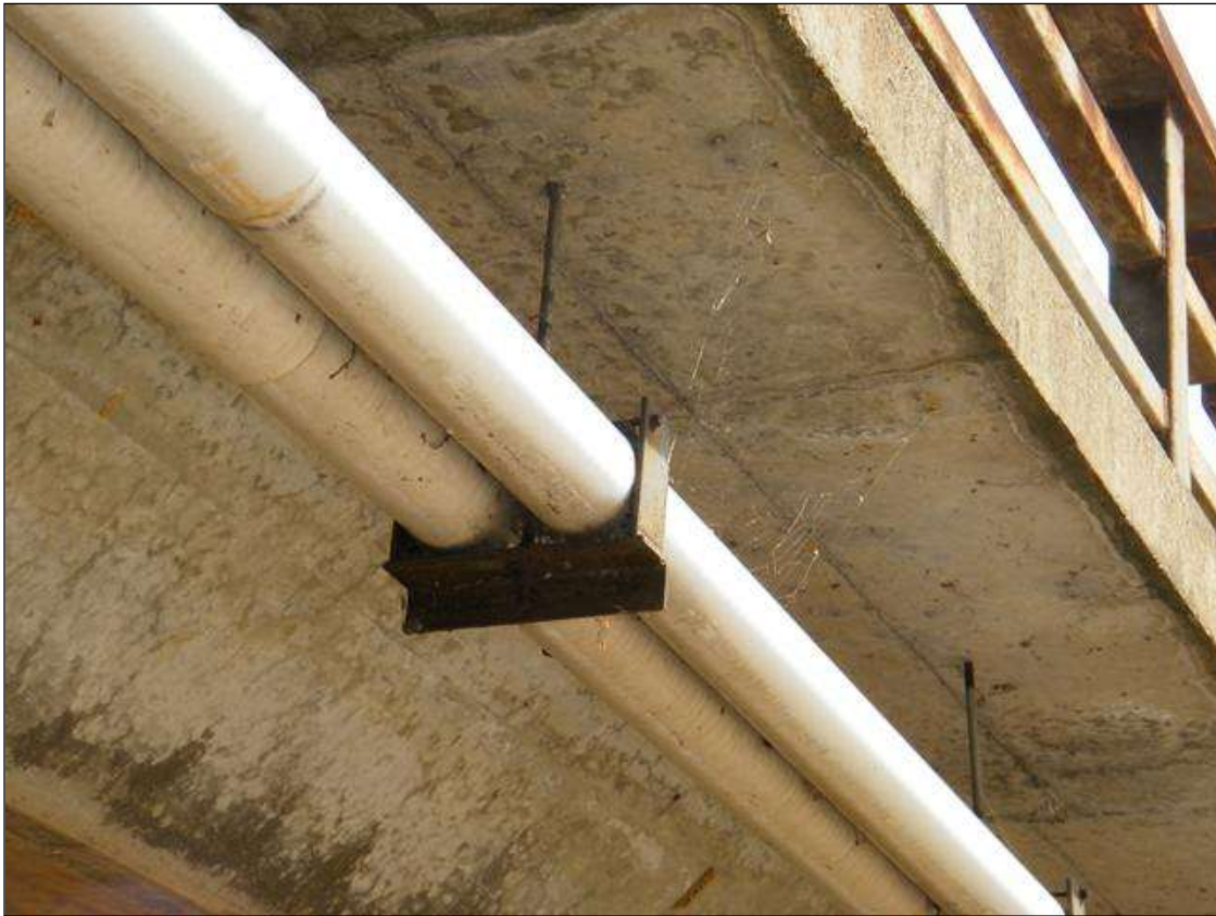
UTILITY AND HANGER UNDER LEFT OVERHANG, 2 LINES OF 6" DIAM. PVC
