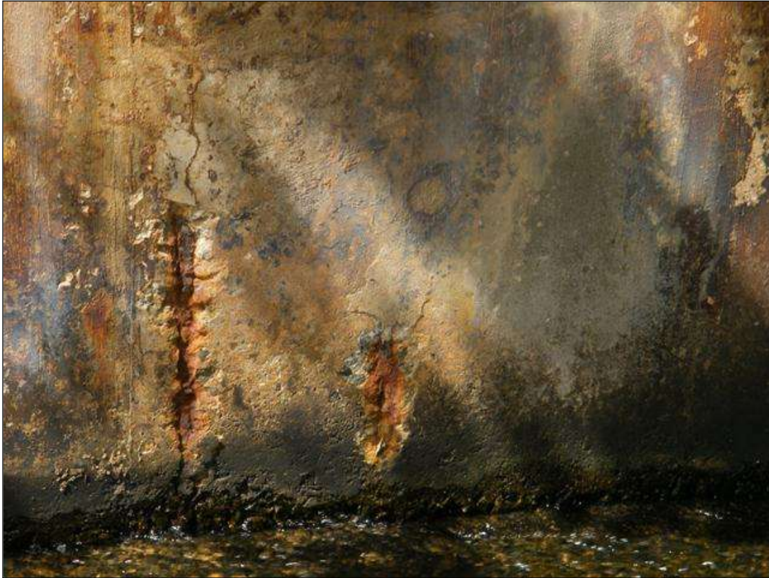
ABUTMENT 2 HAS 2- 1" DEEP SURFACE SPALLS WITH REBAR EXPOSED
