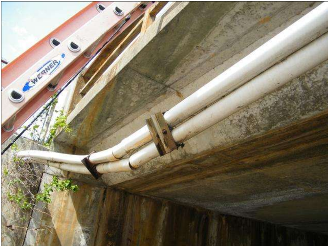
UTILITY HAS BRACKETS BROKEN IN 2 AREAS .
