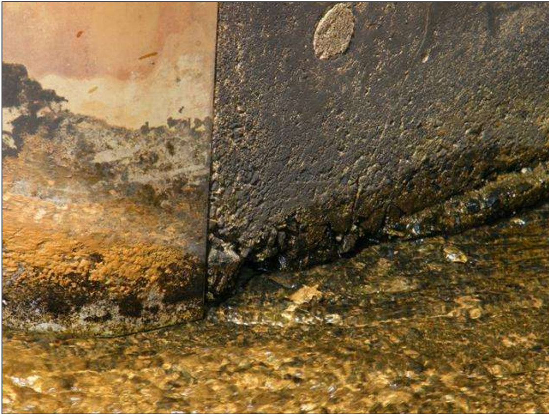
PIER 4 IS PITTING AT W/L 2 INCHES DEEP AT UPSTREAM END IB 6 INCH AREA .
