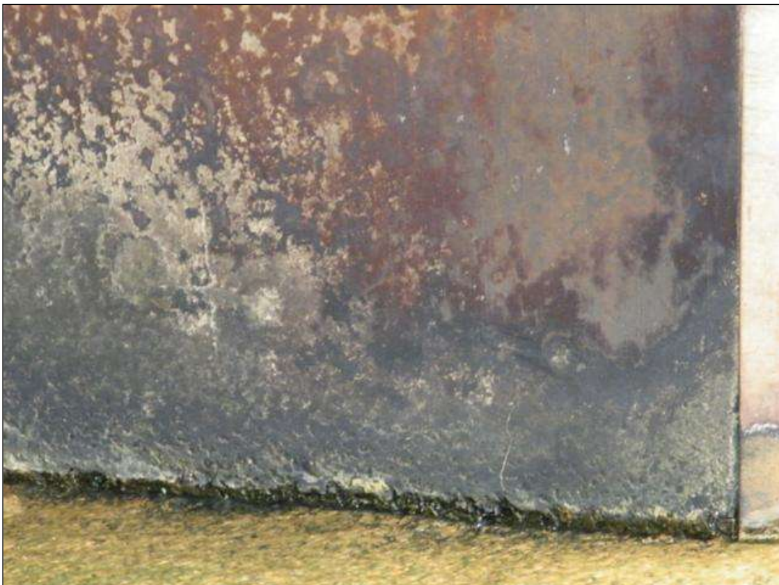
PIER 3 COLUMN IS PITTING UP TO 1" DEEP AT WATERLINE
