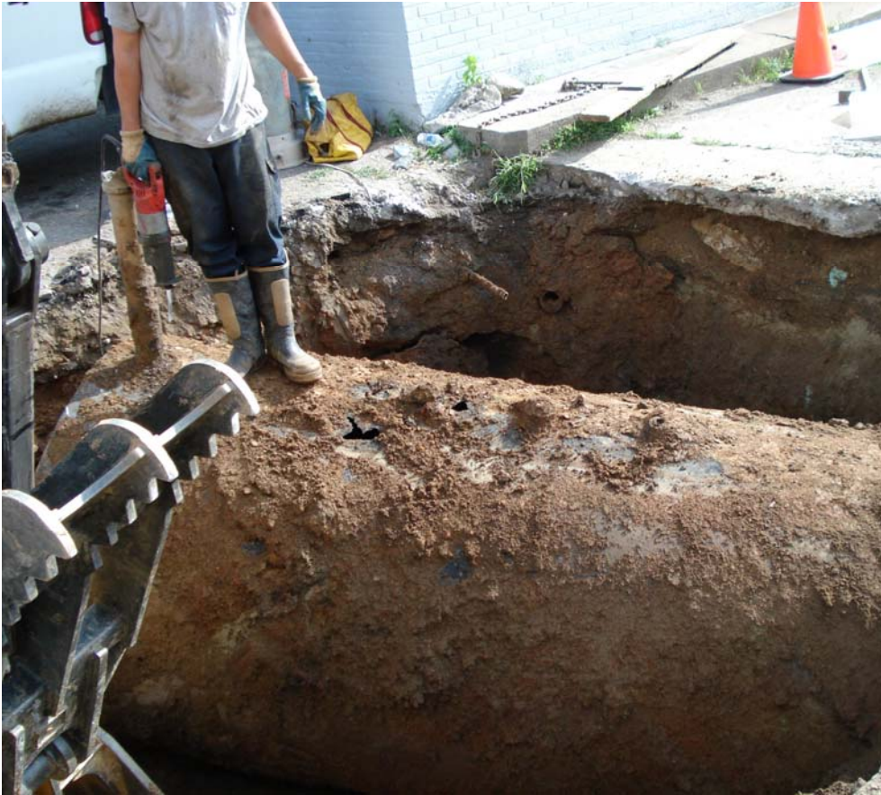
Photograph 3: View looking southwest at removal of UST #002. Holes shown on top of tank were created by UST removal contractor.
