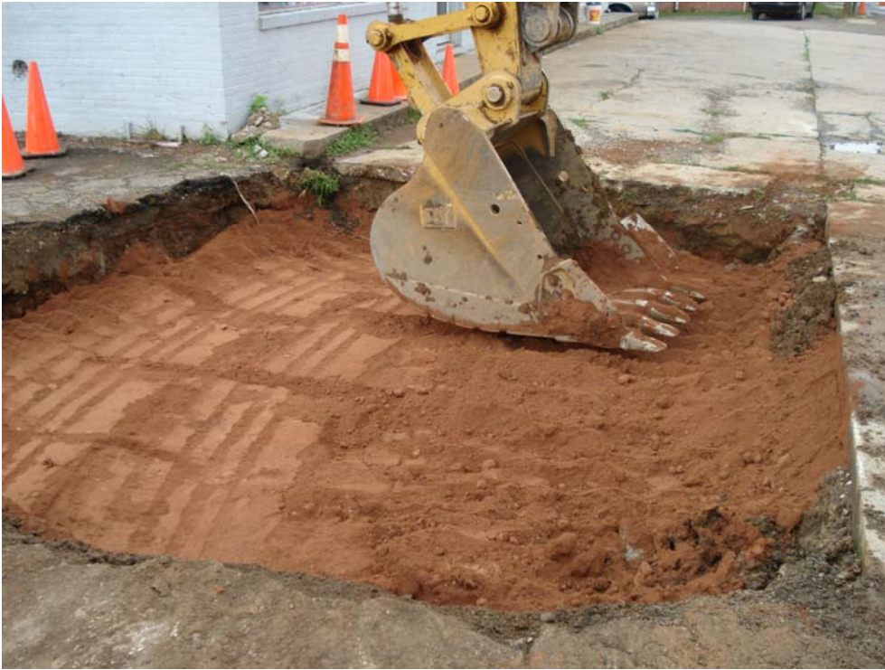
Photograph 5: View looking southwest at compaction of fill material that had been backfilled into UST excavation.
