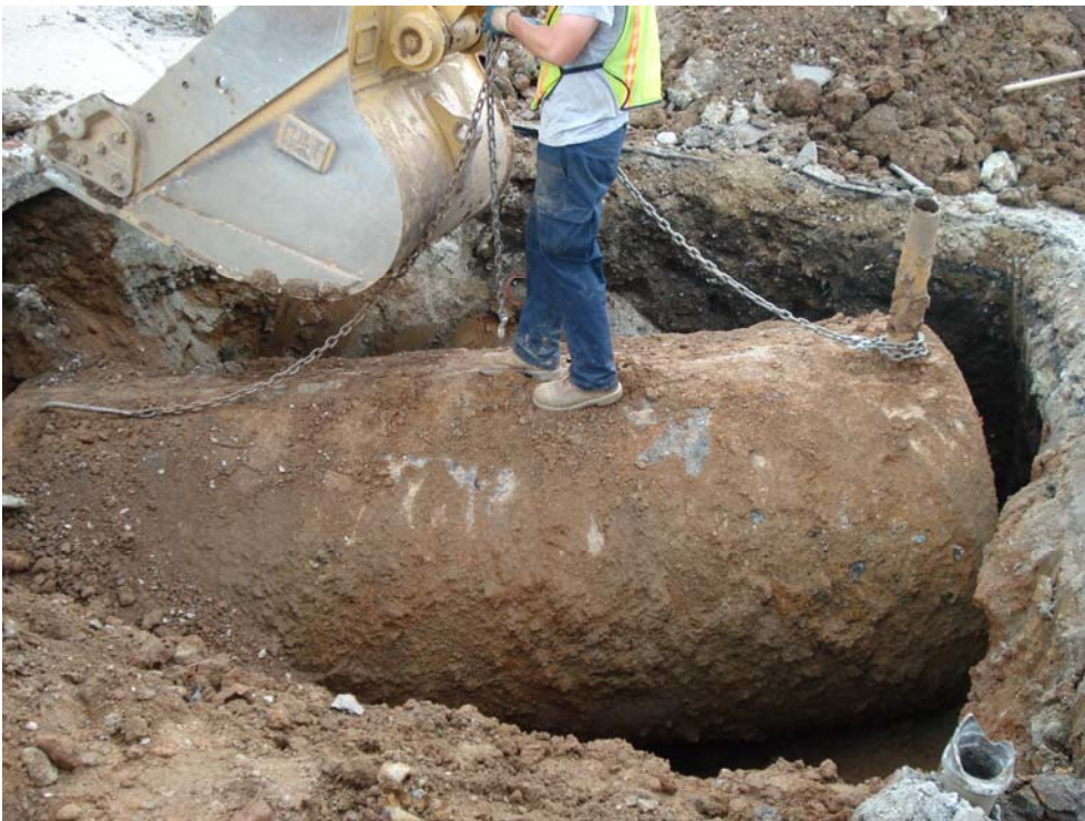
Photograph 2: View looking east at removal of UST #001. UST fill pipe for UST #002 is shown in lower right corner of photo.
