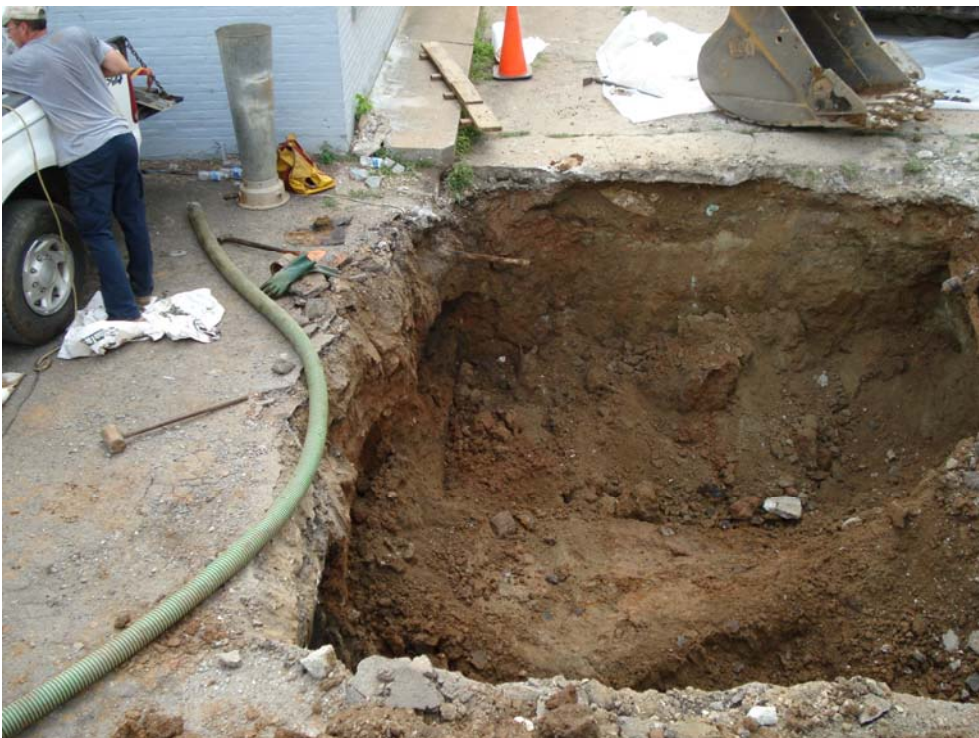
Photograph 4: View looking west at UST pit following removal of UST #001 and UST #002..
