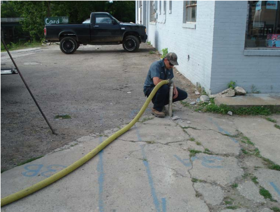
Photograph 1: View looking south at removal of residual liquid from UST #002 fill pipe prior to removal of UST #001 and UST #002
