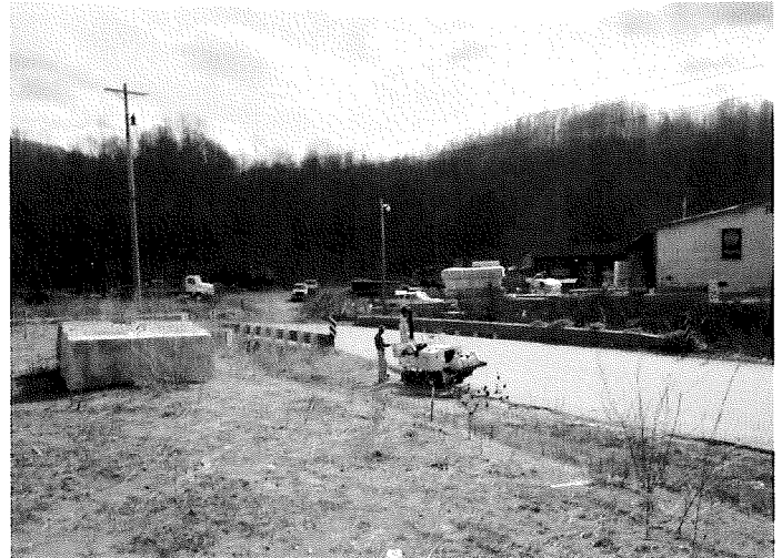
Photograph 4: Looking southwest at (GP-1) boring location along the proposed drainage piping location.
